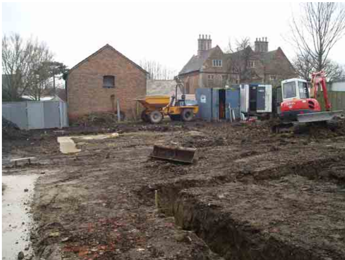
Plate 3: View south across garage area (following concreting of trenches) from between both house plots.
