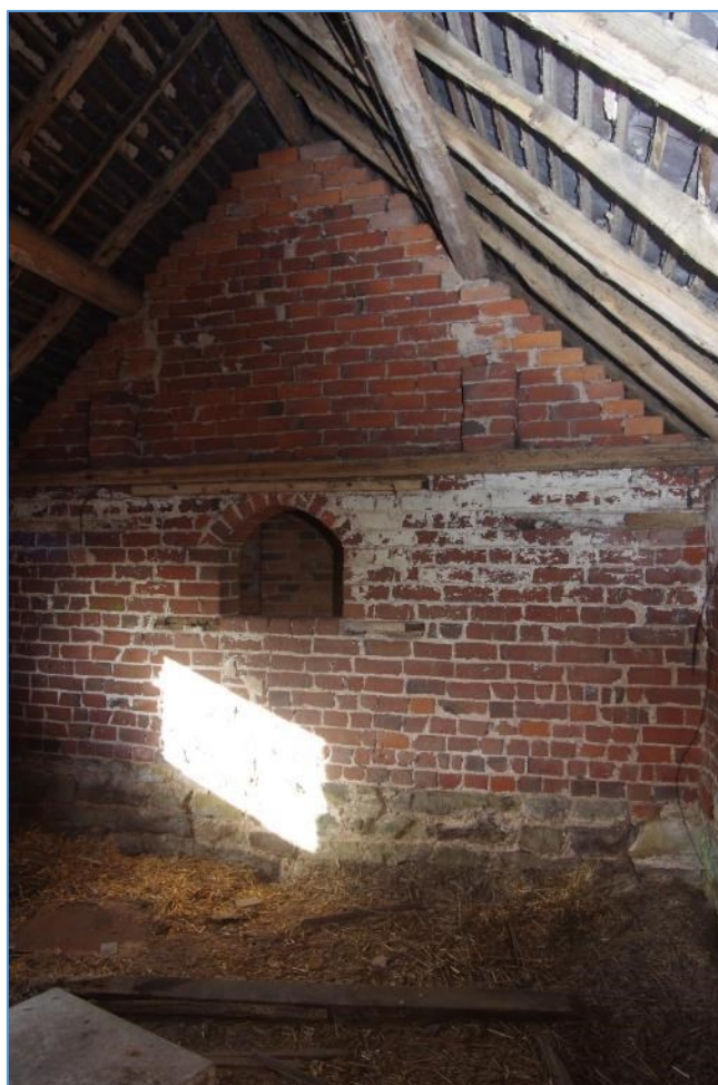
Figure 18 Block B South unit looking north towards original gable end. Note heightened gable and small brick pillars which would have supported the purlins of the original roofline
