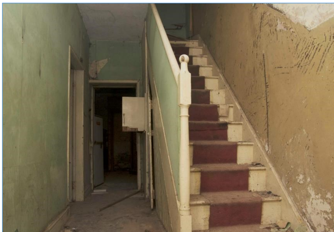
Figure 48 Servants stair. Looking north towards scullery. Small open door shows position of serving hatch
