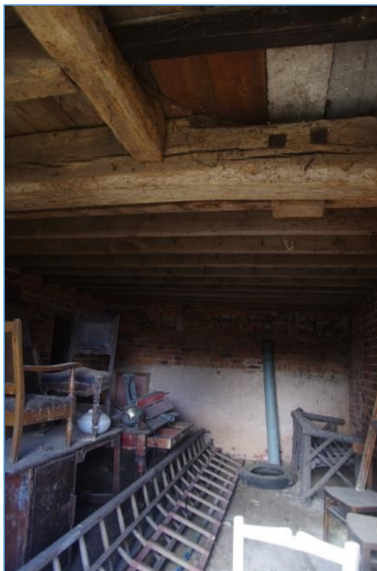
Figure 12 Block A, looking north. Small area of earlier carpentry visible in ceiling
