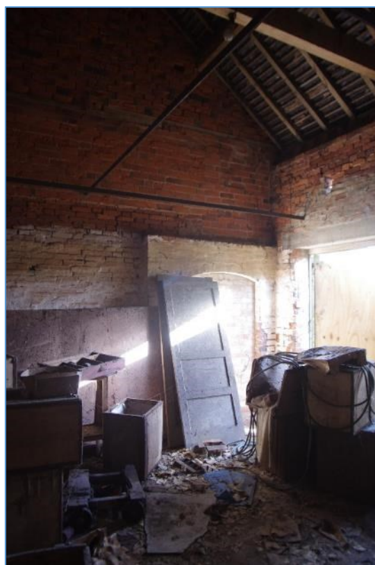
Figure 13 Block A east end, showing blocked door in gable end. Looking south-east
