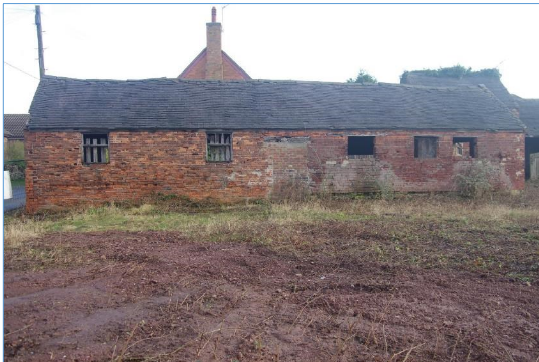
Figure 15 Block B. North unit to left. The blocked central opening indicates the original gap between the two units
