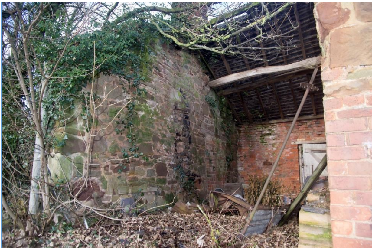
Figure 34 Block F, west end, looking north-west. Note purlin, and possible course of flue
