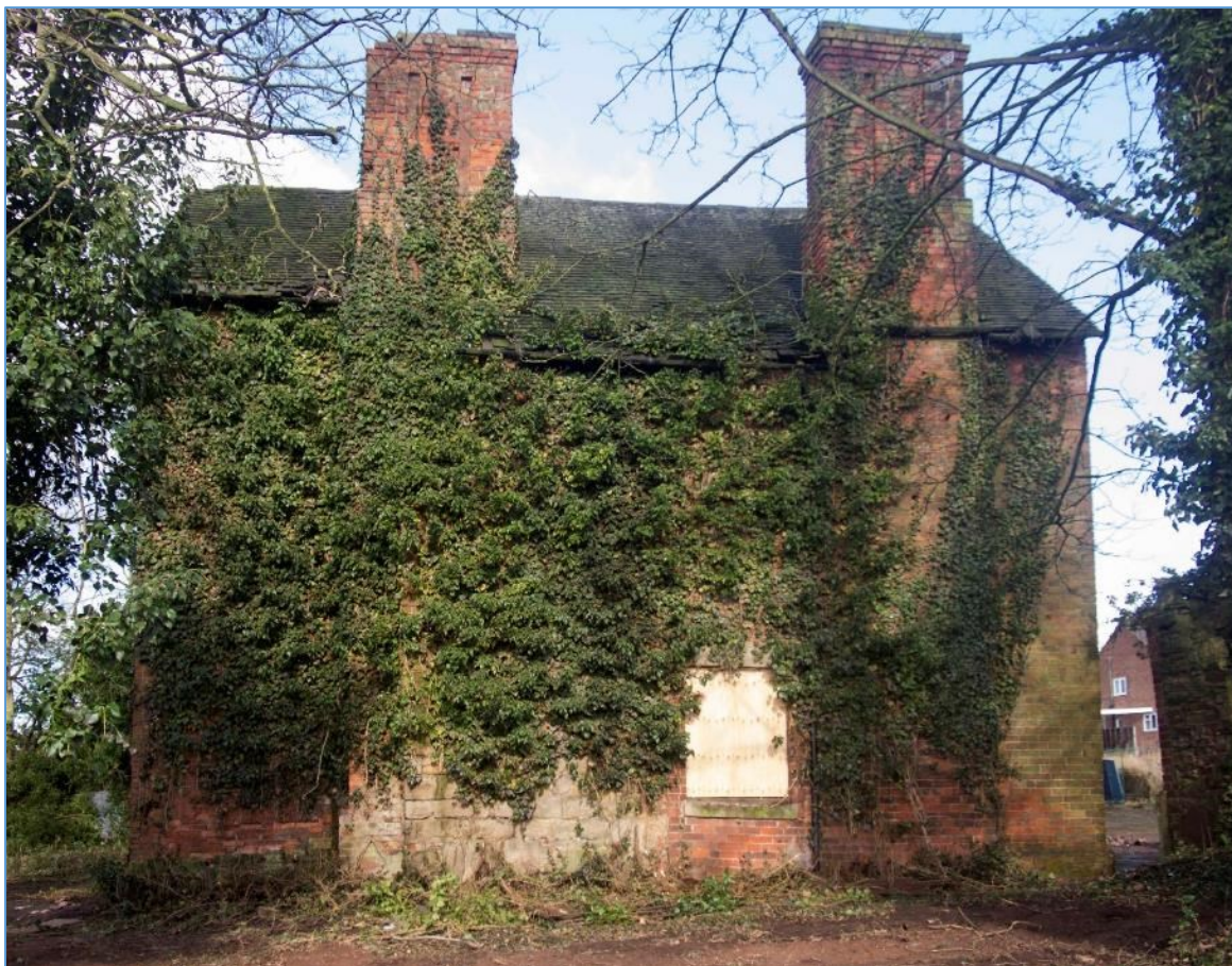
Figure 41 South elevation showing masonry stack base and earlier brickwork to left. Looking north
