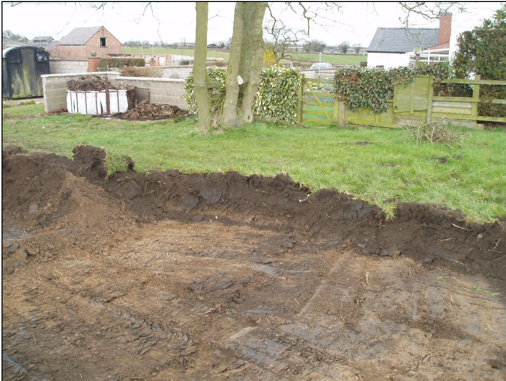
Plate 3. Step in topsoil along length of access road. Viewed from south.
