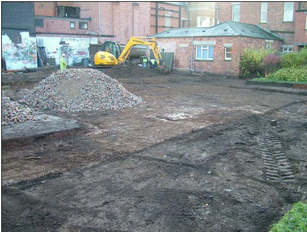
Plate 2. Site viewed from northwest. Topsoil partially removed. Location of demolished outbuildings shown by whitewash on theatre walls.
