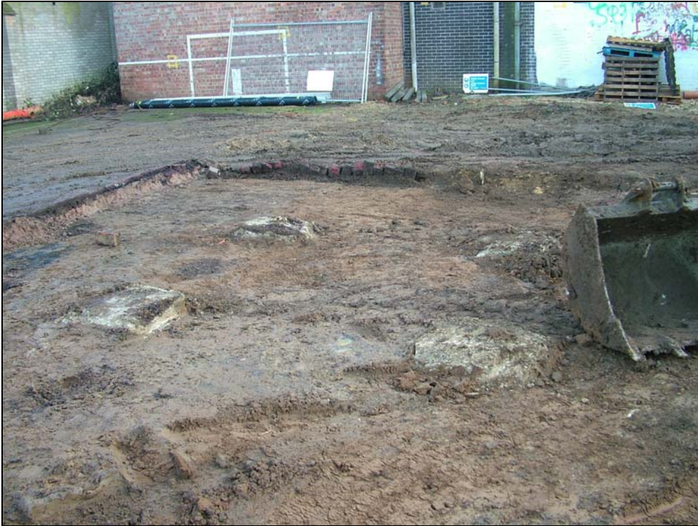
Plate 3. Truncated concrete posts and associated disturbance. Some tarmac surface still to be removed.
