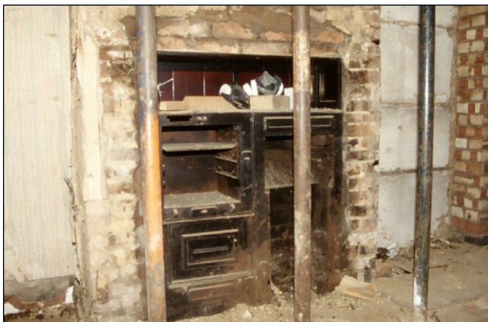
Plate 6. Remains of the ground floor range in the back room of No. 20
