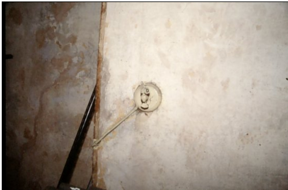
Plate 10. Gaslight fitting in No.20.
