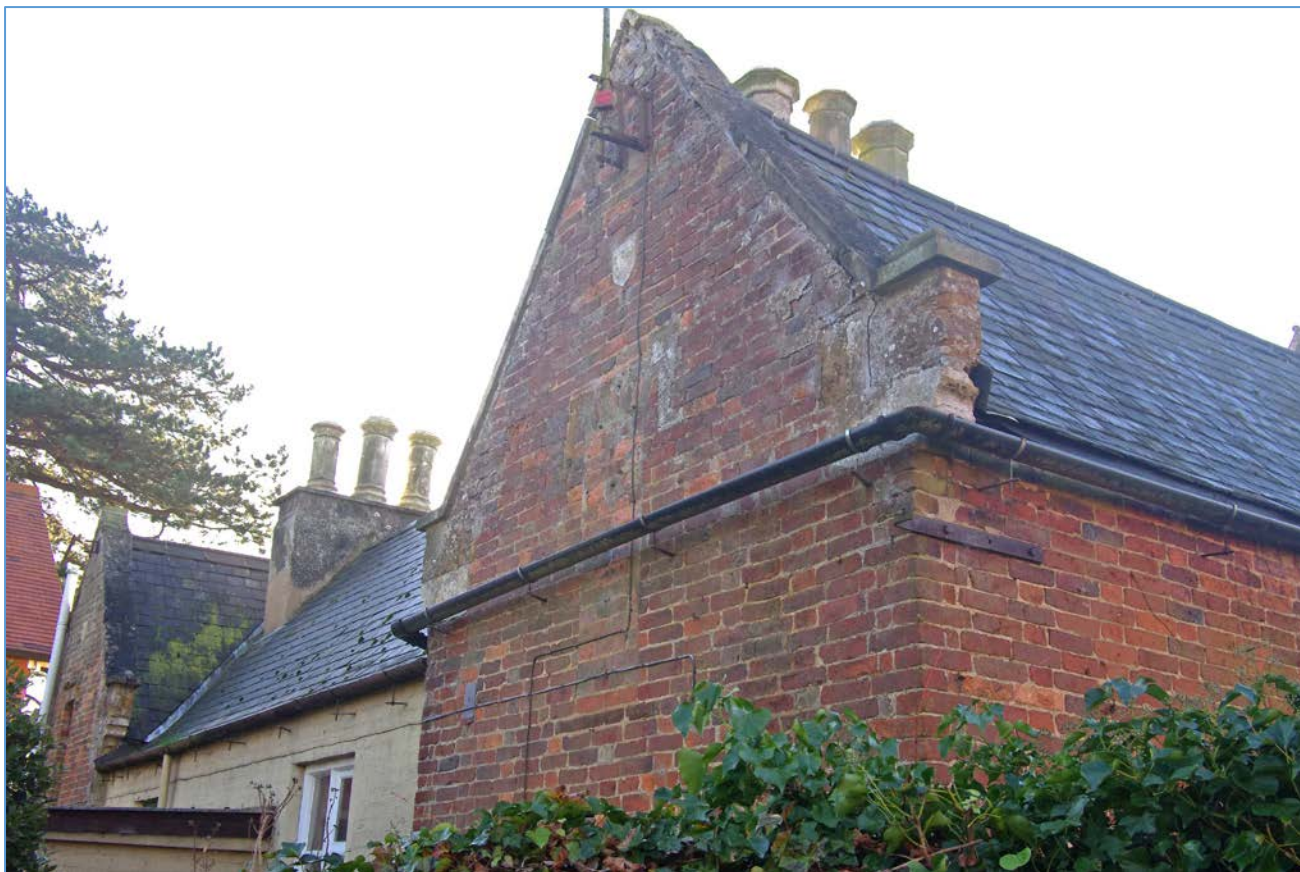
Figure 10 Rear, looking south, showing blocked window and removed hoodmould in nearest gable
