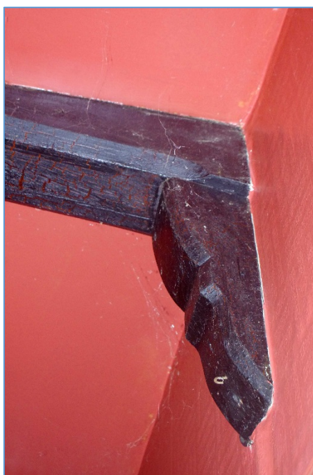
Figure 18 Chamfered and stopped foot of truss tie beam in rear wall
