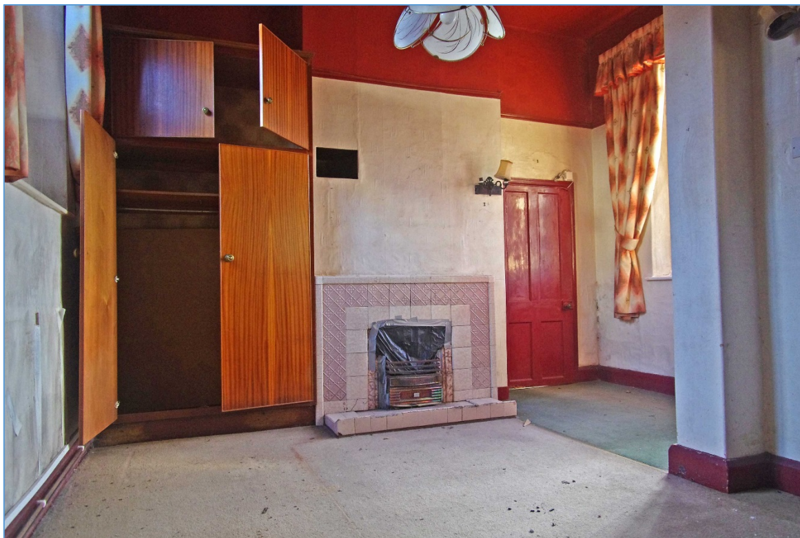
Figure 17 Central room, looking to south-east. Corridor wall to right. Note cut-down panel door into accommodation wing
