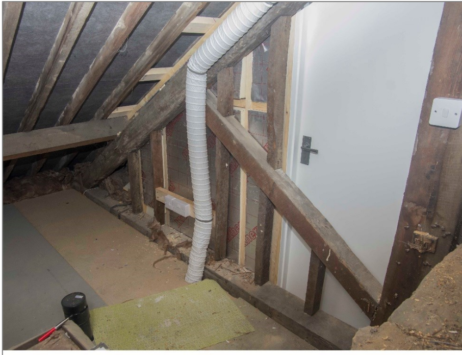
Figure 38 North roof truss, east side. Queen strut to the right with light switch
