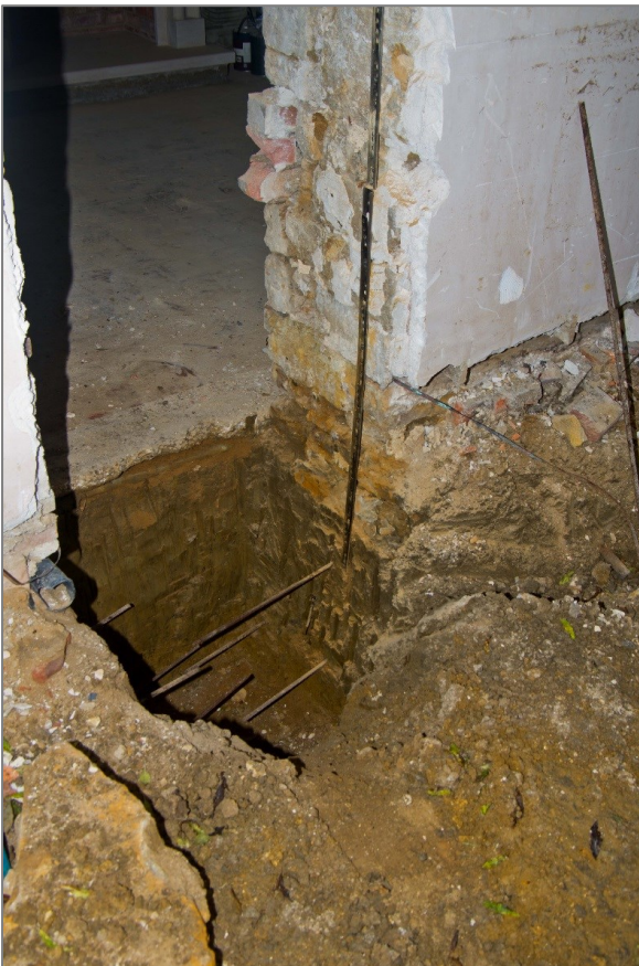
Figure 46 South east corner of main house, showing wall built straight onto the clay ground. Re-enforcing bars hammered into the sections for subsequent underpinning encountered no footings.
