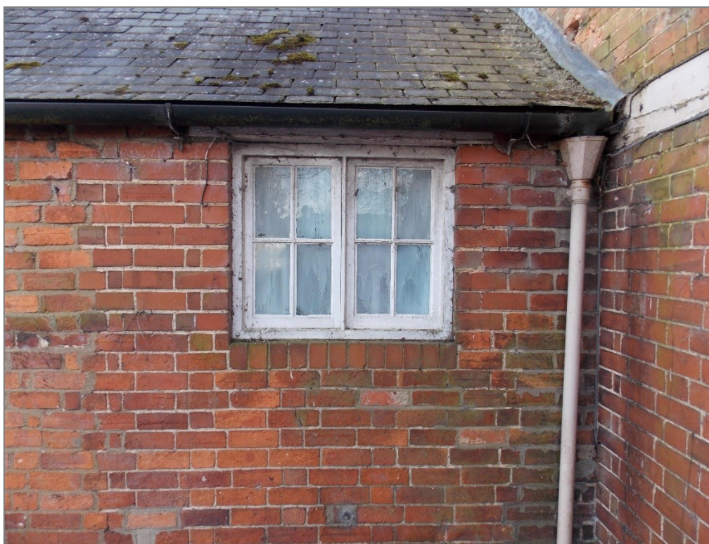
Figure 11 Junction between blocks D and E, north face. Photo provided by client
