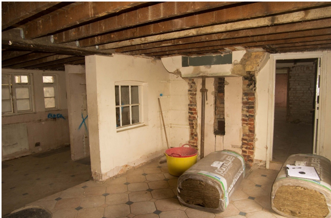
Figure 21 Block D, looking north east. Note apparent continuation of north wall of block E into interior
