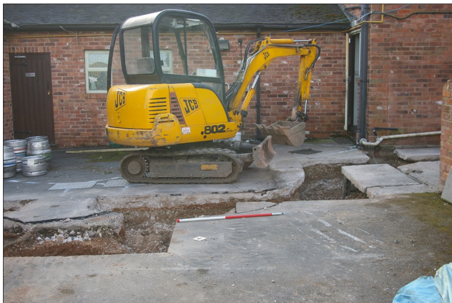
Figure 4: Area of trench prior to excavation with mini digger, concrete had been removed prior to visit by archaeologist.
