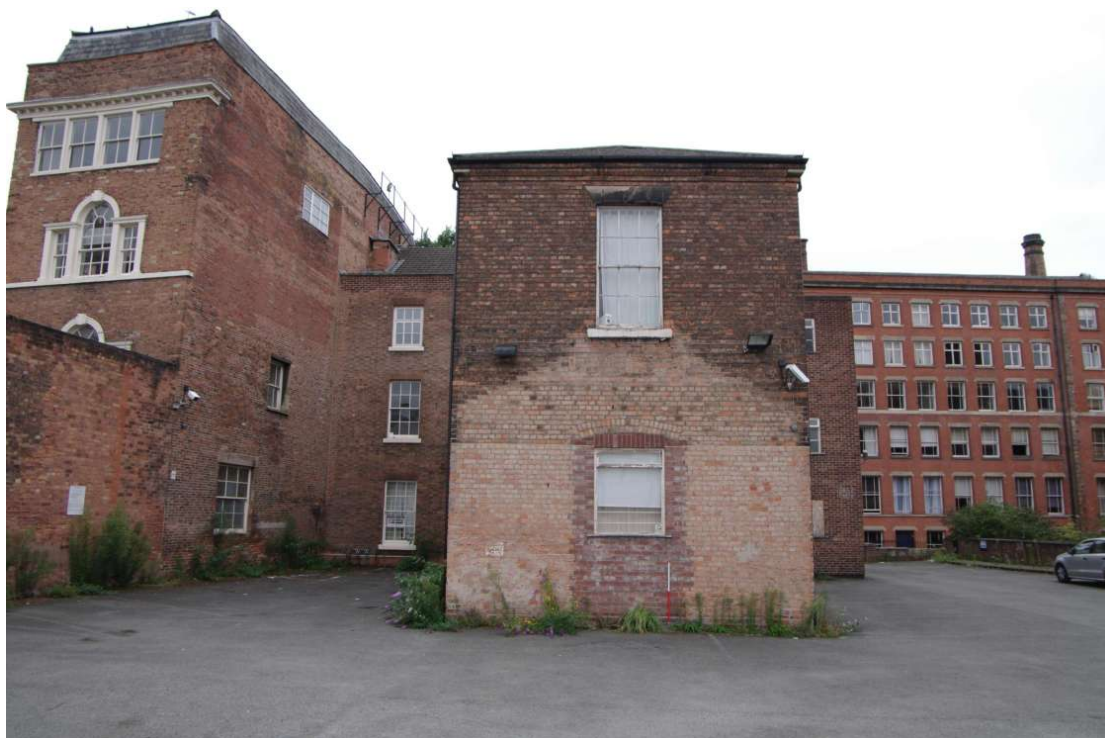
Figure 52 19th century extension, south facing elevation Looking north. Note infilled ground floor doorway. 1m scale
