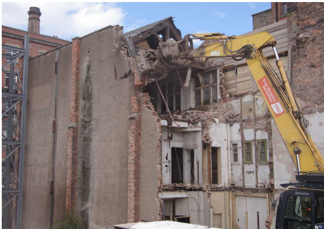
Figure 43 Front section, internal room details Looking north-east. Toilet block on right (green windows)
