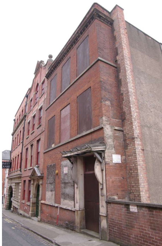
Figure 17 Number 10 Short Hill, north facing elevation Looking south-east, at Short Hill level. 1m scale
