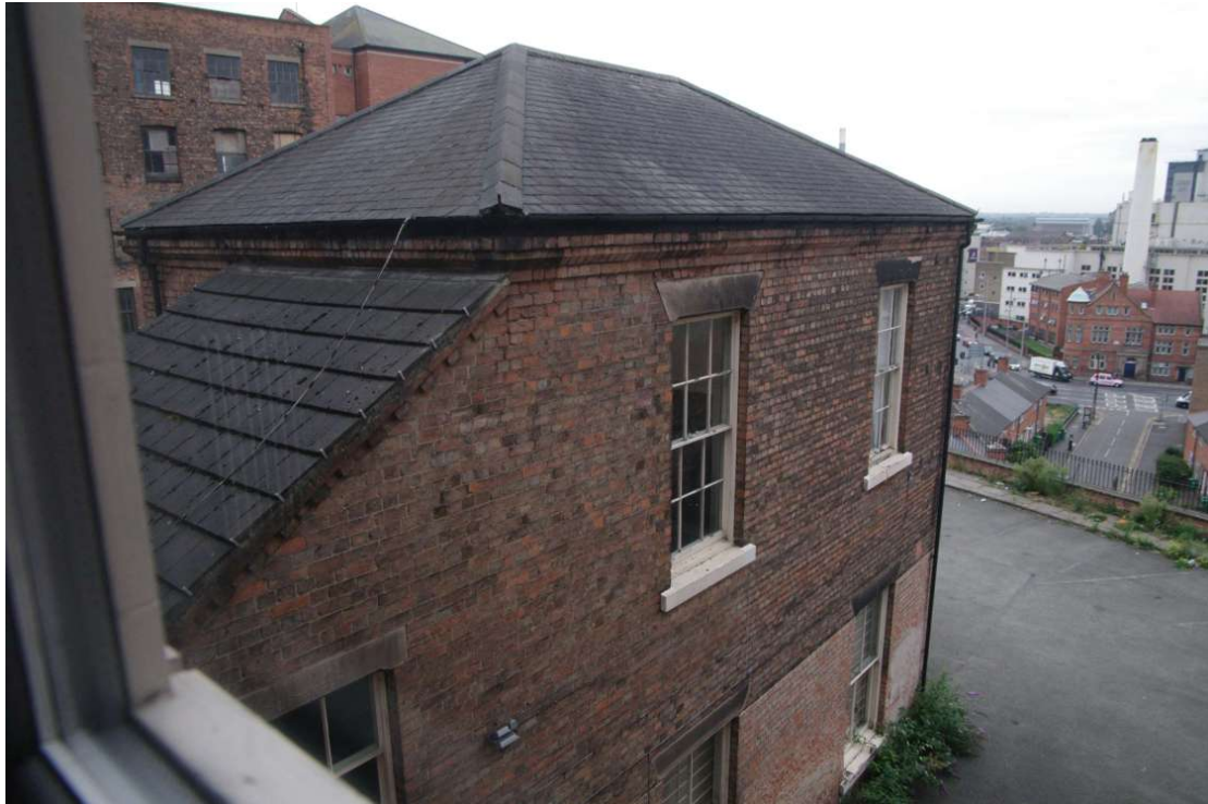
Figure 54 19th century extension, west facing elevation and roof Looking south-east from first floor of Number 56
