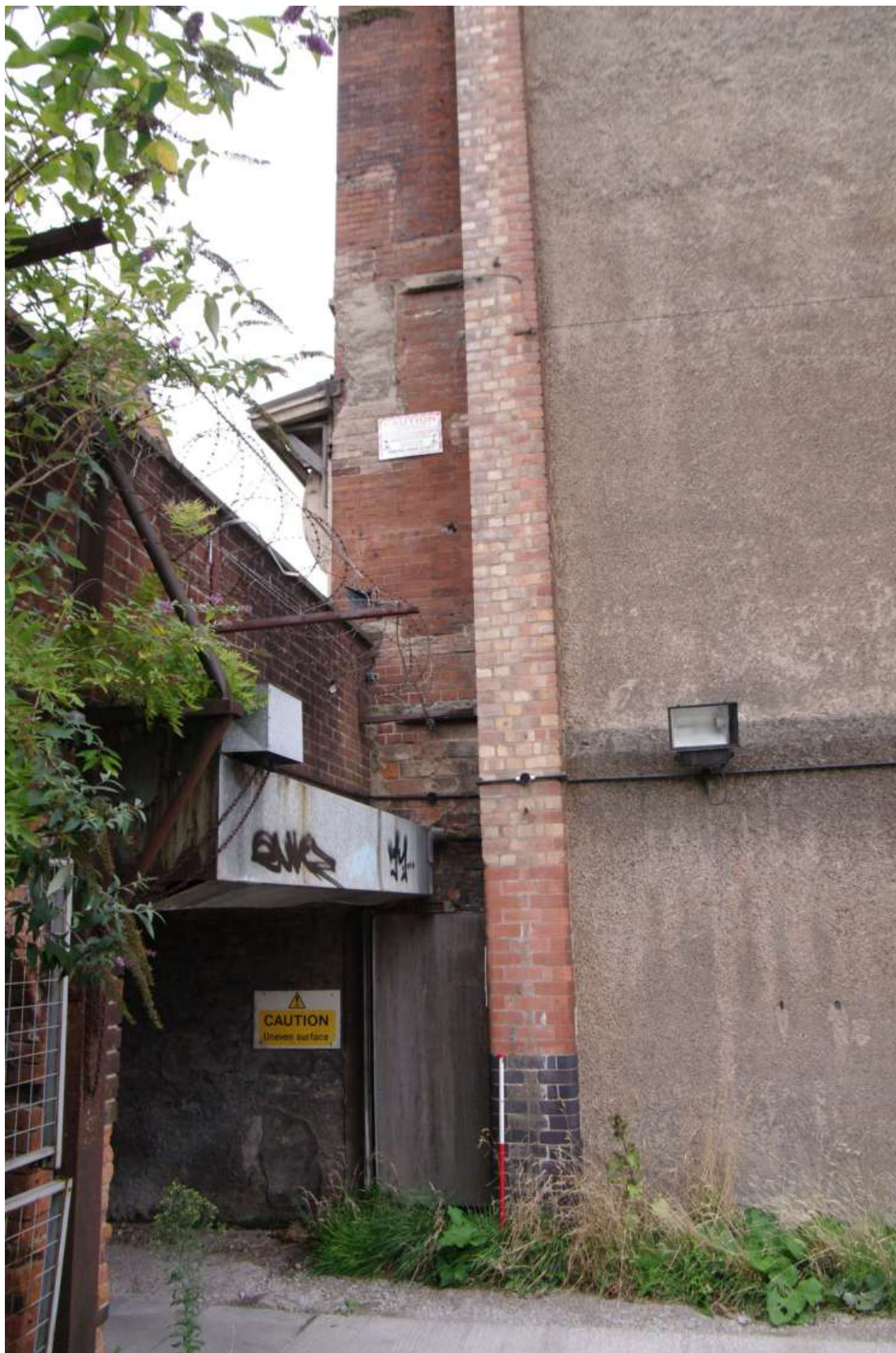
Figure 24 Number 10 Short Hill, west facing elevation. Doorway in north corner Door is behind plywood sheet. Looking north. 1m scale
