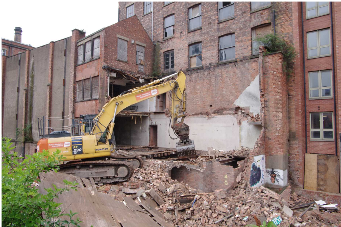
Figure 32 Rear (southern) section of 10 Short Hill during demolition Looking north-east. Note arched ceiling of cellar. Centre gable-ended section still intact at this stage
