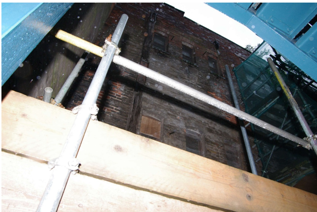
Figure 20 Number 10 Short Hill, east facing elevation Looking up through scaffolding at first and second floors. Note timber bracing
