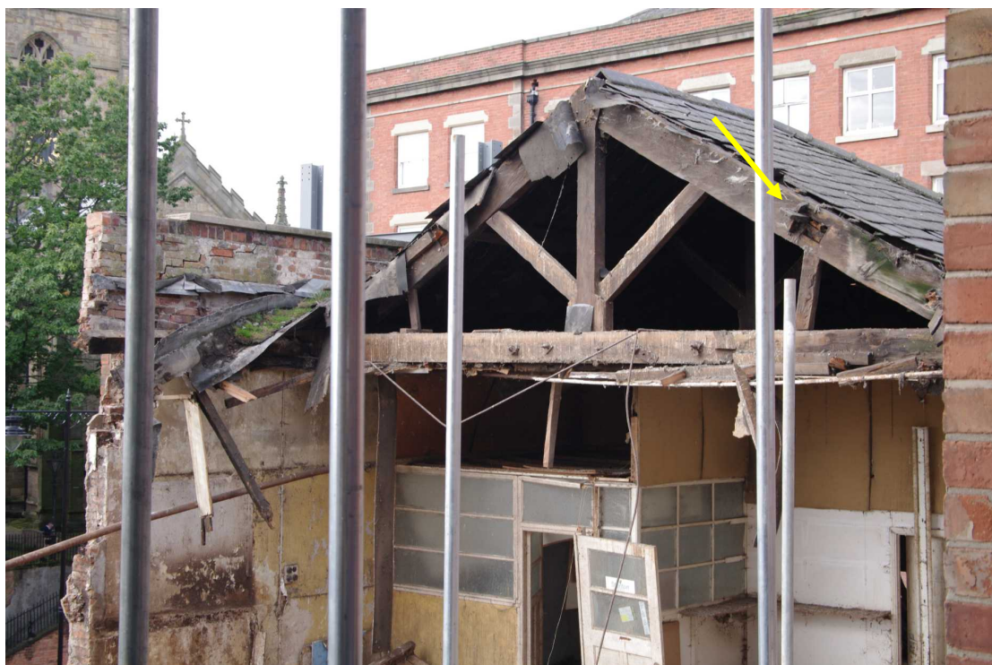
Figure 42 Close-up of roof front section structure Pegged tenon of purlin arrowed. Looking north-west
