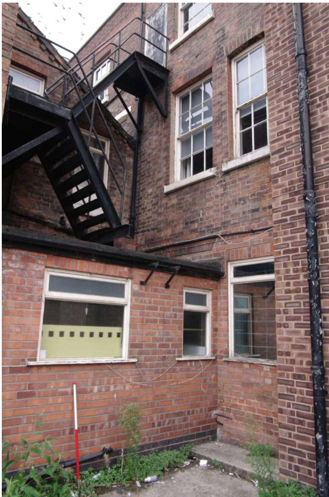
Figure 51 19th century extension, east facing elevation and link to main building Looking north-west. 1m scale
