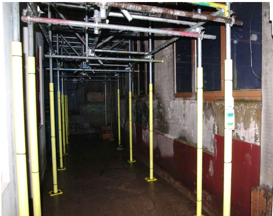
Figure 21 Number 10 Short Hill, east facing elevation Looking south-west at ground floor east wall from covered entrance
