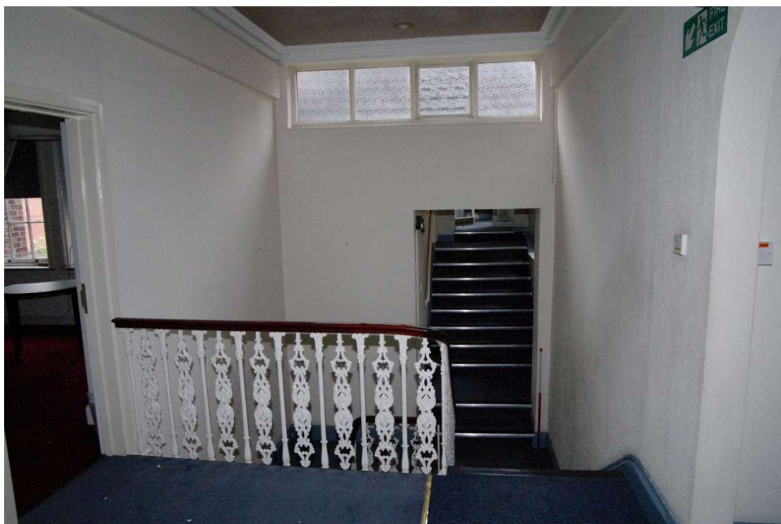
Figure 59 Stairs to first floor of 19th century extension Looking south-east from first floor of Number 56. 1m scale
