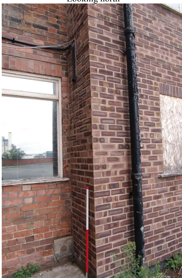
Figure 65 1960s extension, south facing elevation and ground floor joint Looking north-east. 1m scale
