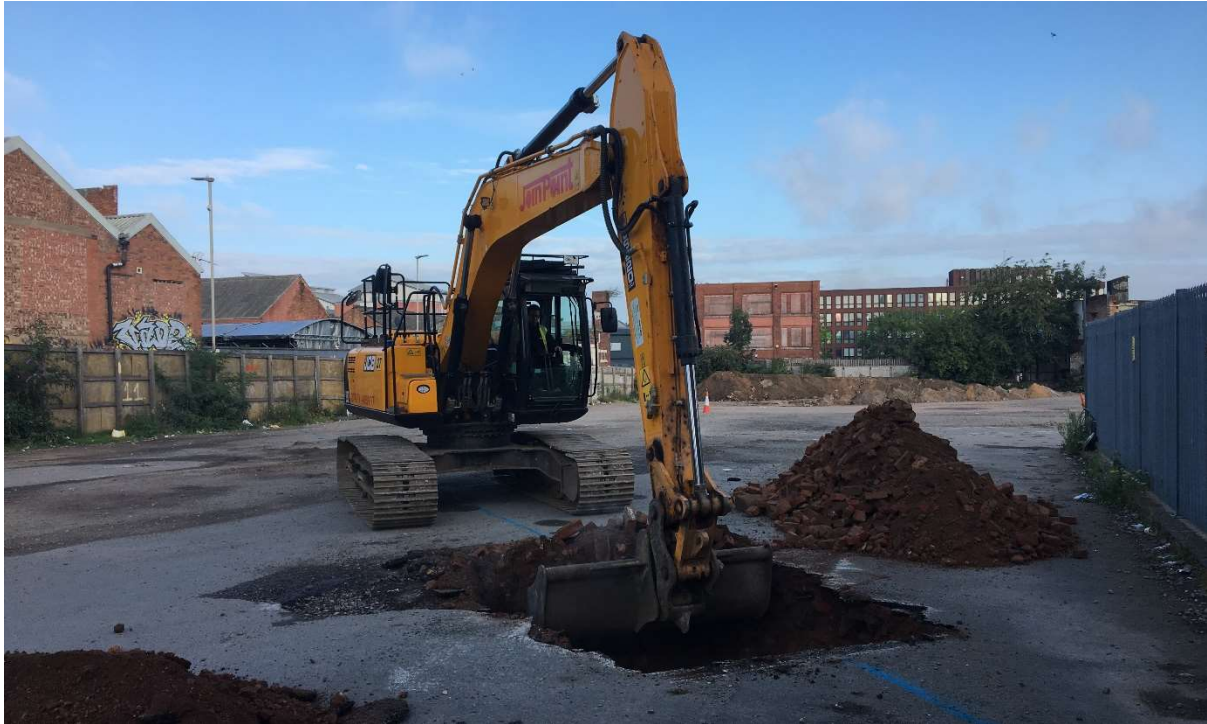
Figure 3: Looking north across the development area, with the mechanical digger excavating Trench 3.
