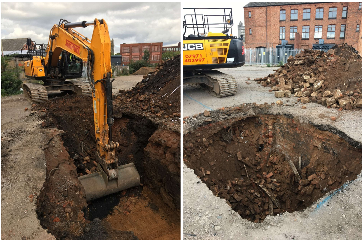
Figure 4: Left, the mechanical digger removing cellar infill from the west end of Trench 3. Right, test-pit excavated into cellar infill at the west end of Trench 4 to establish depth.
