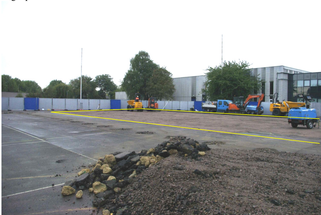
Figure 5 Site after removal of tarmac and prior to excavation of pads Looking south-west. Area highlighted by yellow line
