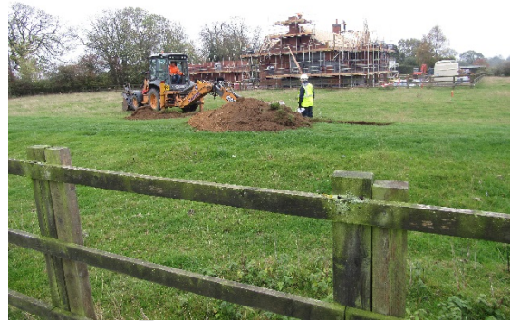
Far south end of site looking south. Mechanical excavator used on site
