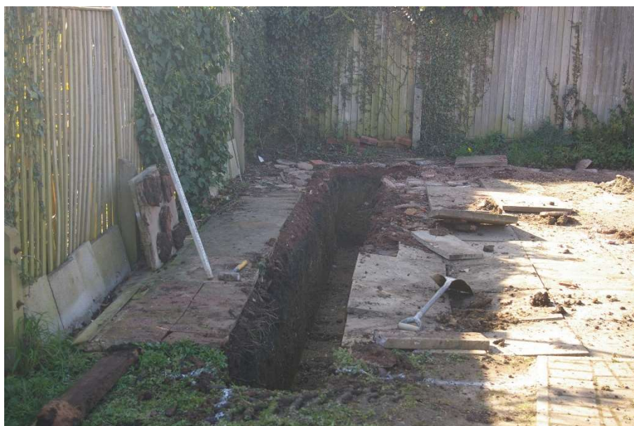
Figure 5: South side wall trench. Attempts to photograph walls of trenches were hampered by narrowness and shadow
