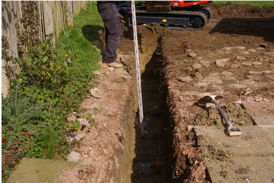
Figure 3: Contractor measuring depth of west back wall trench. Attempts to photograph walls of trenches were hampered by narrowness and shadow
