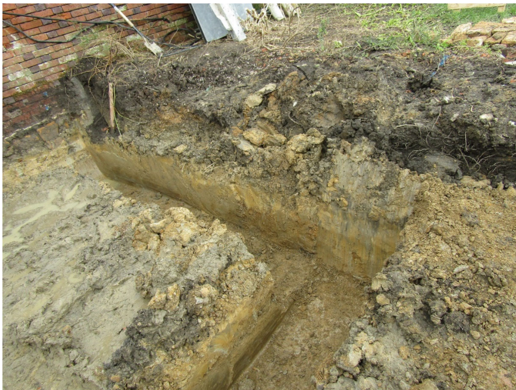
Figure 6: Foundation trenches at the north- east end of the site looking north.
