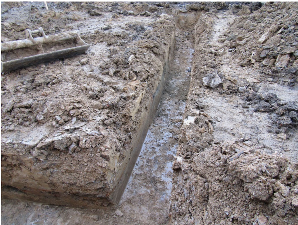
Figure 9: final trench to be excavated looking north-east, some oil in section, likely seeping in from the old farmyard above.
