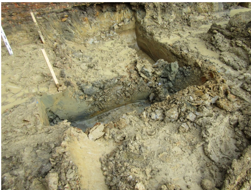
Figure 5: Foundation trenches at the north-west end of site looking north (For scale Trench is 0.65m wide, 2.80m long)
