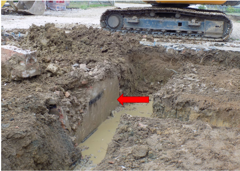
Figure 8: The remains of the brick-lined mechanic's pit in the side of the trench (arrowed). Looking southeast
