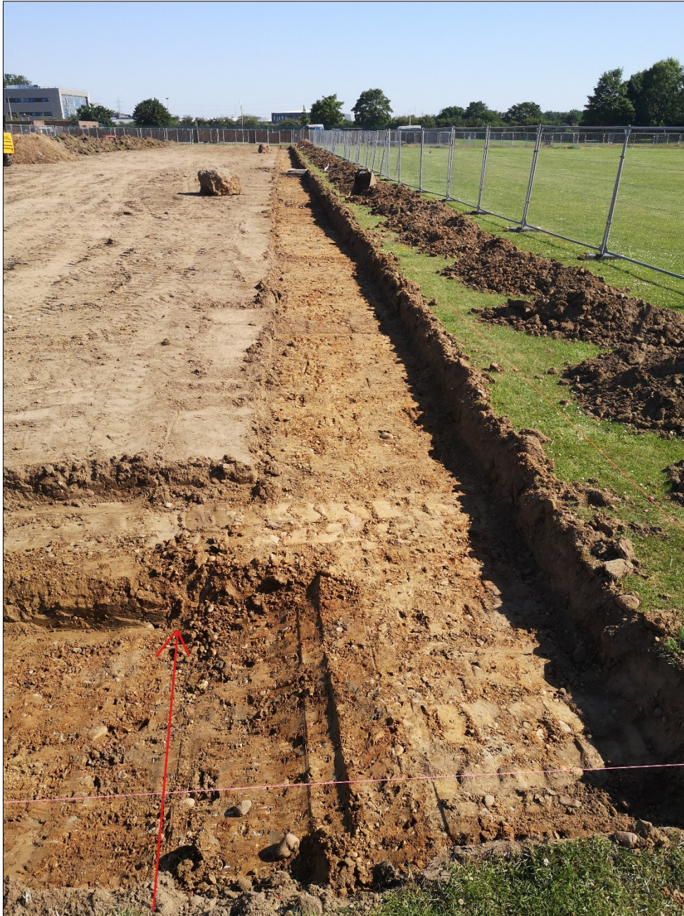
Fig. 10: Trench 1 south end, showing west edge of backfilled deep service, looking N
