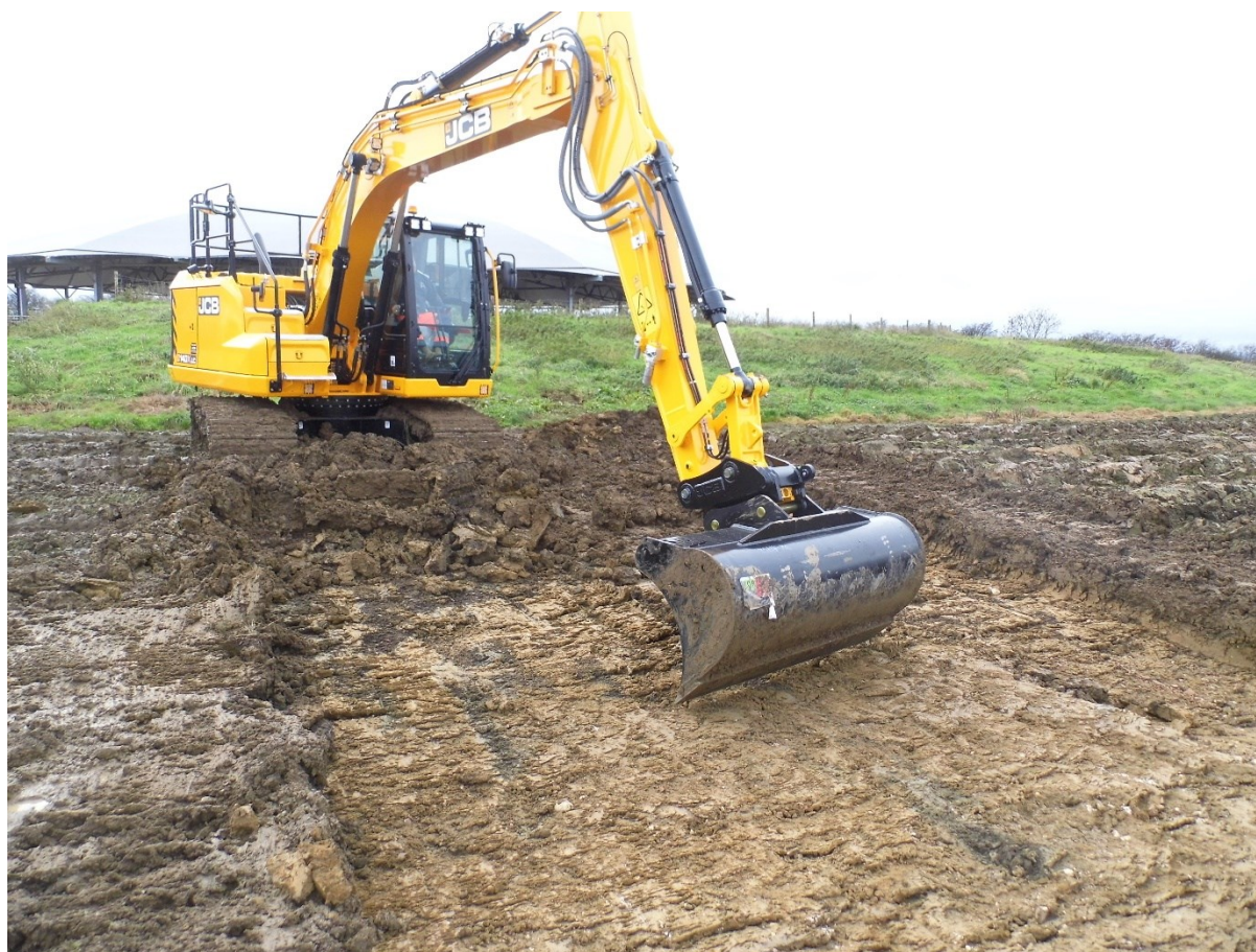
Figure 8: Stripping the shallow topsoil in the south-western corner with disturbance from recent ploughing.
