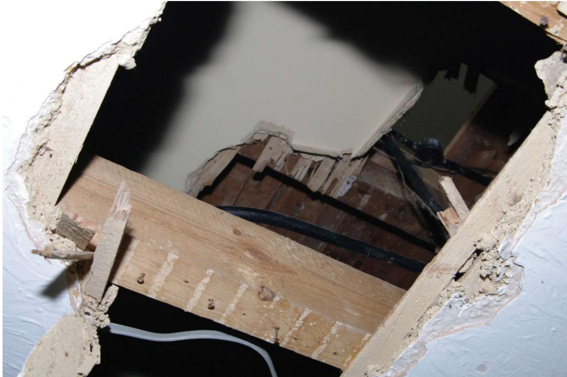
Figure 74: Hole in Room G7 ceiling
