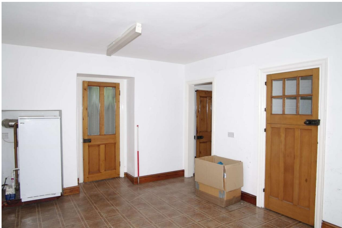
Figure 79: General view of Room G10 Looking north. 1m scale. The left hand door leads into entrance G11, the two right hand doors lead out to the doorways seen on the north-east facing elevation
