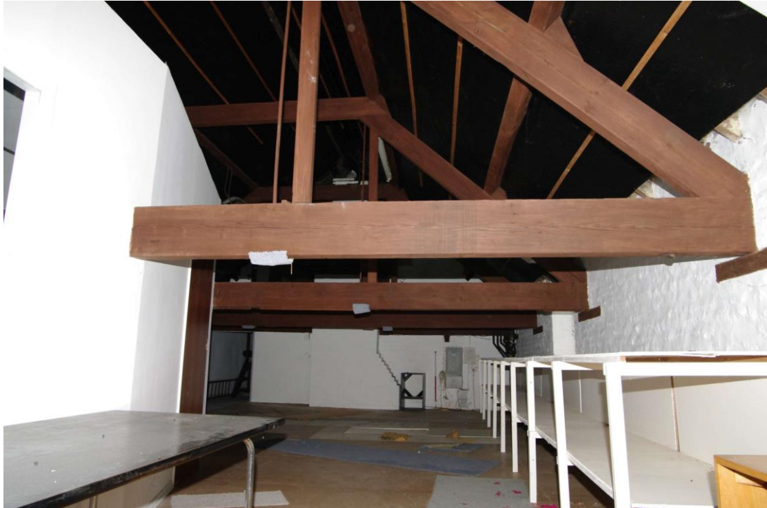
Figure 110: General view of R2 Looking north-east. 1m scale. The partitions on the left are wooden temporary walls
