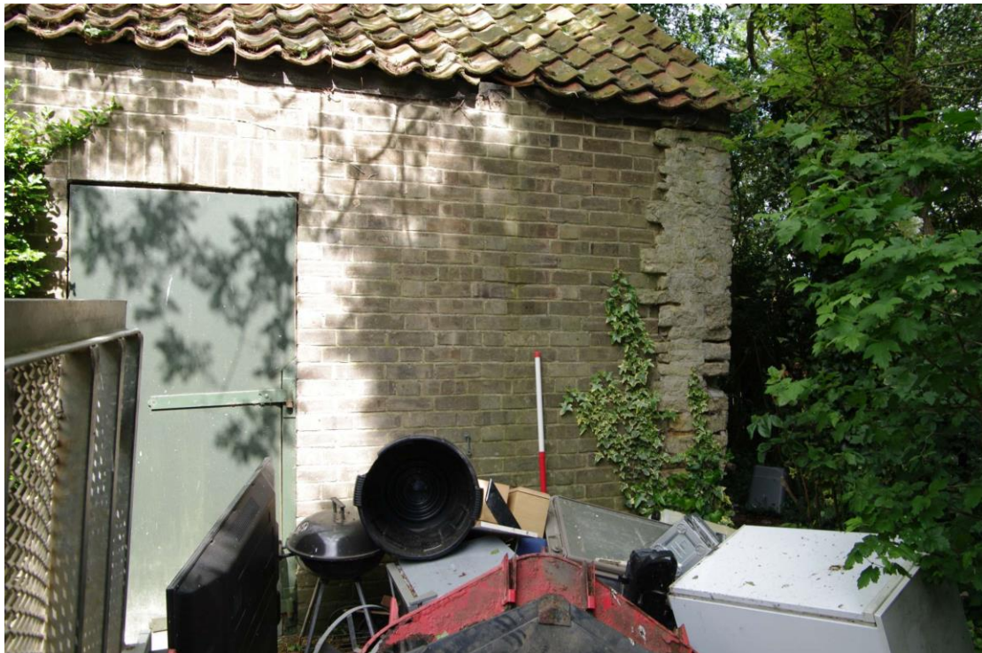
Figure 121: South-eastern outbuilding brick infill on south-west facing elevation Looking north. 1m scale
