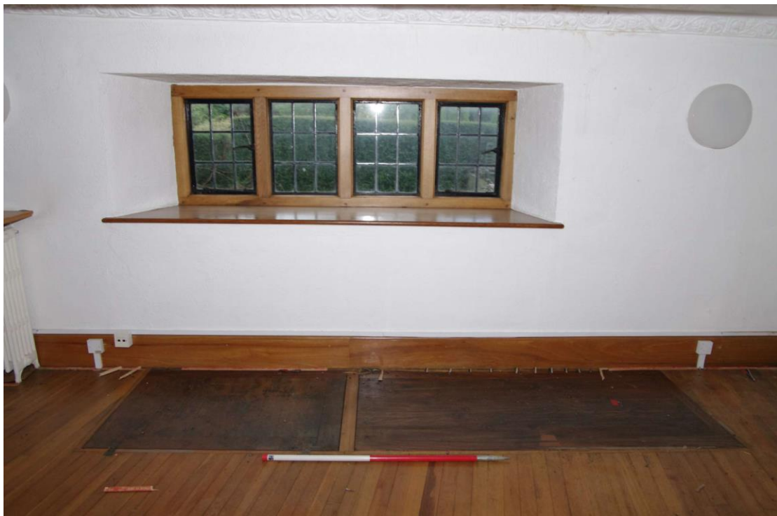
Figure 56: Room G1, north-west end window Looking north-west. Note 1m scale lies in front of the hatches on the floor
