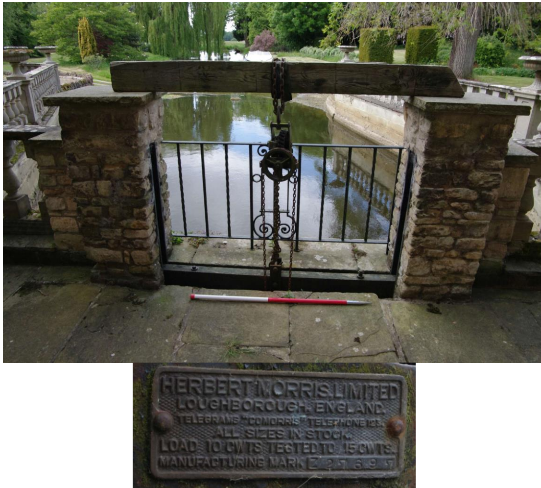
Figure 32: Internal water wheel sluice gate Inset below is the maker's plate. Looking north-west. 1m scale
