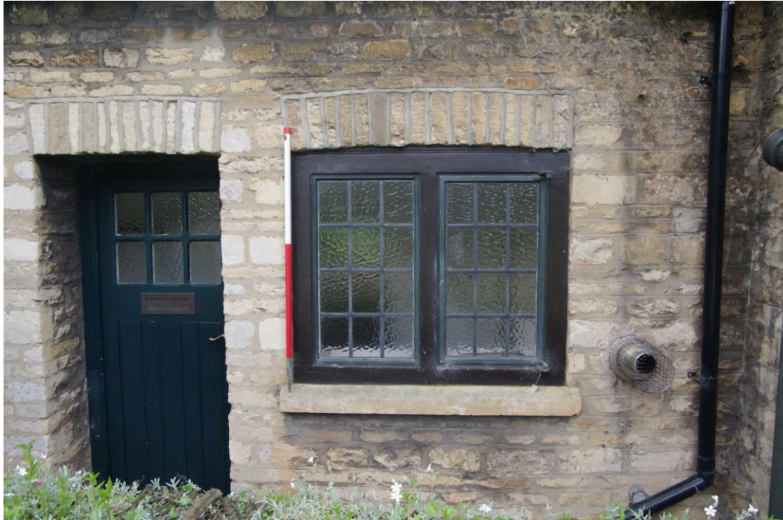
Figure 36: Window and door detail, north end of NW facing elevation Looking south-east. 1m scale
