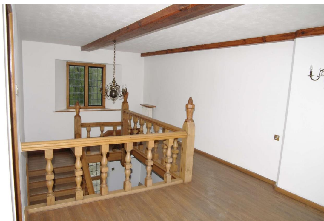
Figure 88: F4 stairwell and landing Looking south. Note step in wall on left where the inserted chimney stack rises up from the ground floor
