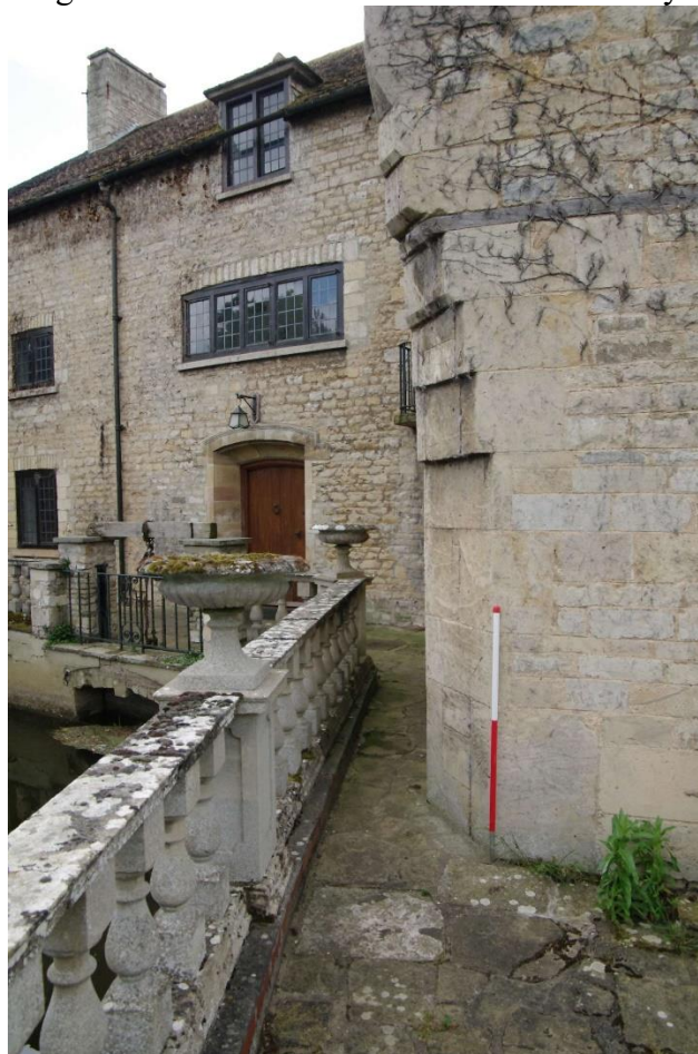
Figure 21: Chamfered corner of western end of the NW facing elevation Looking south-east. 1m scale
