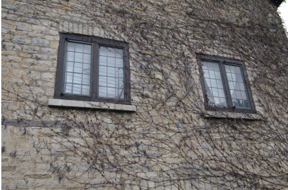
Figure 18: First floor windows, western end of the NW facing elevation Looking south-east
