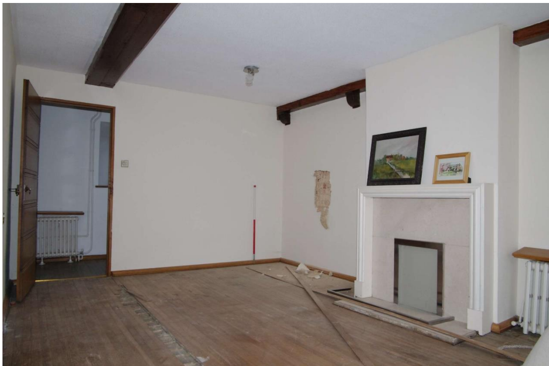
Figure 93: General view of Room F6 Looking north. 1m scale. Doorway to corridor F4 on left
