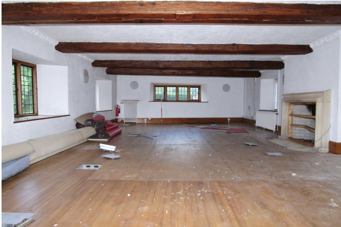
Figure 53: Ground floor room G1 Looking north-west. 1m scale. Note angle of far wall
