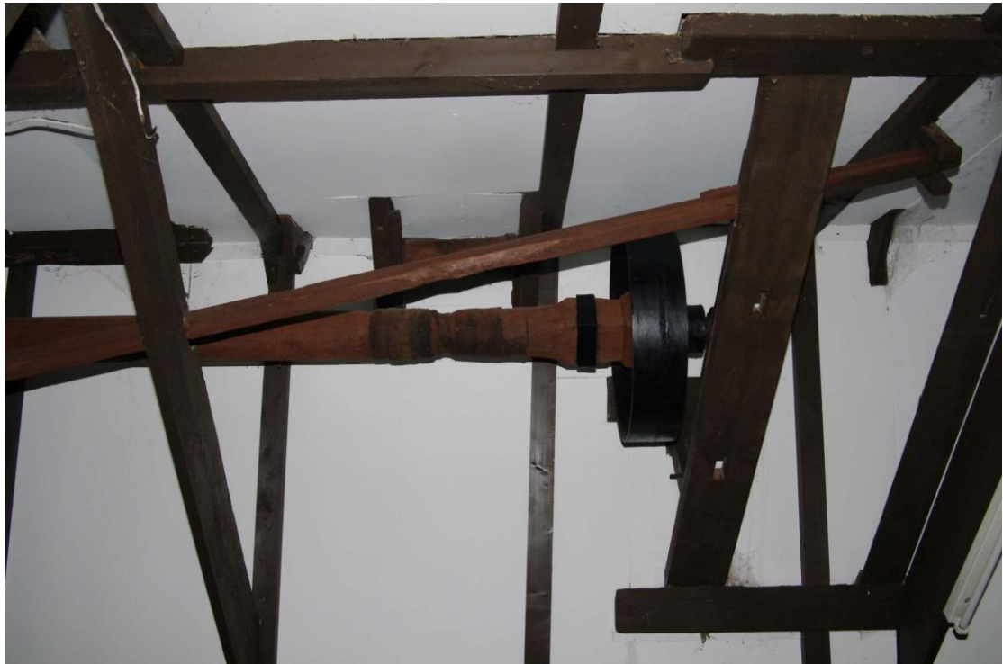
Figure 108: Sack hoist shaft showing rope wear
