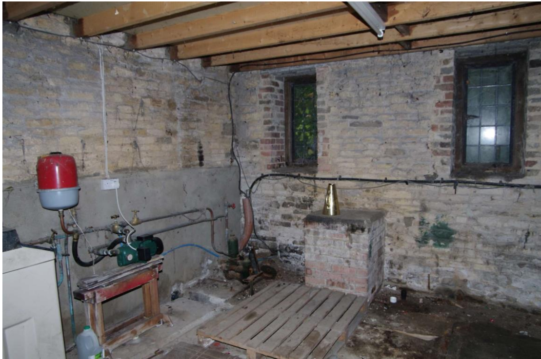
Figure 127: Space within the northern end structures of the barn Looking north-west. Note windows on external north-west facing elevation
