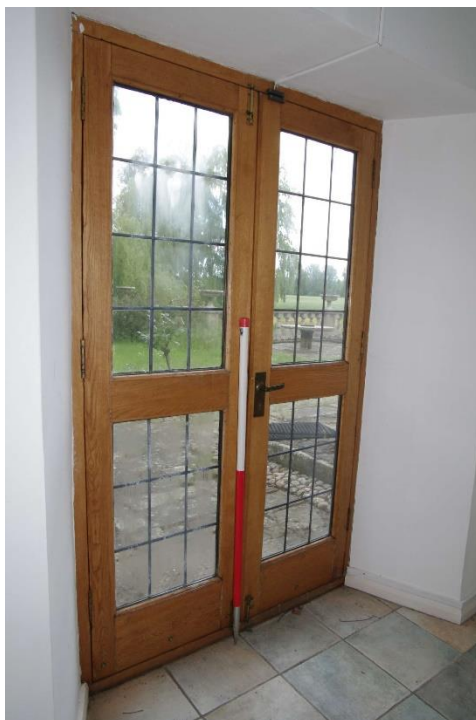
Figure 83: Room G12, doors to south-east facing elevation Photographed from G10 doorway looking south. 1m scale
