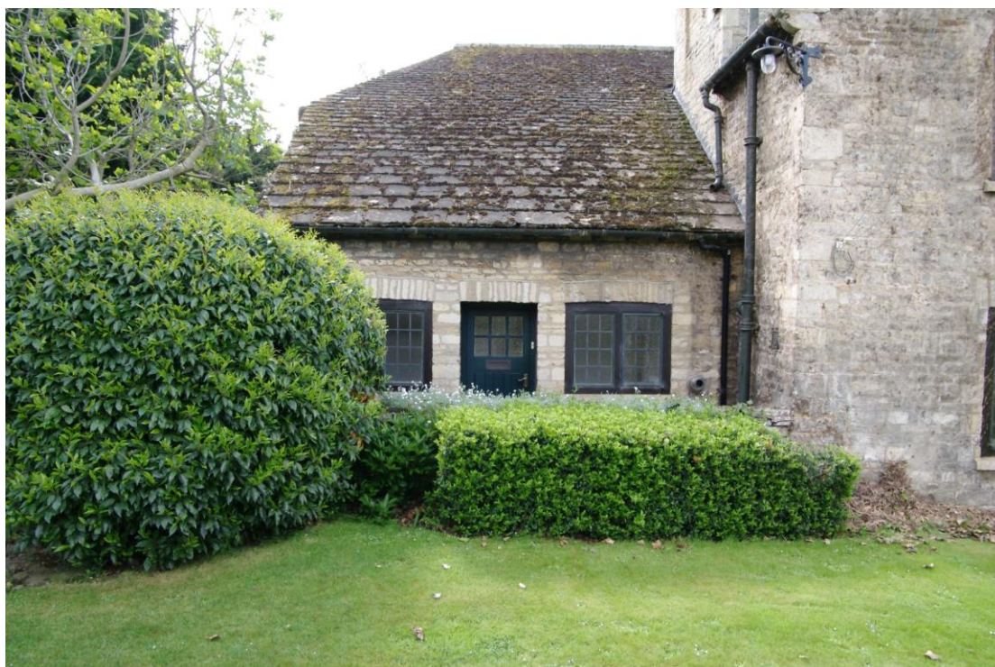
Figure 35: Northern end of the north-west facing elevation Looking south-east. See also Figure 33
