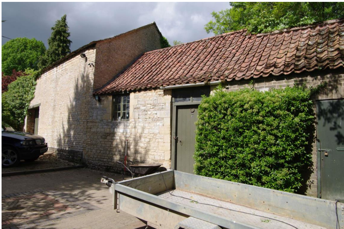
Figure 119: Barn and outbuilding junction on south-west facing elevation Looking north. 1m scale
