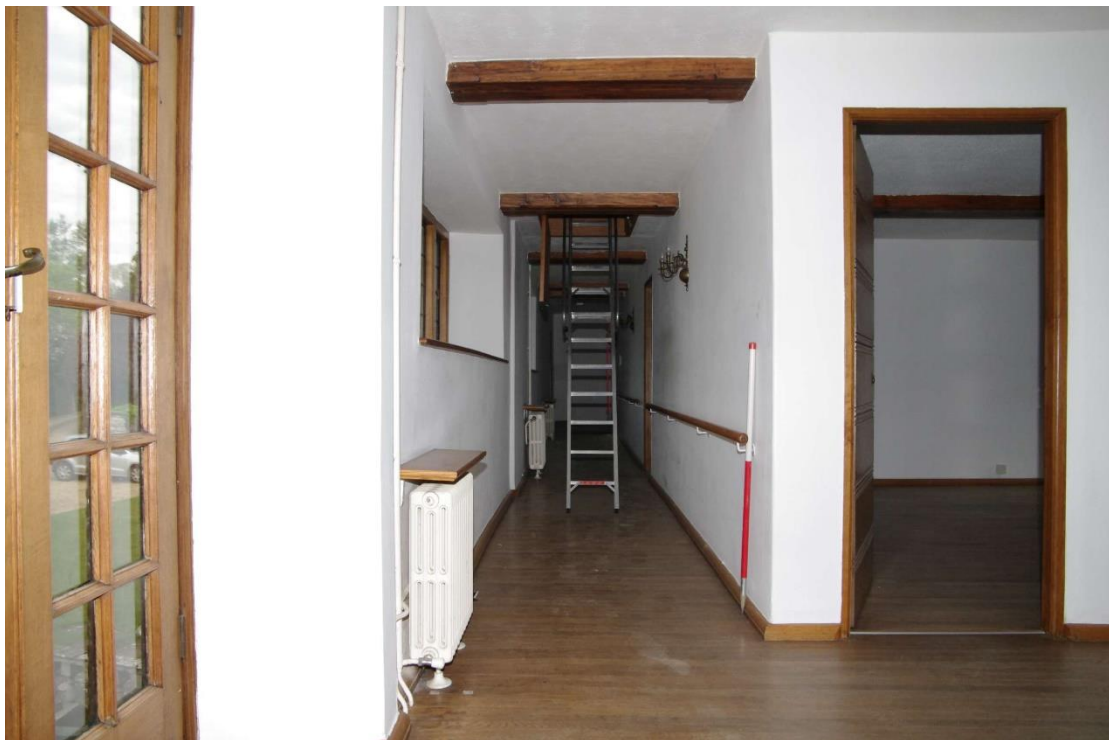
Figure 90: F4 landing and corridor Looking north-east. 1m scale. The metal steps are the only access to the roof space. Note the step in wall thickness just beyond the corridor window close to the steps. Doorway to Room F5 on right of picture. Balcony doors on left
