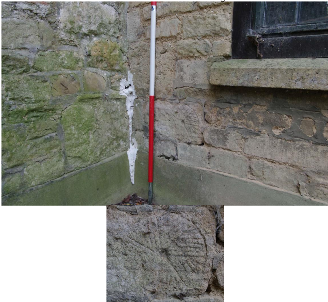
Figure 40: Carved picture of a mill stone on the north-east facing elevation Looking south. 1m scale. Lower picture: close up
