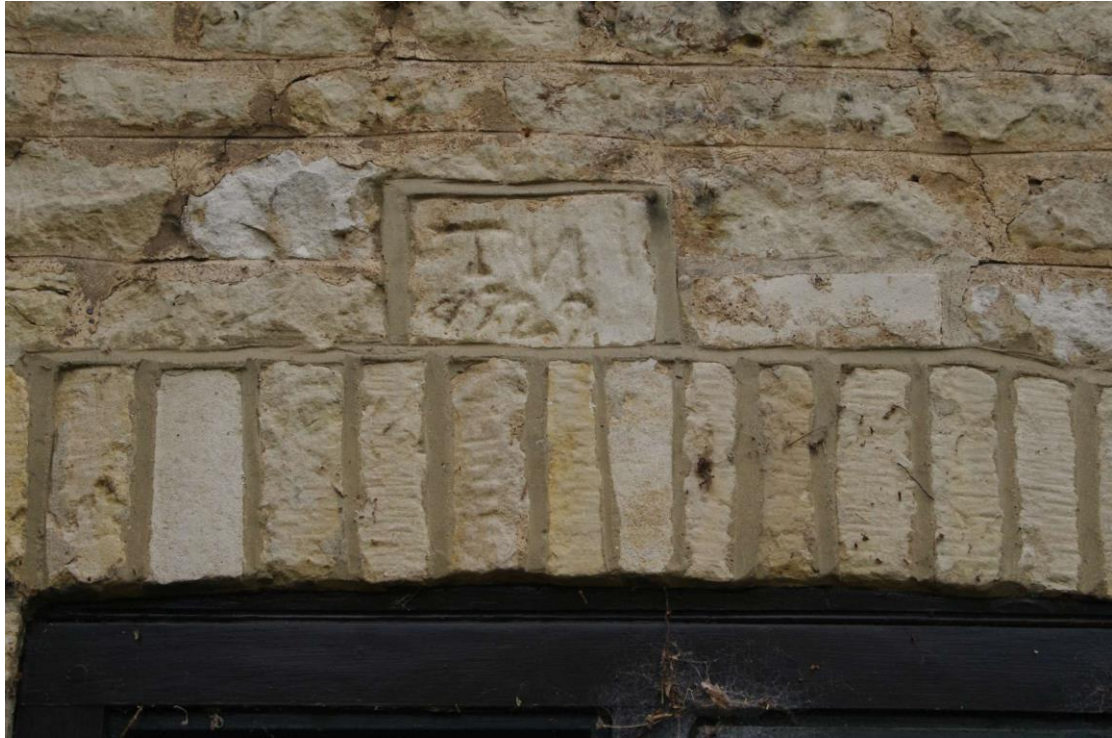
Figure 30: Date stone above ground floor window of centre section, NW elevation Looking south-east
