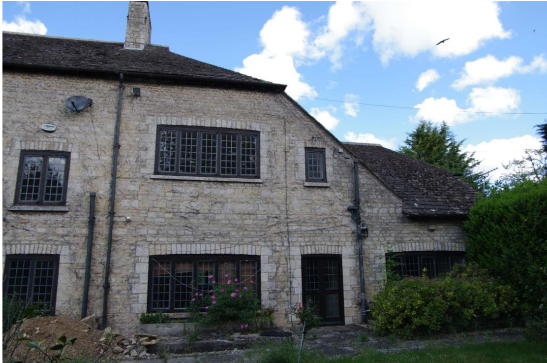
Figure 44: Northern end of the south-east facing elevation Looking north-west. Possible line in stonework can be seen at first floor level to the side of the pipe on the right
