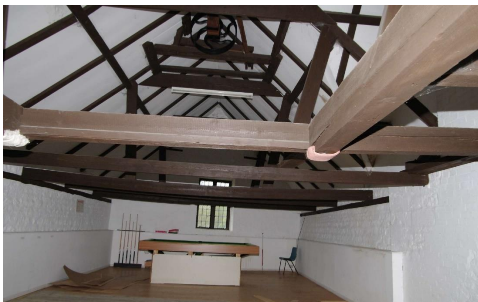
Figure 104: General view of R1 Looking north-west. 1m scale. Sack hoist in apex of roof
