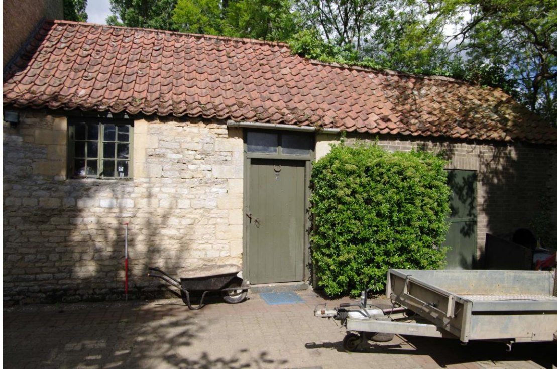
Figure 120: Outbuildings, south-west facing elevation Looking north-east. 1m scale. Note brickwork on right hand building
