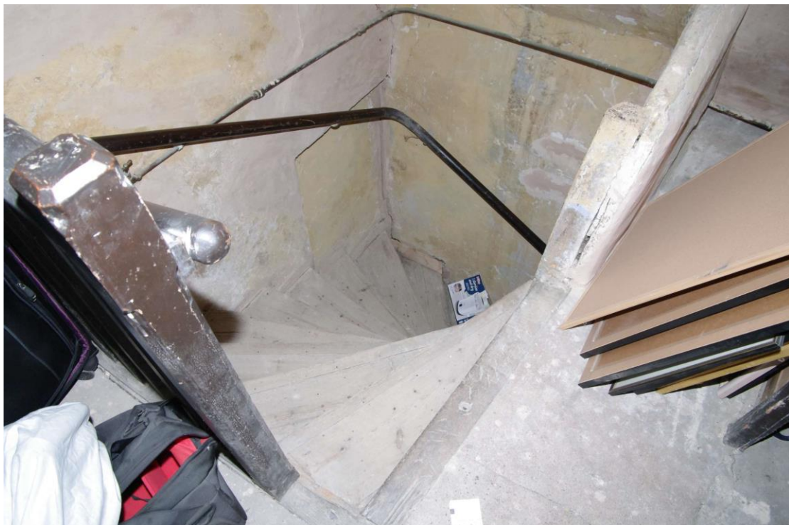
Figure 34 Second floor service stairs Looking down from second floor. Blocked window by angle in handrail
