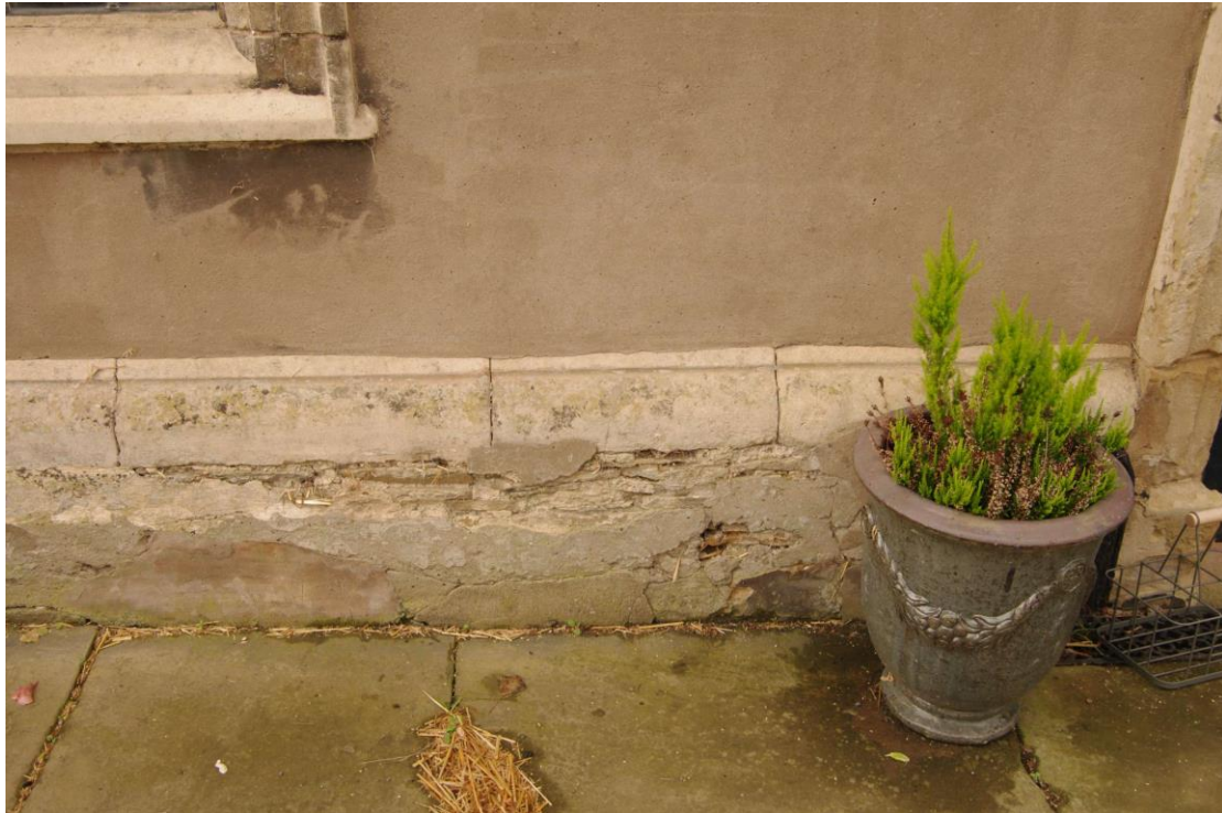
Figure 5 Stone plinth on which the 1691 range sits Looking south on eastern side of front door. Note how the plinth consists of a moulded stone course above stuccoed rubble
