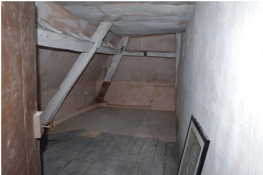
Figure 44 Former second floor landing and stairs in NW corner of house Looking north. The boarded area at the far end indicates where the stairs were located. Note the small window (top right) which lit the stairs
