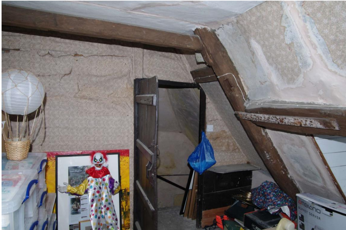
Figure 37 Second floor, inside the partitioned room Looking south-east. The door may be moved slightly to the left
