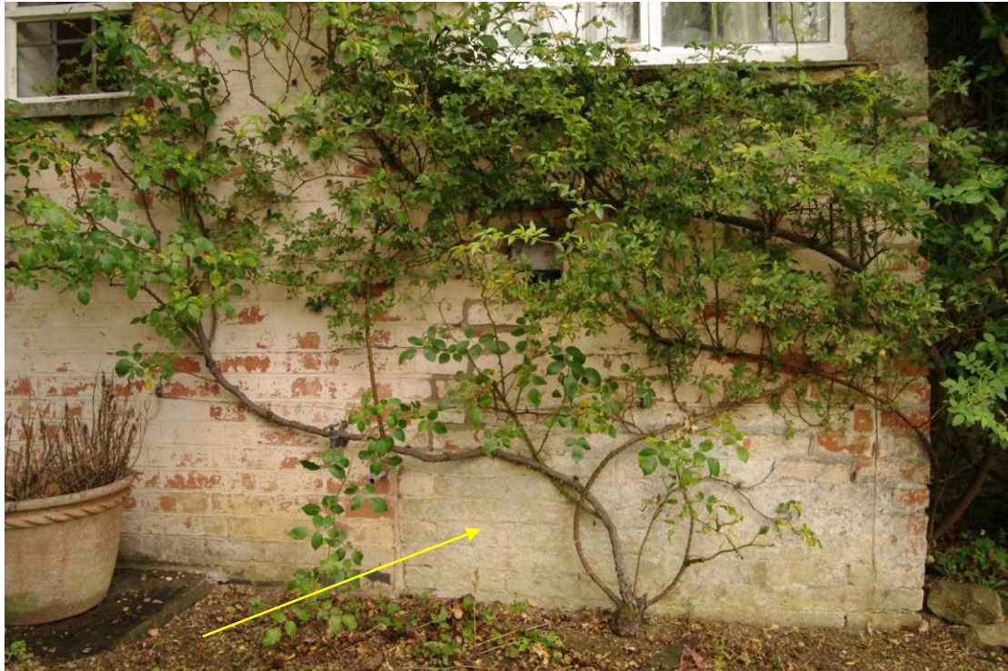
Figure 19 Blocked opening on extension Looking east. Arrow points to blocking brickwork
