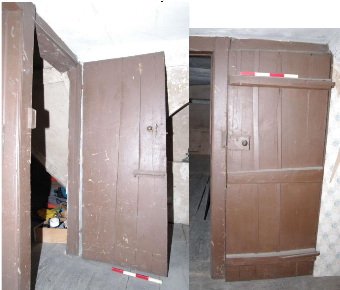
Figure 42 Second floor. Wide-boarded door from middle room to rear range 0.4m scale. This doorway is proposed to be blocked
