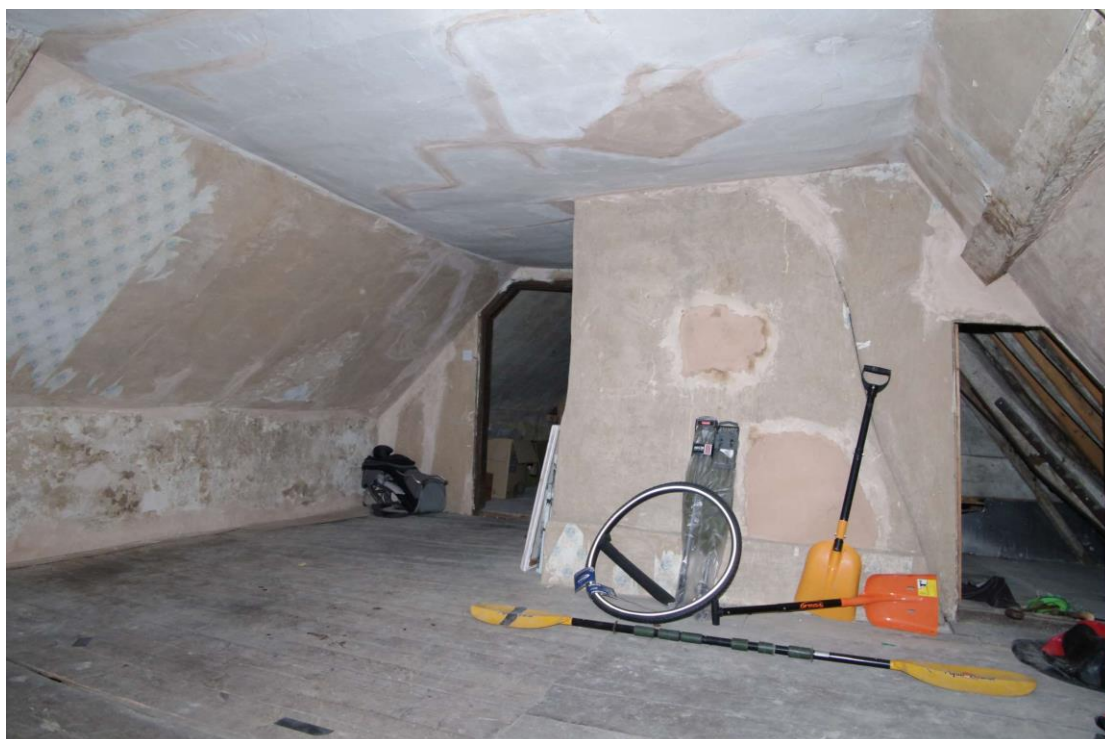
Figure 40 Second floor, middle room Looking north-east towards partition wall corridor (on left). A new bathroom will be inserted into the space on the left of the picture
