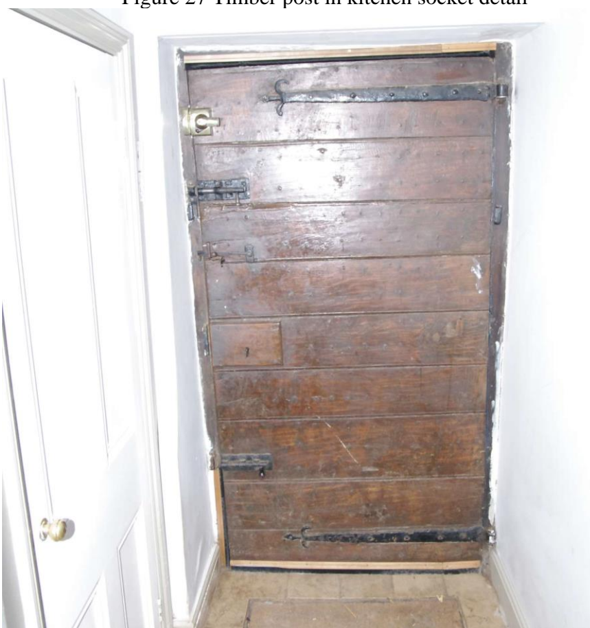
Figure 28 Rear kitchen door detail Looking south. Note wooden lock case and the strap hinges. Inserted toilet on left
