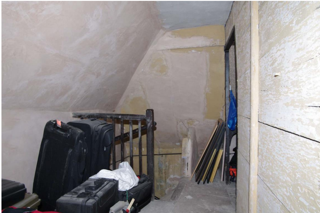
Figure 33 Second floor and top of service stairs Looking south. Note boarded partition wall on right
