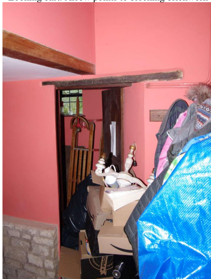
Figure 20 Doorway to toilet within single storey extension Looking south-west. Stair to cellar go down to left of picture. The visible window is the one shown in Figures 16 and 18
