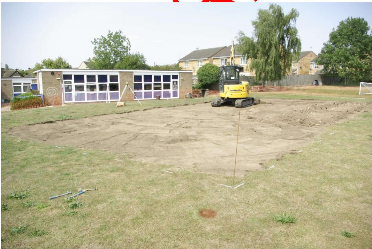
Figure 8 Games area following turf stripping Looking north-west. The two goal areas have yet to be stripped
