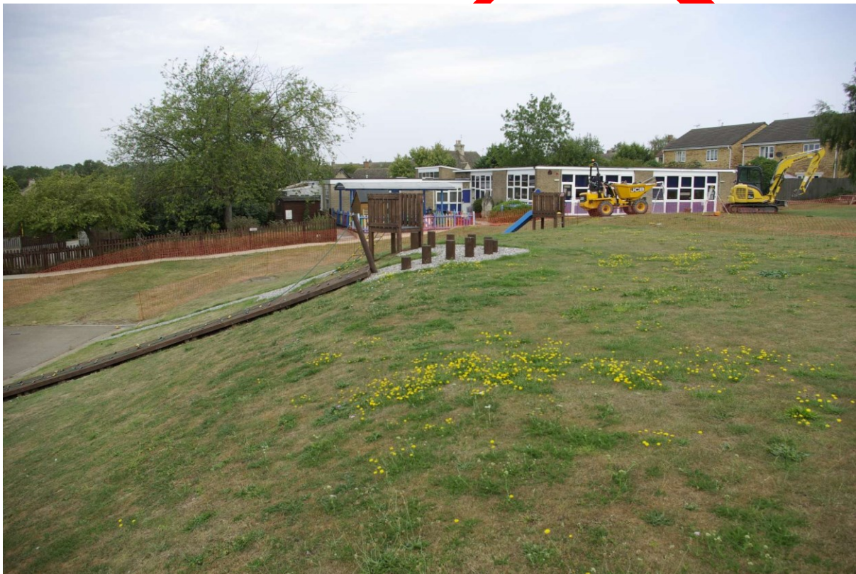
Figure 6 General view of site and terrace Looking north-west. The games area is located where the excavator is standing
