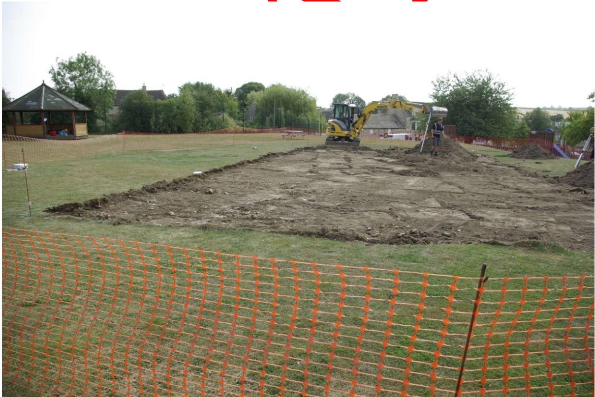
Figure 10 Stripped games area from the north With the exception of the spoil heap the area is at maximum depth
