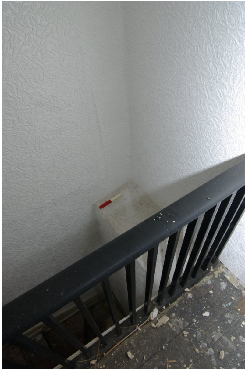
Figure 8 Change in Wall Thickness Between Ground & First Floor, No 47.
