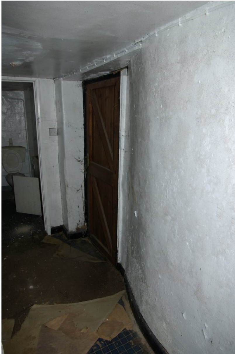
Figure 9 Unusual Wall Angle 47 B.
