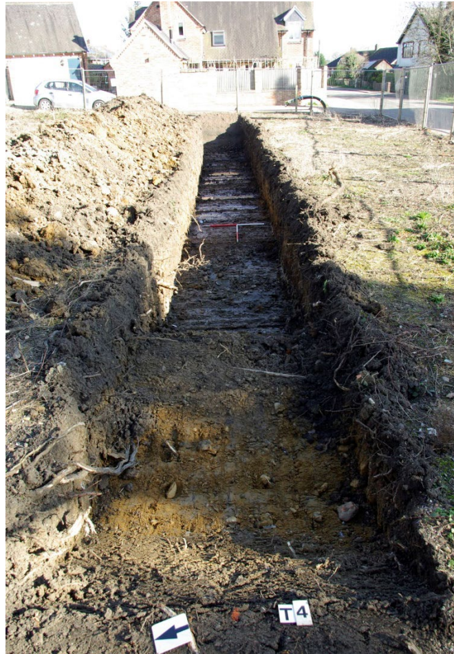
Figure 15 Trench 04 Looking east. 1m scales. Ashby Road on right. Water pipe in foreground
