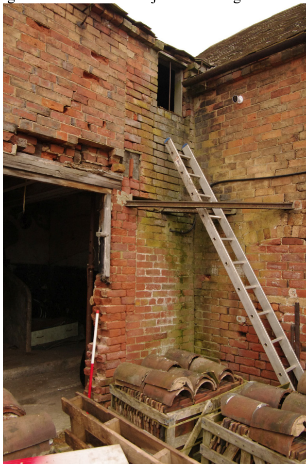
Figure 20 Detail of the joint between the former house and hayloft Looking north-east. 1m scale
