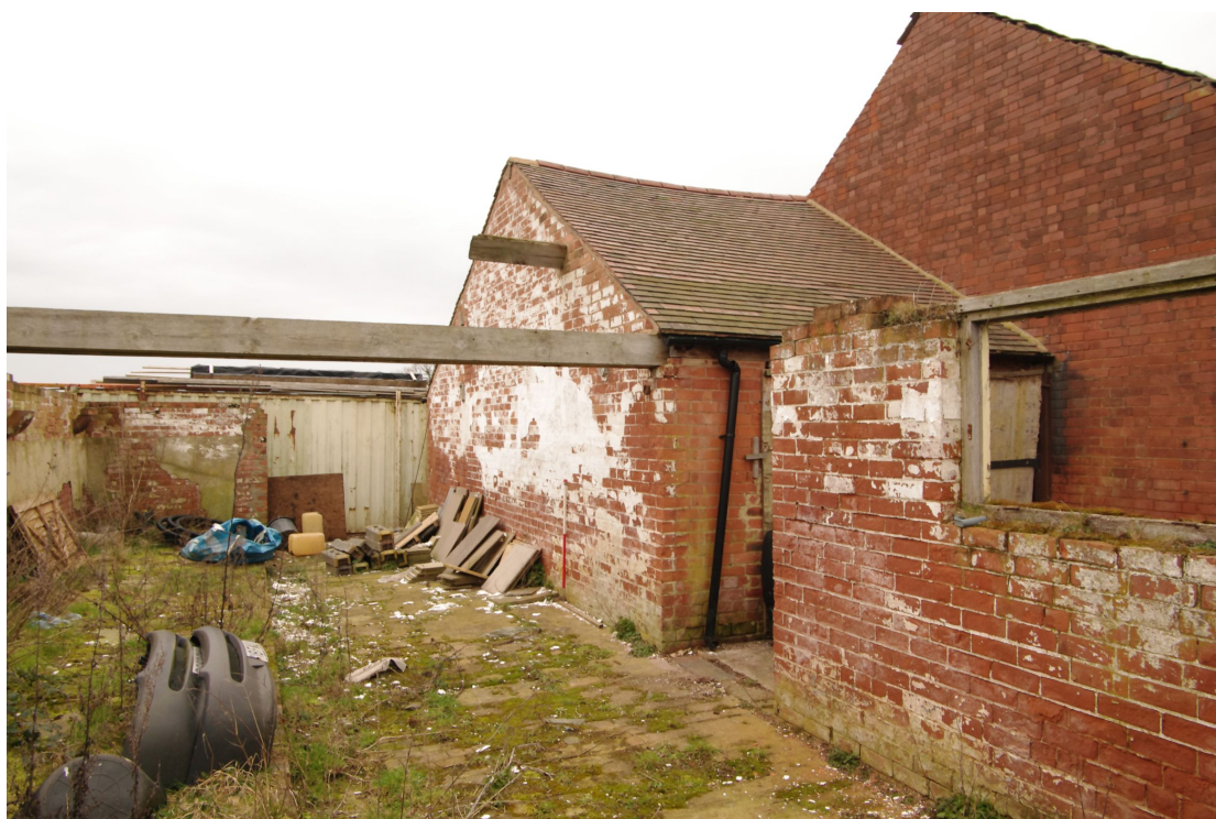
Figure 47 Inside the milking parlour, Barn 3 range Looking north-west. 1m scale. Extension and cart shed on right
