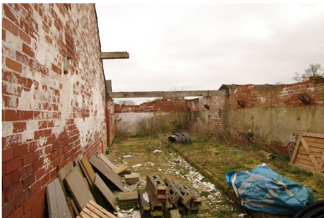
Figure 46 Inside the milking parlour, Barn 3 range Looking east in the roofless building. 1m scale. The gable end of the extension seen in Fig. 45 is on the left
