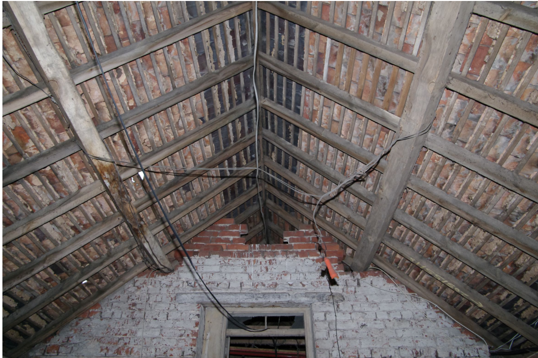
Figure 35 Roof detail in first floor room at northern end of Barn 1 range Looking north
