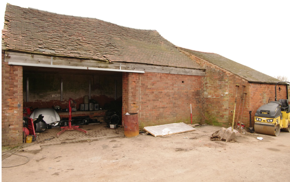
Figure 41 West facing elevation of former cart shed, Barn 3 range Looking south-east. 1m scale. The lower wide building to the right is later than the cart shed
