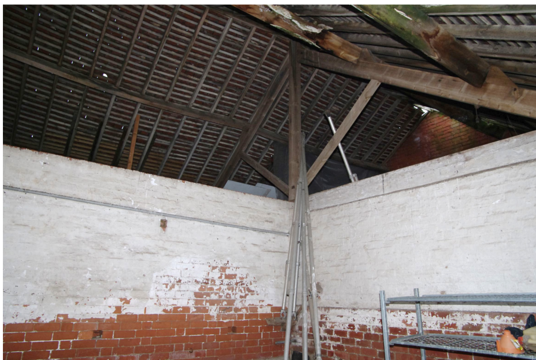
Figure 42 Inside Barn 3 range, the former cart shed Looking north-west in the south-eastern room. Internal brick walls, which are original, sub-divide the space into three
