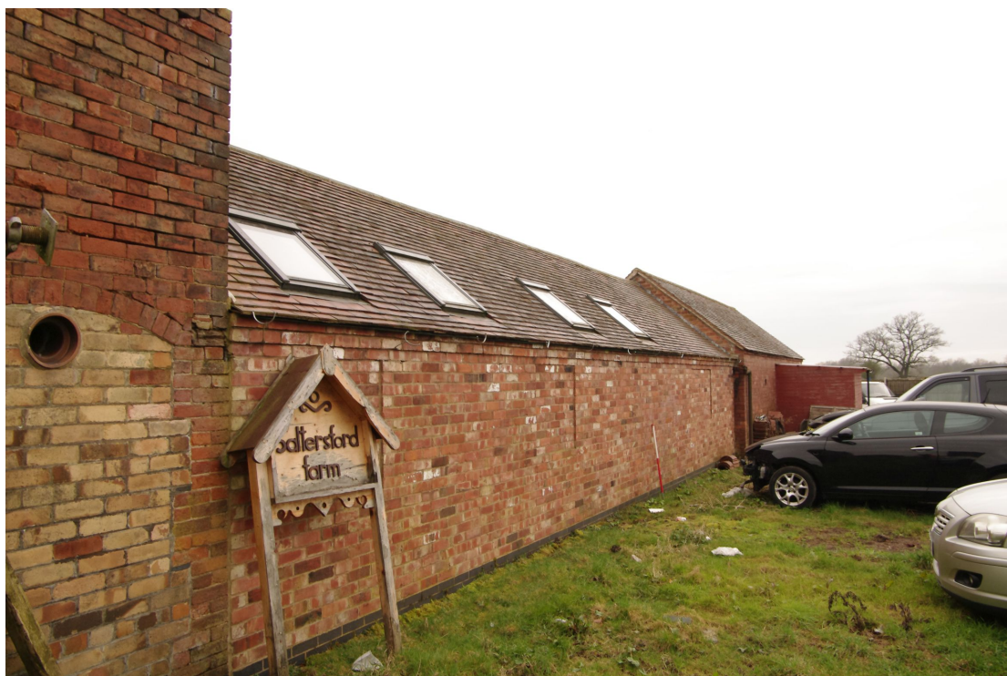
Figure 13 Single storey range of north facing barns (Barn 2) Looking south-west. 1m scale. The wall has been rebuilt and now has a blue-brick damp-proof course. The roof has also been re-covered and repaired
