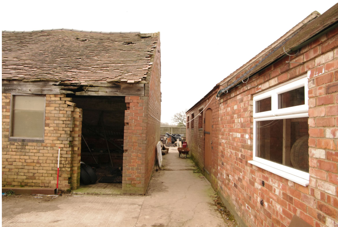
Figure 16 South facing elevation of Barn 2 range Looking west. 1m scale. Former cart shed Barn 3 on left
