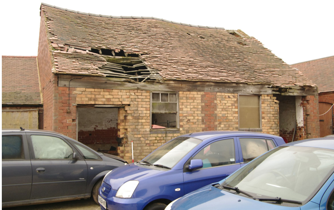
Figure 39 East facing elevation of Barn 3 range Looking north-west. 1m scale. The open-fronted cart shed building with a central red-brick pillar has been infilled with pale bricks. Note the large timber lintel
