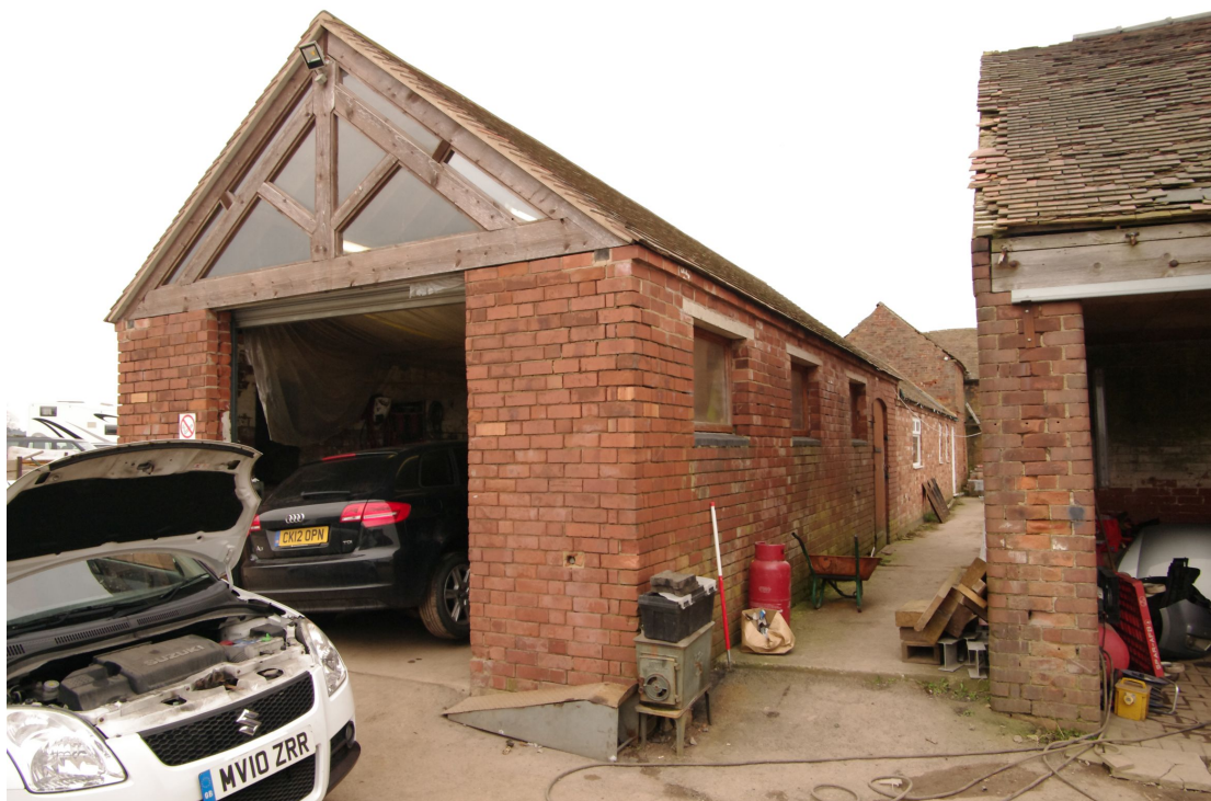
Figure 15 West facing gable end of Barn 2 range Looking north-east. 1m scale. The internal details of this single storey range are modern. Note concrete lintels. The edge of Barn 3 is on the far right
