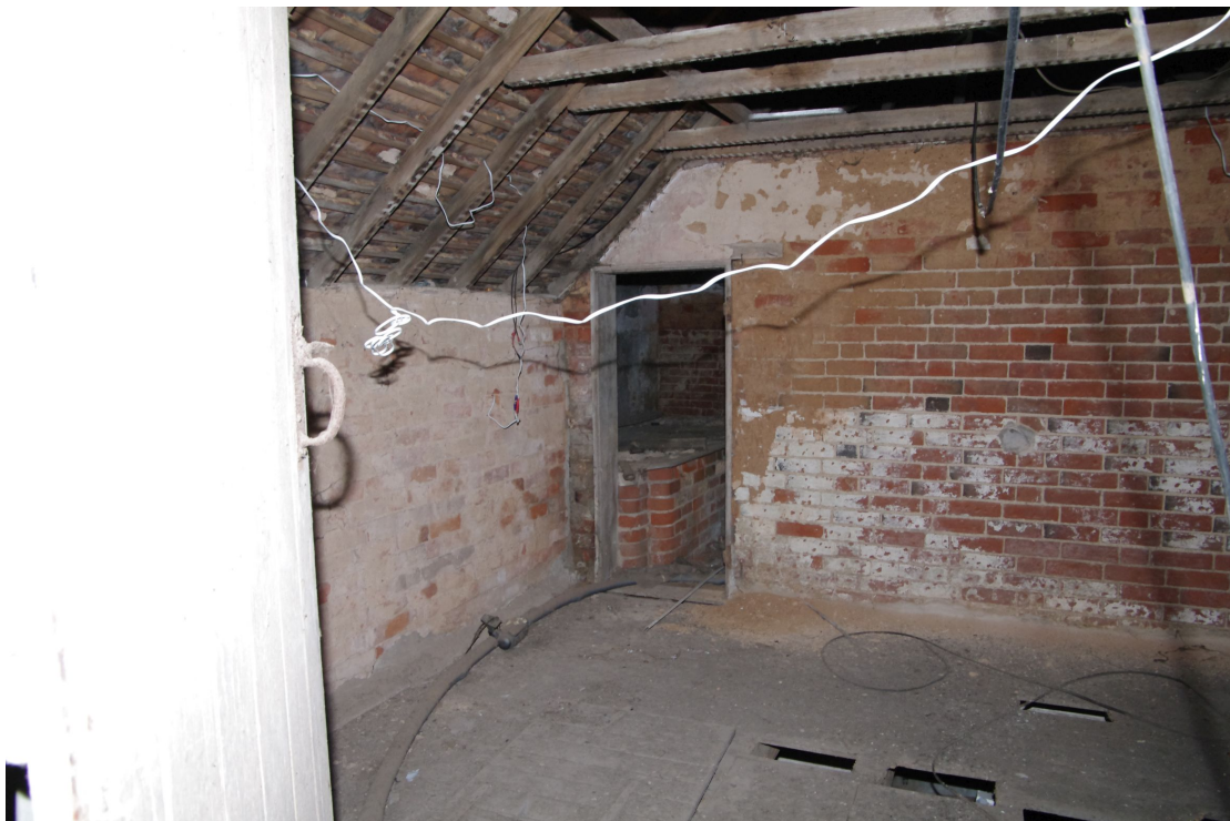
Figure 36 First floor room at north end of Barn 1 Looking north-west. The doorway leads into the rooms seen in Figs 28 and 29. Note that this room was plastered and had a ceiling and may have been part of the former house
