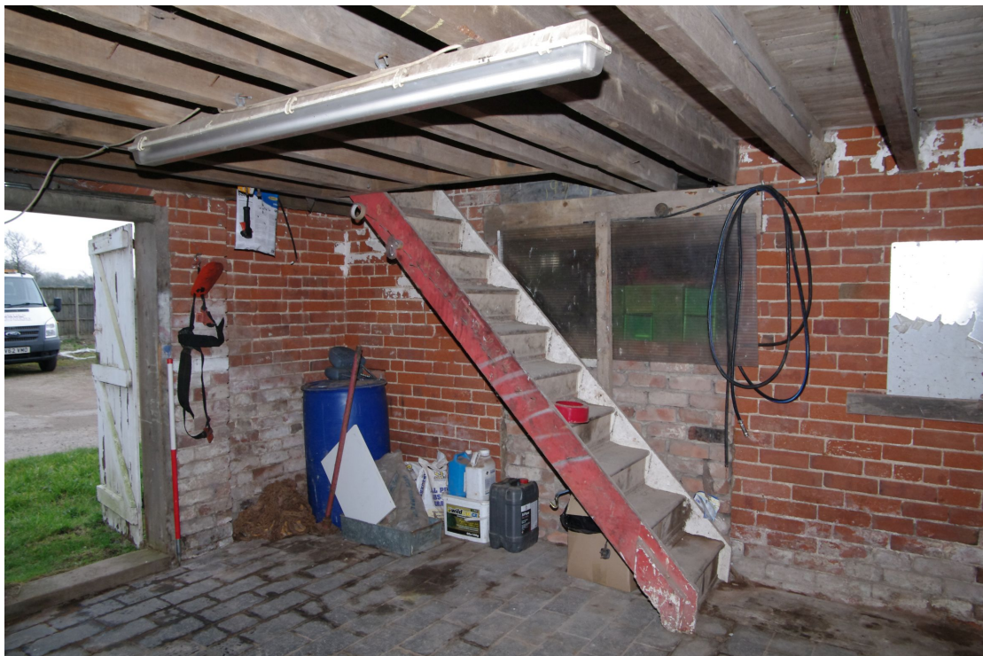
Figure 30 Ground floor room at northern end of Barn 1 range Looking south-east. 1m scale
