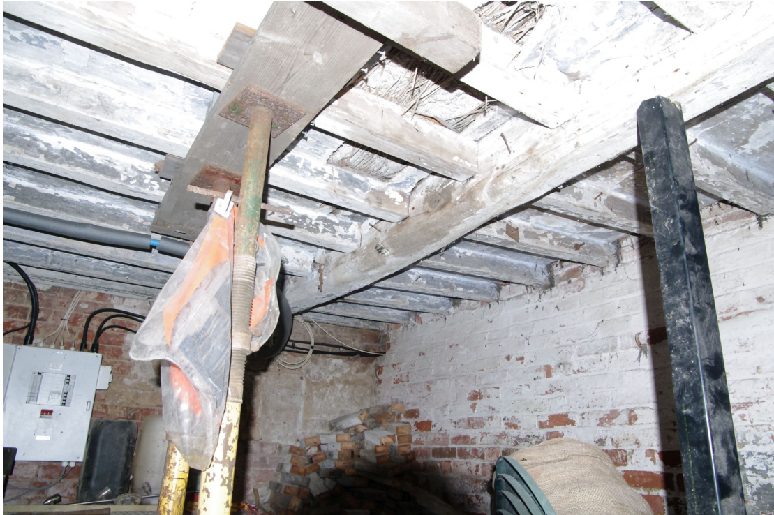
Figure 27 Ground floor room of former house Looking south-west. Note straw and plaster ceiling
