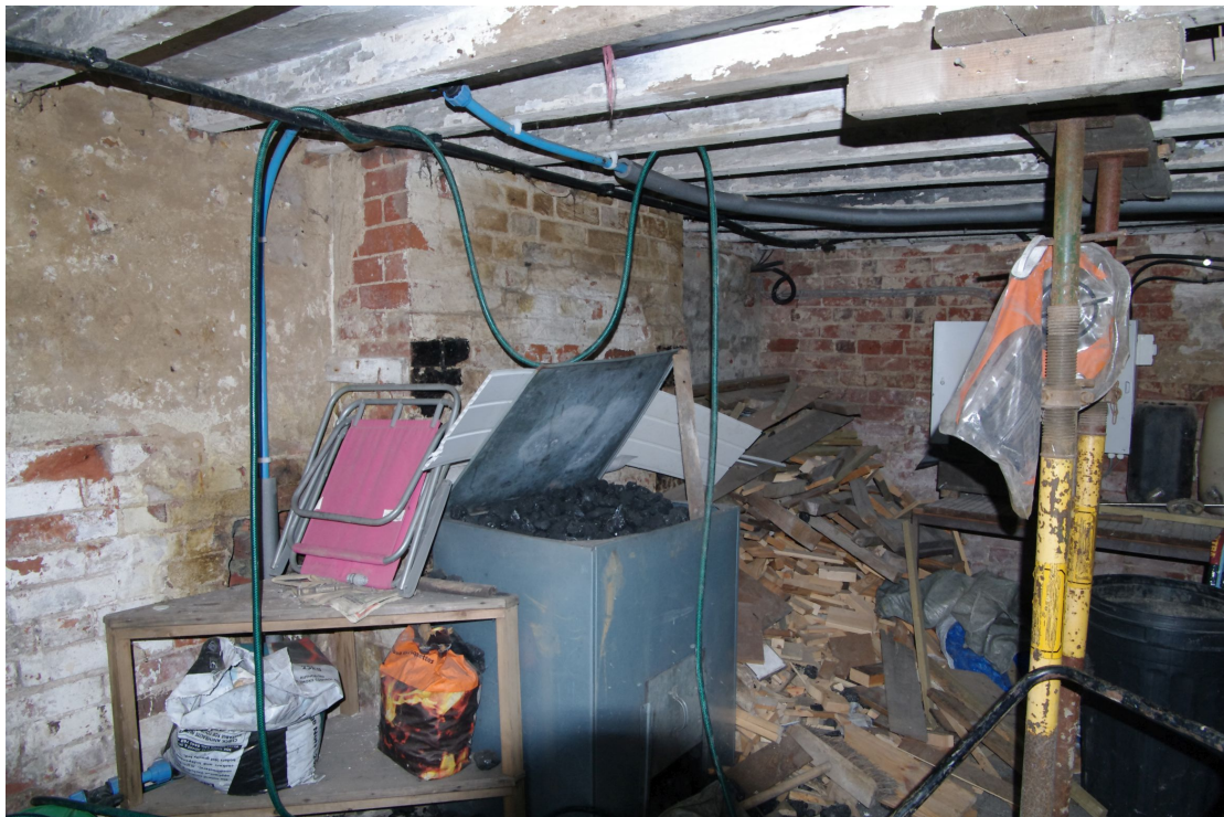
Figure 26 Ground floor room of former house Looking south-east. Fire place is behind the coal bunker and wood pile
