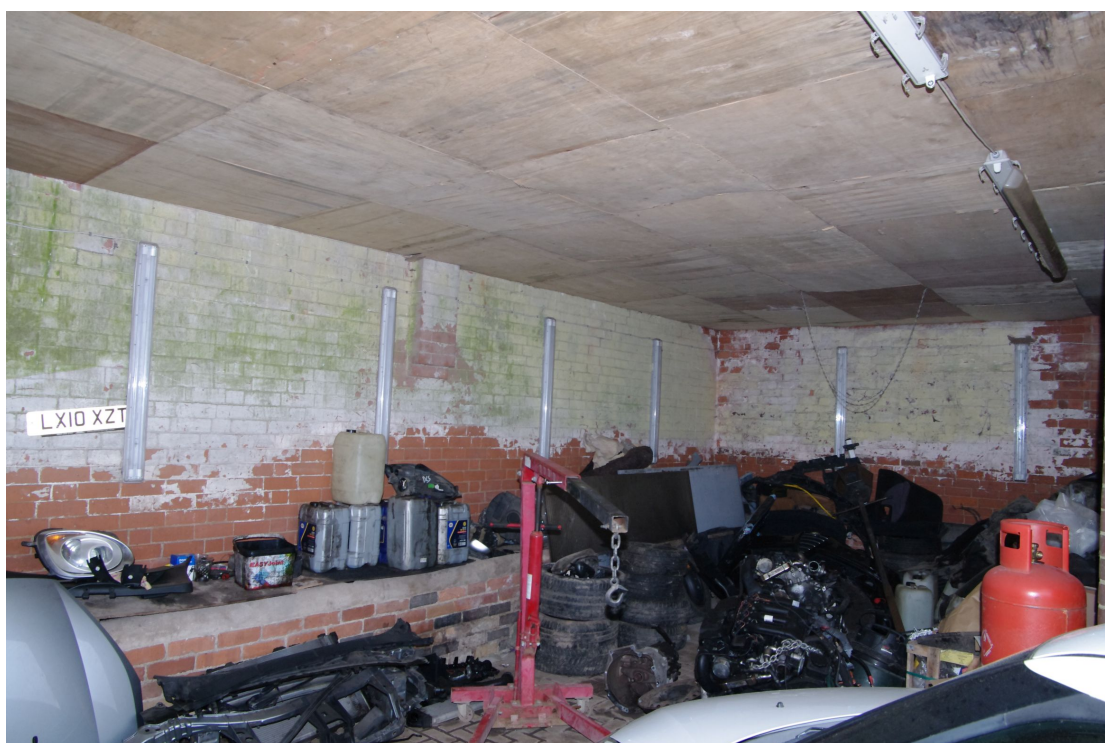
Figure 44 Inside Barn 3 range, the former cart shed Looking south-east in the western room
