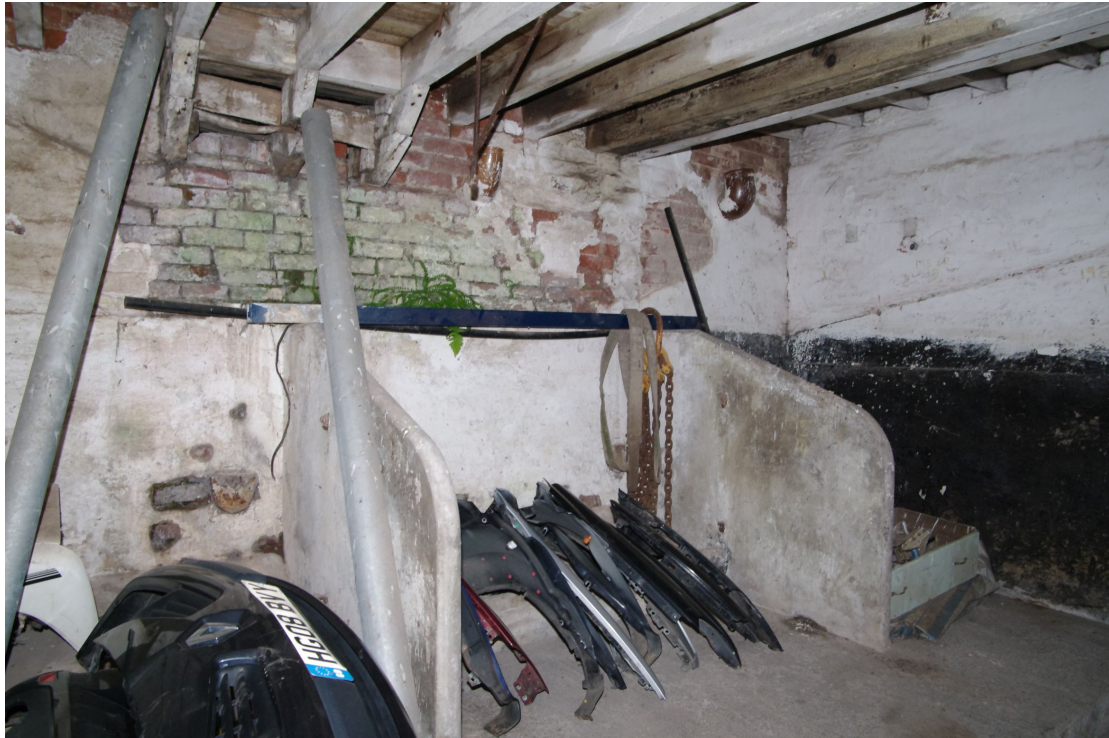
Figure 37 Ground floor of extended hayloft section of Barn 2 range Looking north-east. The change in floor joists at the far right may indicate where the former staircase was located
