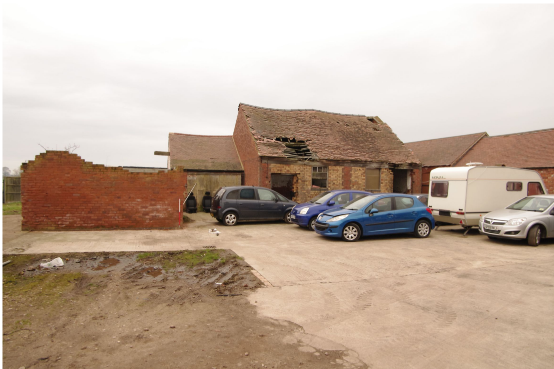
Figure 38 East facing elevation of Barn 3 range Looking north-east. The roofless milking parlour is on the left, extension building and cart shed to the right of this. Barn 2 range on right behind the caravan
