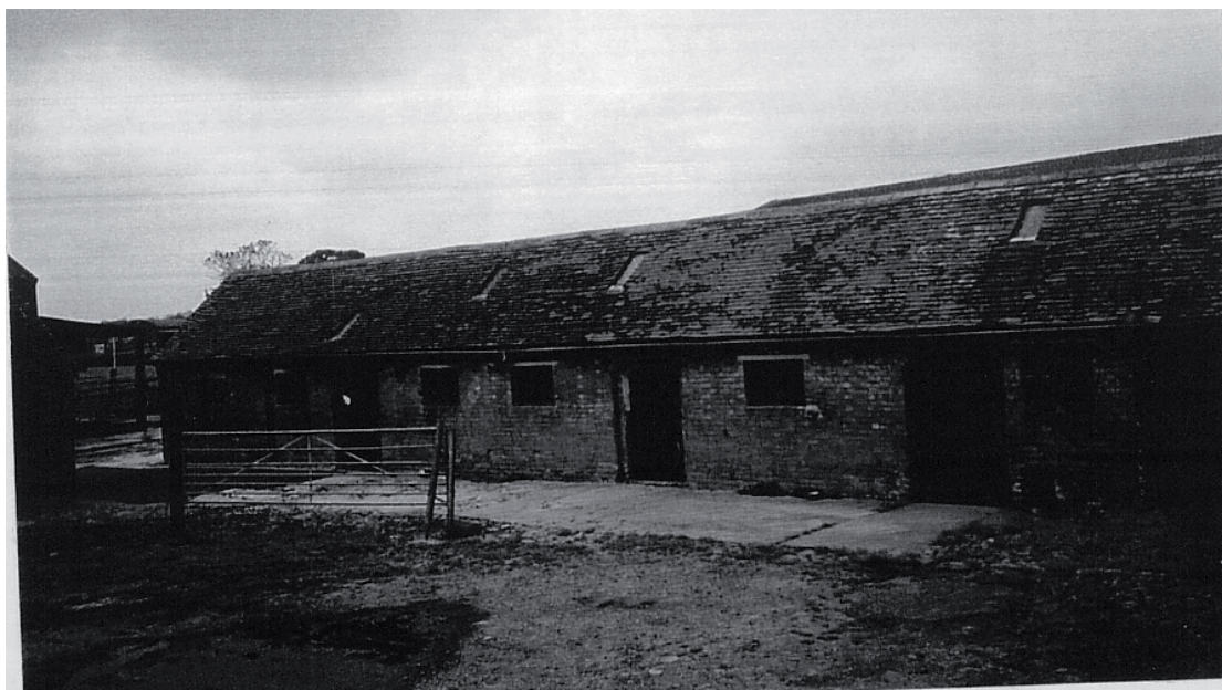
Plate 8 North Range- Milking Parlour- shows earlier form of roof lights set into tiled roof. Original window surviving on right-hand side of view all doorways are rebated with bull-nosed bricks.
