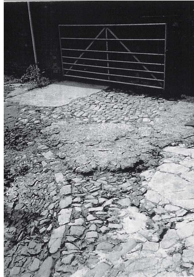
Plate 10 Detail of ranged cobbling partly using granite wasters with some dressed cobbles in Courtyard area. Areas of concrete appear to cover the traditional roundstone cobbles.
