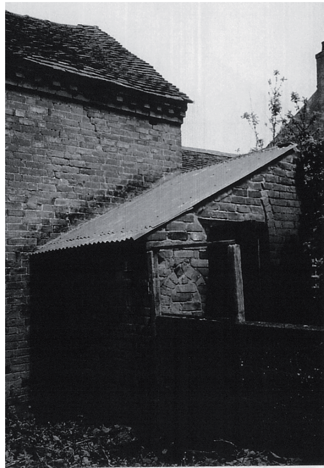
Plate 4 Lean to I, privy on south elevation of south range, shows Gothic window detail and part of doorway arch.
