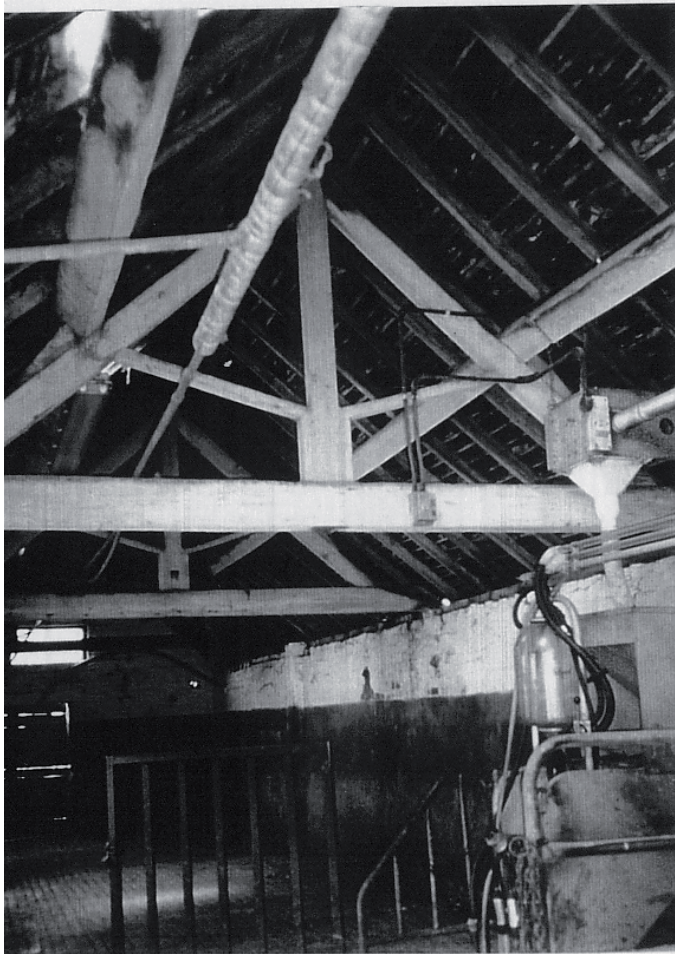
Plate 9 Milking Parlour-North Range-truss detail. A similar Truss is used in the single storey building of the West range.
