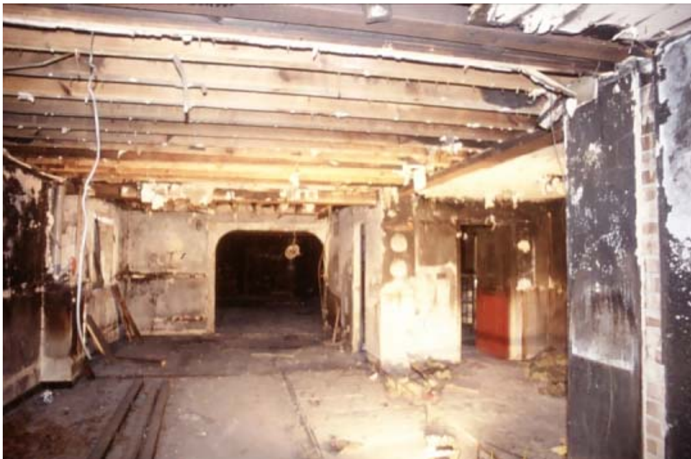
Colour Plate 2 Extent of Damage, Ground Floor.
