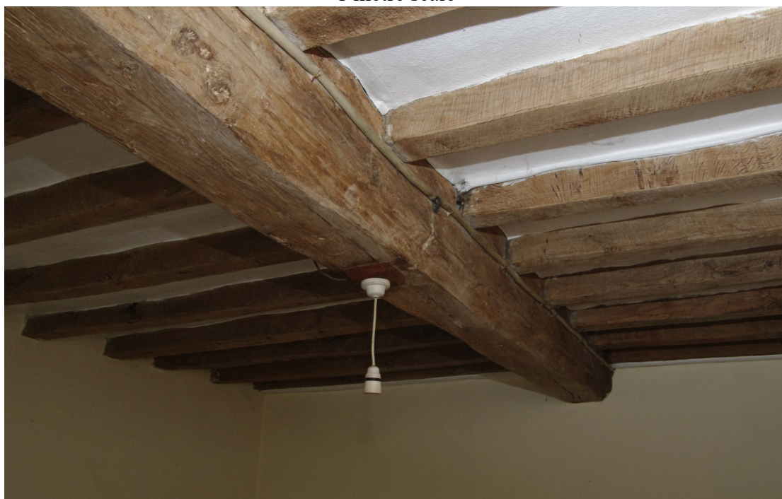
Figure 47 Beam detail Room G5 Nails on the underside of the joists suggest that they were originally hidden
