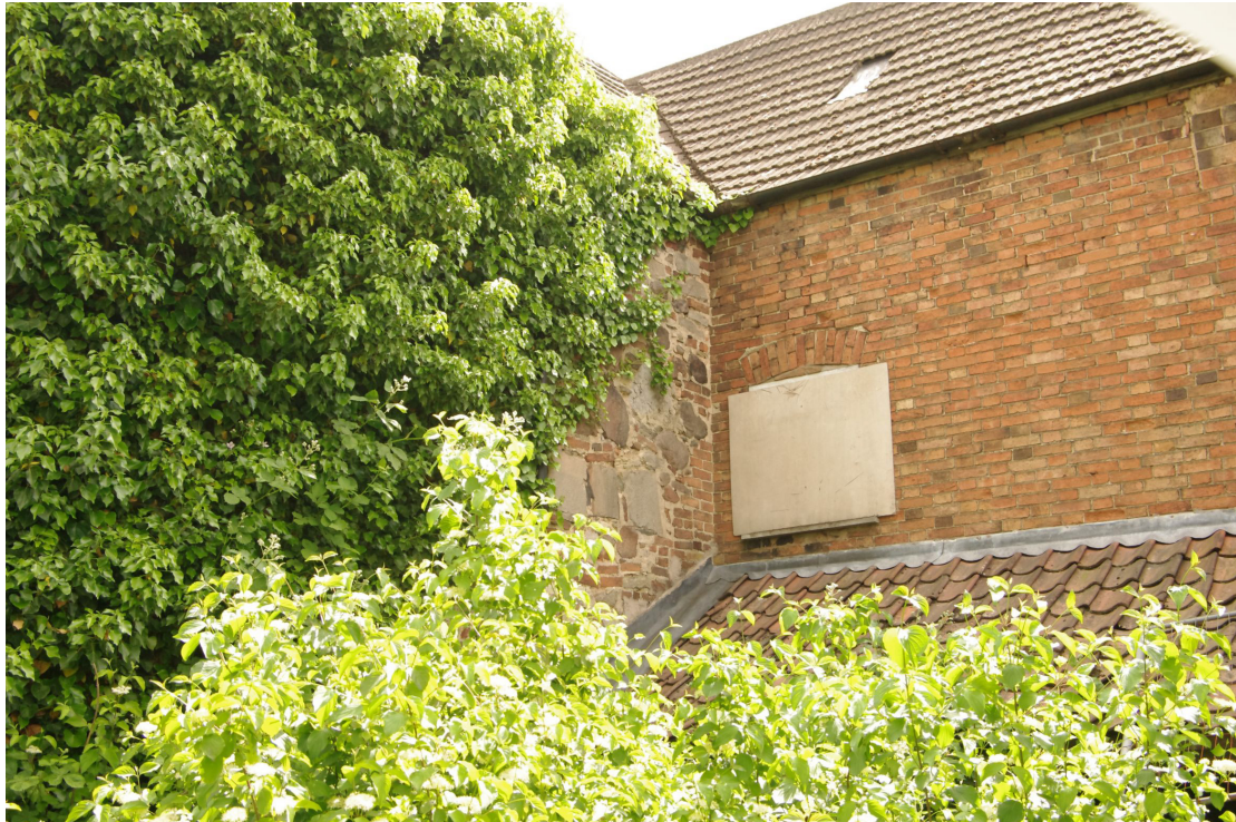
Figure 26 SW facing elevation of rear range and NW facing elevation of 18th century range
