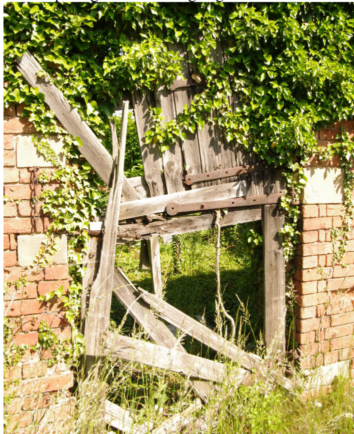
Figure 95 Barn 2 door detail on south-east facing elevation Stable type doors with limestone inserts to support the hinges and fittings
