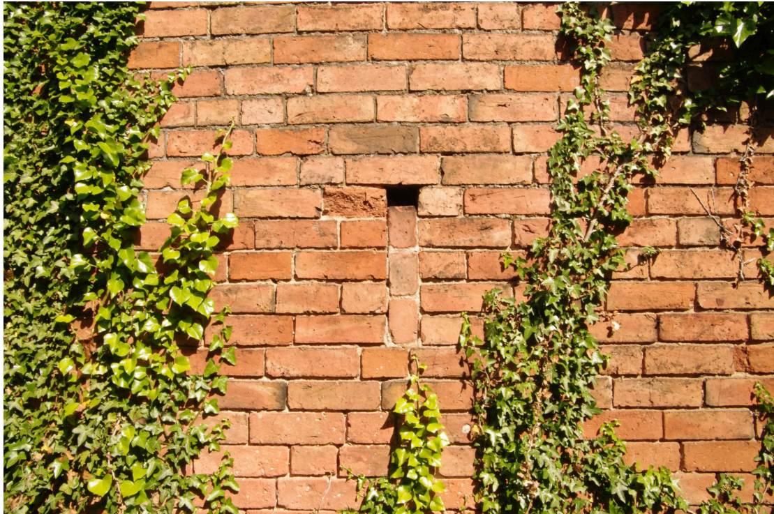
Figure 96 Barn 2, south-east facing elevation blocked ventilation slit Looking north-west
