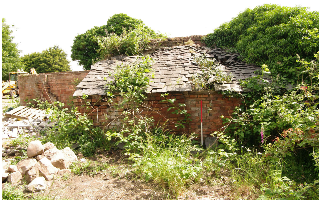
Figure 101 Outbuilding 1, south-west facing elevation Looking north-east. The roof uses graded slates which have been drilled suggesting a 19th century date
