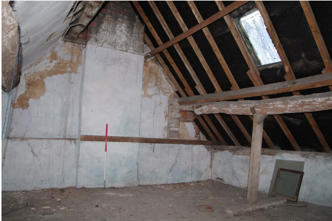
Figure 74 General view of Room S3 Looking west. Note supported purlin and the two later replacement purlins and rafters probably added in the later 20th century. 1m scale
