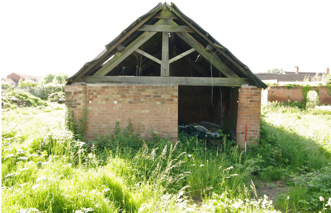
Figure 88 Barn 1, north-west facing elevation Looking south-east. The bolted roof structure suggests a later 19th century date although the purlins inside are re-used and earlier. Barn 2 to right.
