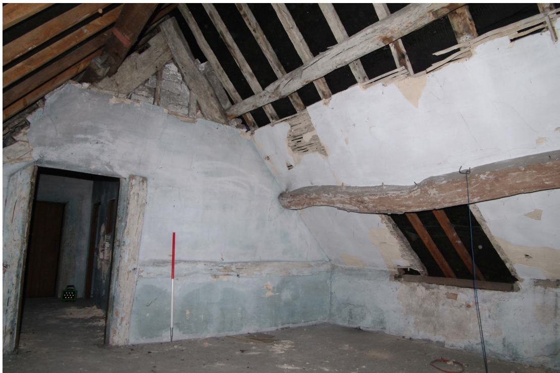
Figure 75 General view of Room S3 Looking east. Doorway leads to Room S2. Both purlins and the rafters survive on this side of the roof. The lower purlin has begun to split and has had a plate bolted to it. Pegged roof truss with redundant sockets on the left side. 1m scale
