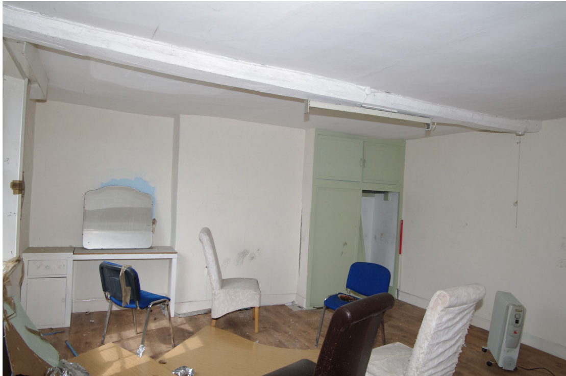
Figure 56 General view of Room F2 Looking west. The beam in this room has a rudimentary chamfer. 1m scale
