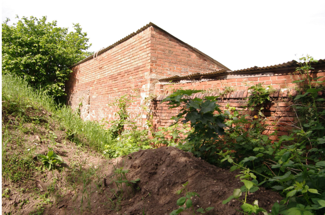
Figure 105 Boundary wall close to north-western corner of the site Looking west. Note the area of stone towards the left of the picture which has been incorporated into the building. The capped brick wall runs towards Outbuilding 2 (see Fig. 103 above)
