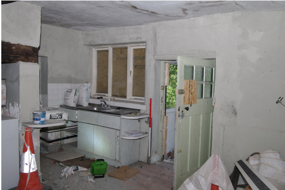
Figure 32 General view of Room G1 Looking north towards outside door. 1m scale
