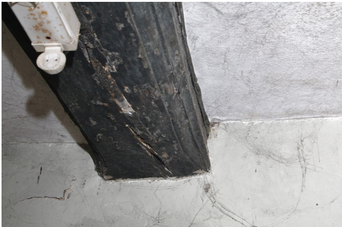
Figure 35 Room G1 beam detail at south-east end The chamfer appears to end in a stop-chamfer at the wall suggesting that it was once a longer beam cut to fit this room
