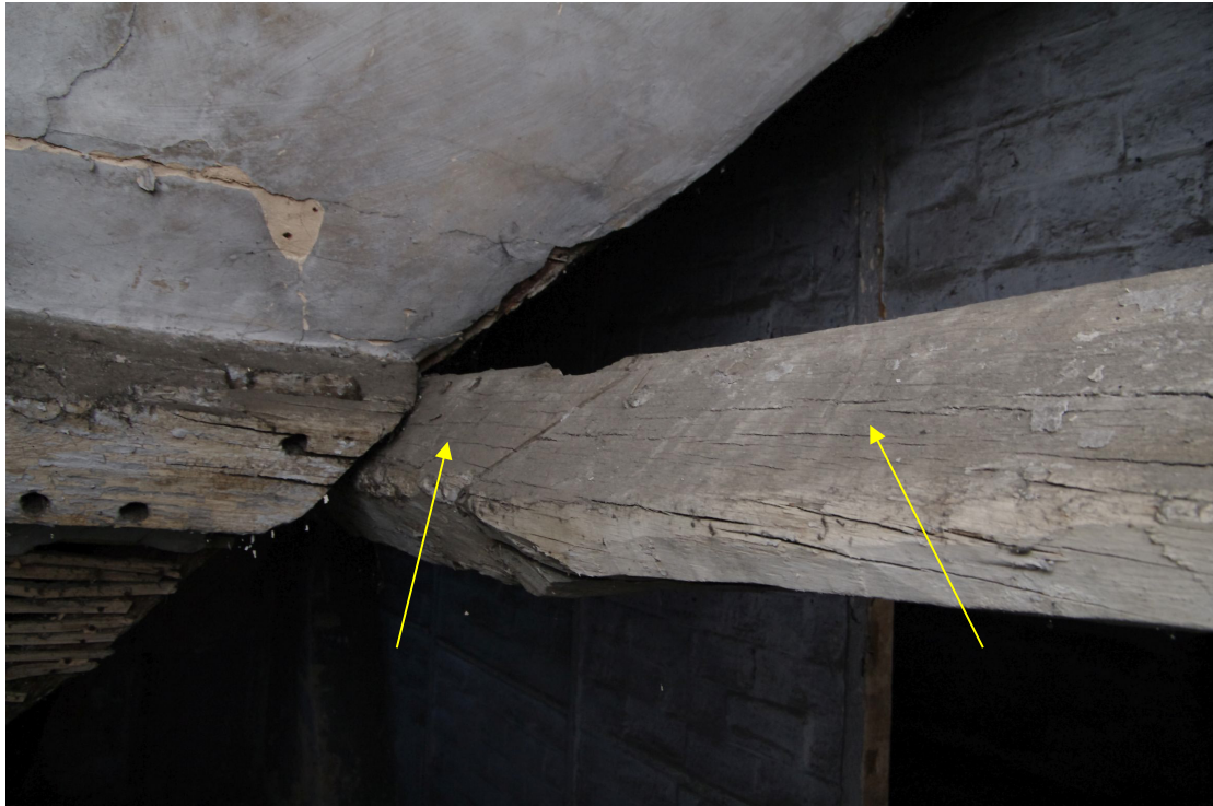
Figure 82 Redundant peg holes and carpenter's marks, Room S5 Looking south-east. The carpenter's marks are seen as Roman numerals II and are highlighted with the arrows
