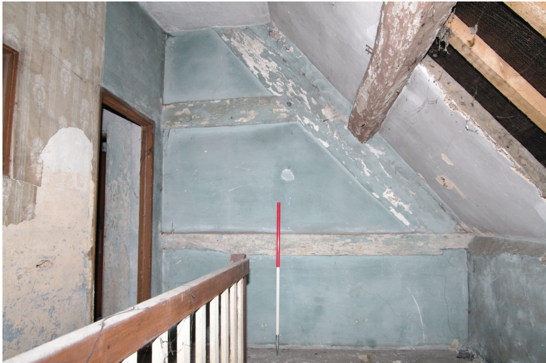
Figure 68 General view of Room S1 Looking north-east. Door on left leads to S2. 1m scale
