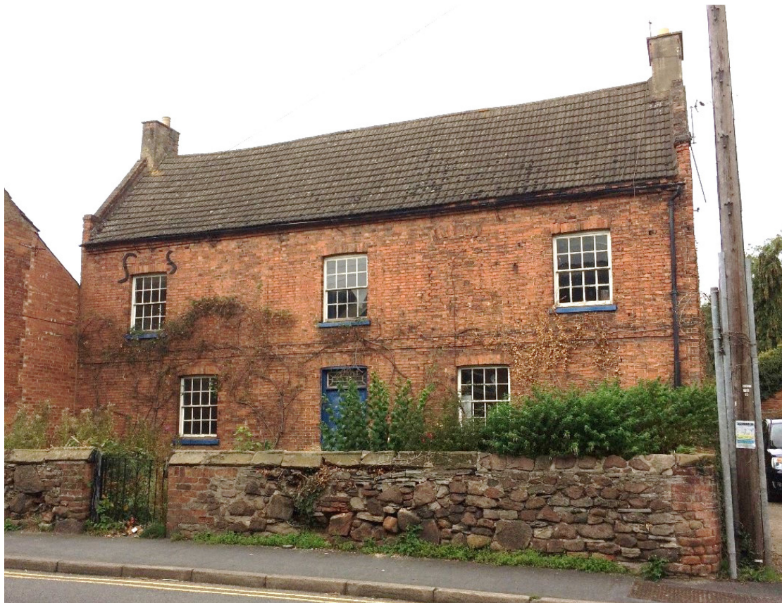
Figure 10 South-east facing elevation of farmhouse Picture source: Lanpro Services DBA 2017. Photograph taken before erection of hoardings and demolition of boundary wall
