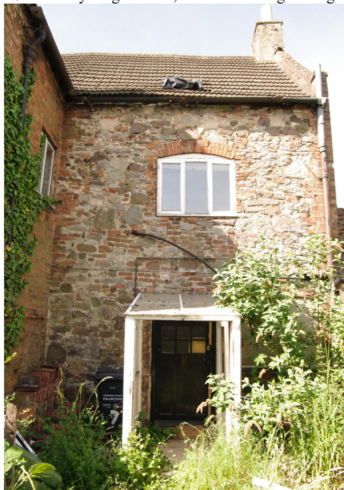
Figure 21 North-east facing elevation of rear range Note rather haphazard use of uncoursed stones and brick infilling
