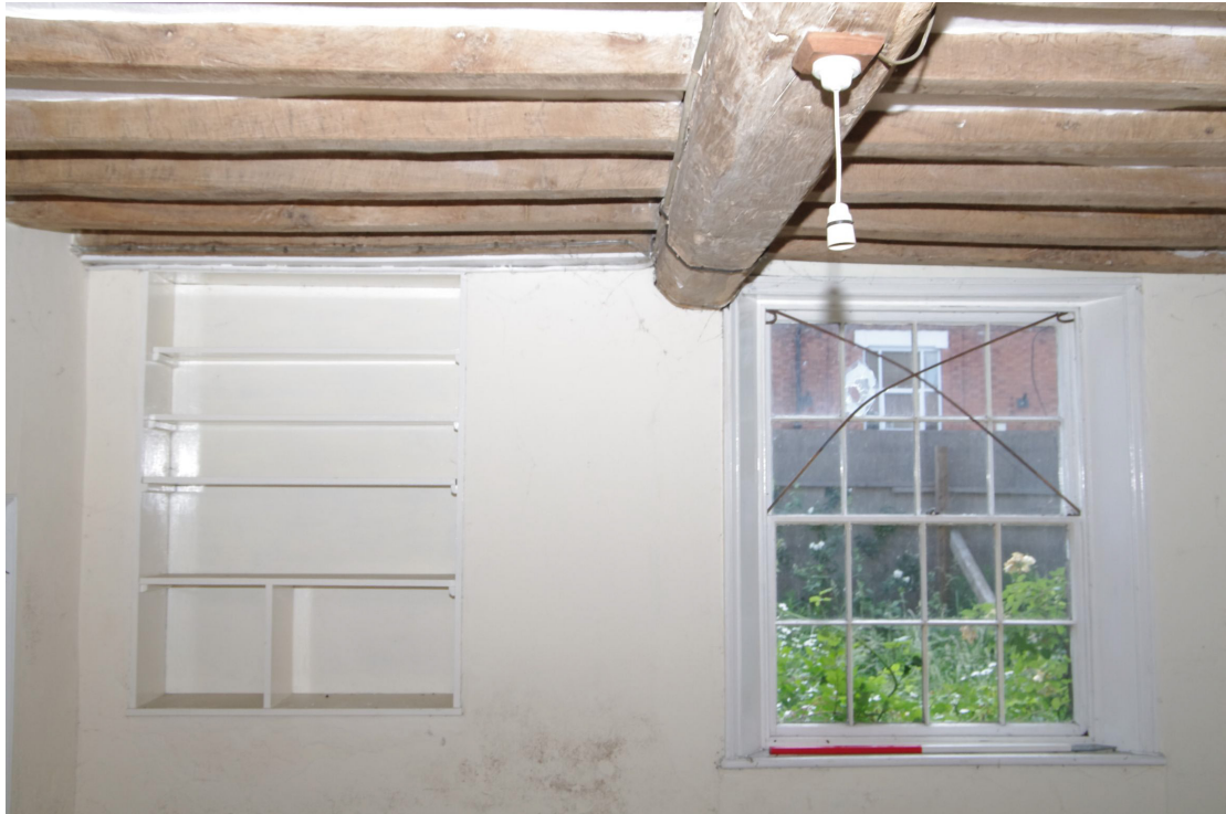
Figure 44 South-east wall and window detail of Room G5 Looking south-east. Note earlier and smaller blocked window on right adapted to be used as shelving. The later windows are splayed whilst the earlier blocked ones are not. 1m scale
