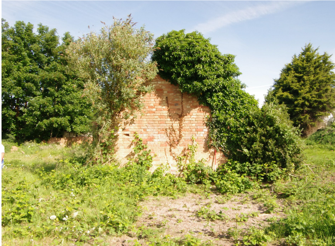
Figure 86 Barn 1, south-east facing gable end Looking north-west. The OS maps show this gable continuing south-eastwards to join the courtyard barns. 1m scale
