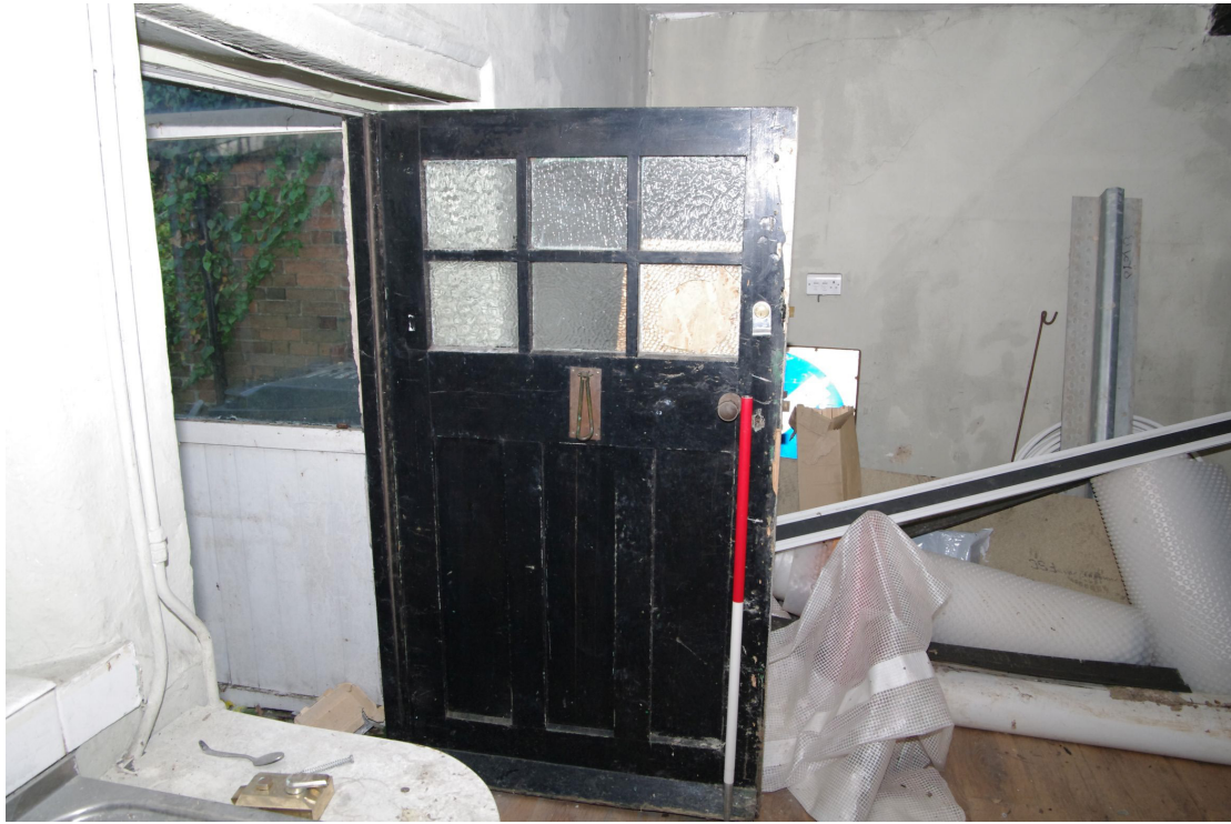
Figure 30 Door detail of rear range door into G1 Note that the earlier staircase was located in the corner behind the door
