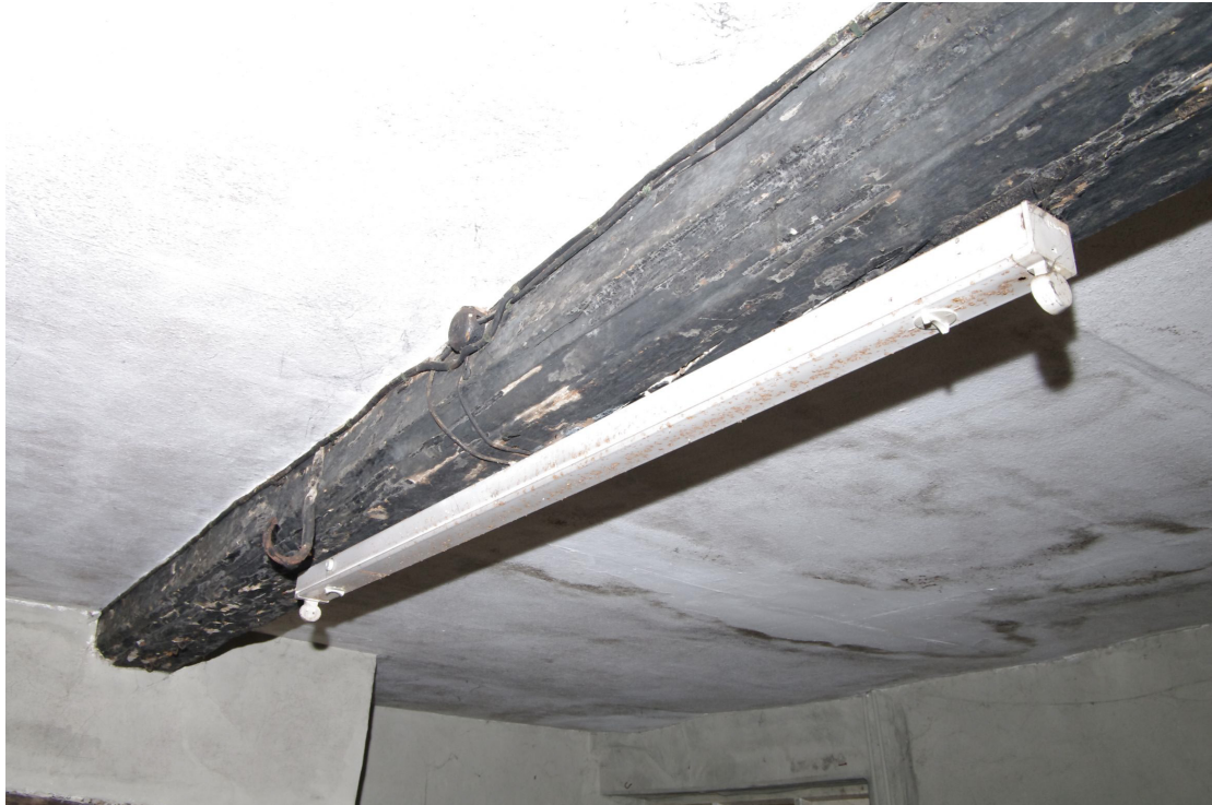
Figure 34 Room G1 beam detail Looking north. Note hook, also that the chamfer continues into the wall above the fireplace
