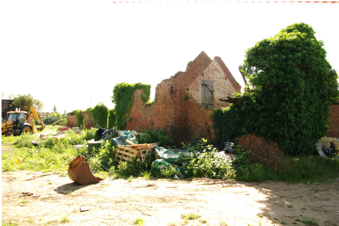
Figure 92 Barn 2, north-west facing elevation Looking east towards the two-storey section of the barn
