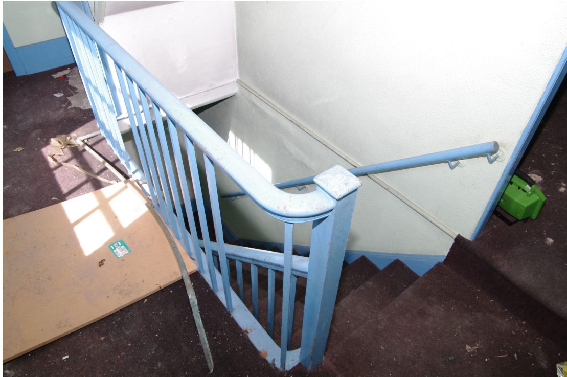
Figure 52 Stairs from ground floor G4 up to first floor F1 Looking west. Doorway to F5 and rear range on right
