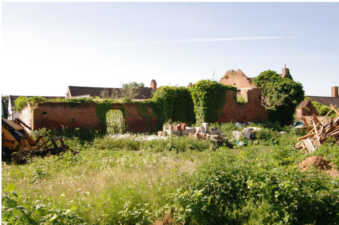
Figure 91 Barn 2, north-west facing elevation Looking south. Single storey block on left, two storey on right. The roof of the modern garage can be seen above the arched doorway centre left. Farmhouse rear range chimney above ivy on right
