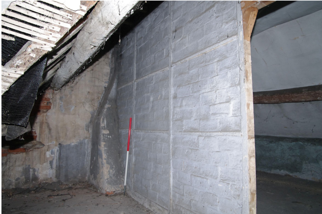
Figure 80 Partition wall between S5 and S4 Looking east at the oversized brick and timber wall. Doorway to S4 on right. 1m scale
