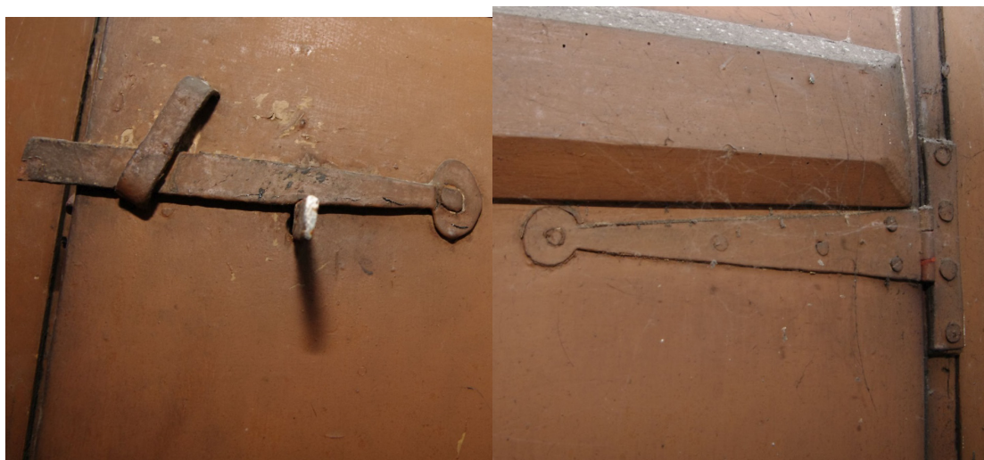
Figure 73 Handmade fittings of door between S2 and S4
