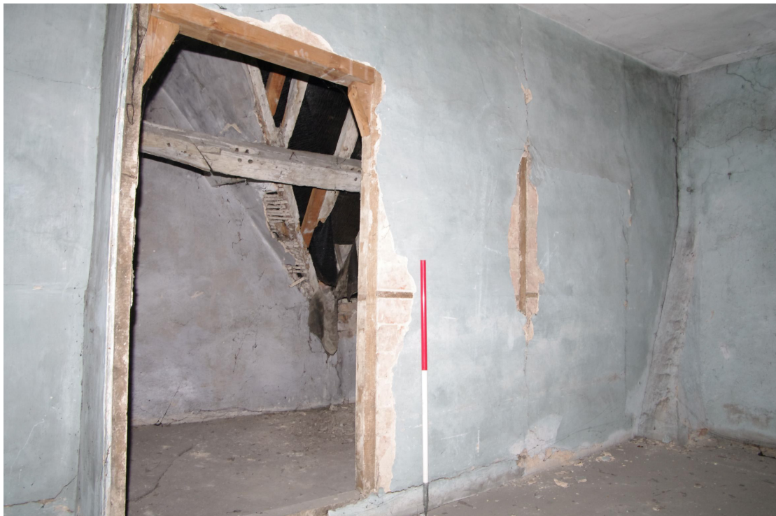
Figure 79 Partition wall between S4 and S5 Looking north from Room S4. The oversized bricks are set within a timber framework made of thin battens. 1m scale
