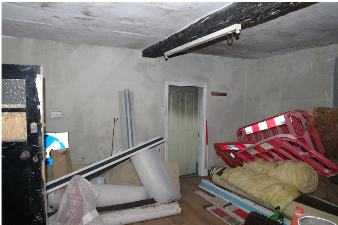
Figure 31 General view of Room G1 Looking south towards doorway to G2 and 18th century range. A blocked doorway from G8 is in the corner behind the safety barriers although no trace is visible here
