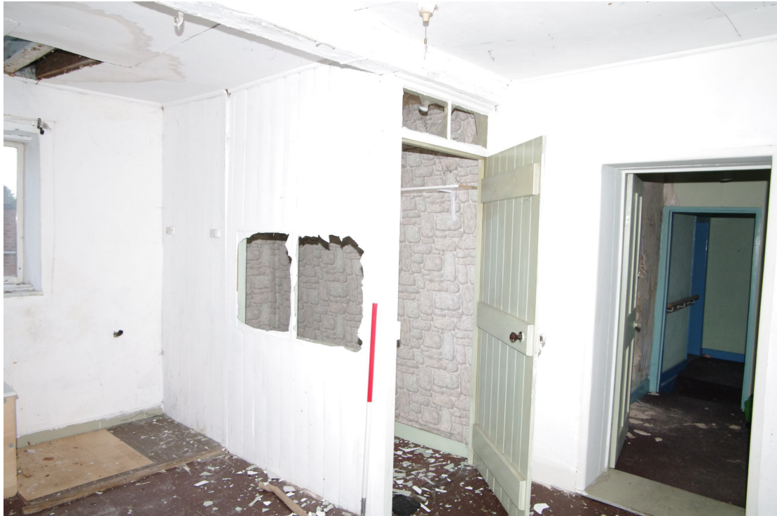
Figure 64 Room F6 and enclosed staircase partition The stairs are no longer present. Doorway to Room F4 on right
