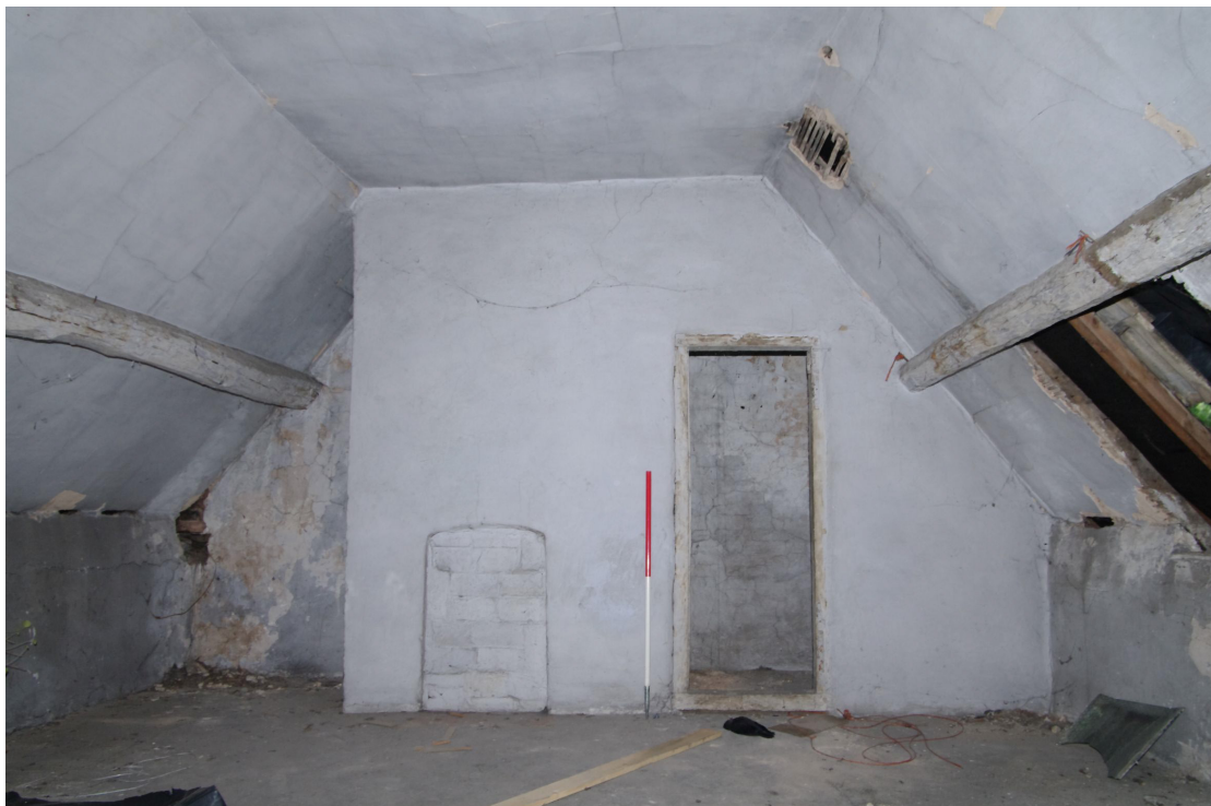
Figure 83 General view of Room S6 Looking north-west. The doorway to the right of the 1m scale leads into a large cupboard space
