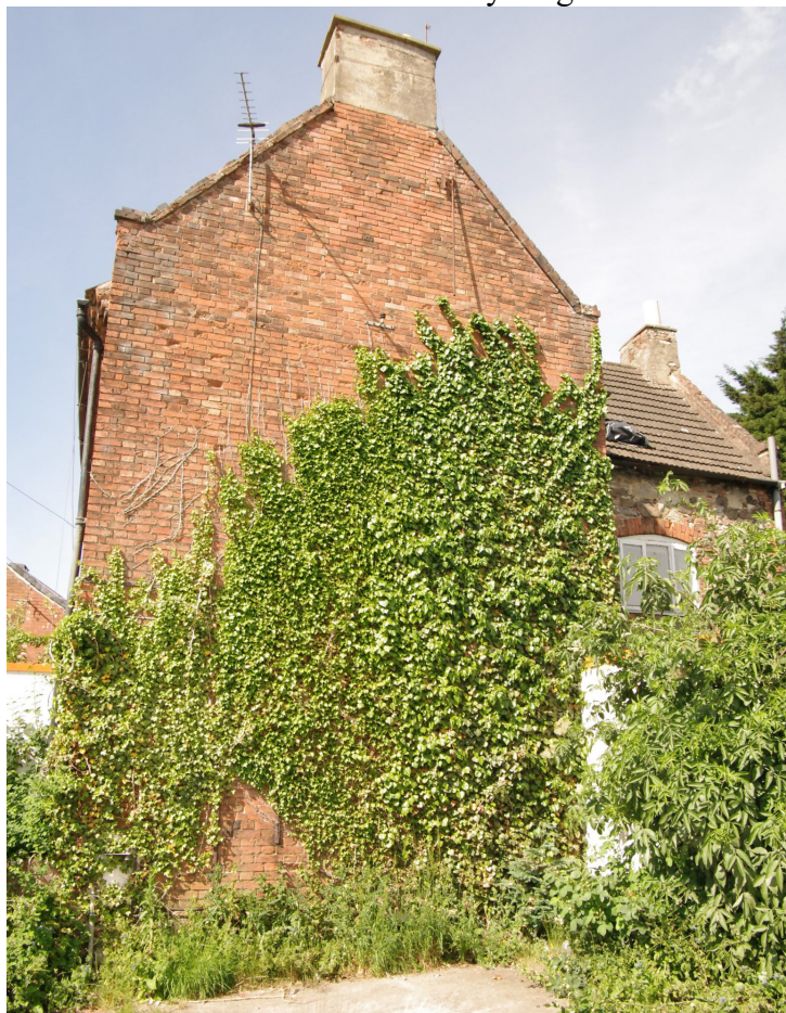
Figure 19 North-east facing gable end of 18th century range Looking south-west. Earlier stone-built range on right
