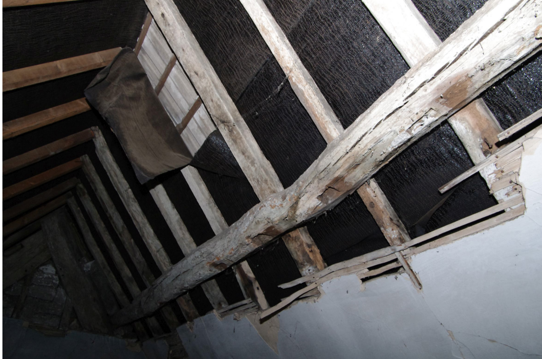
Figure 76 Room S3 upper purlin detail on SE side of roof This is a re-used timber with many redundant sockets. Looking east
