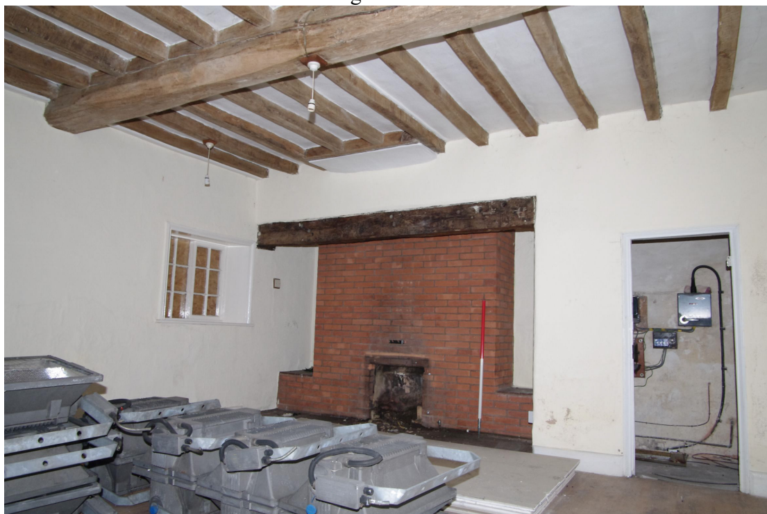
Figure 43 General view of Room G5 Looking north-east. The fireplace brickwork is fairly modern. 1m scale
