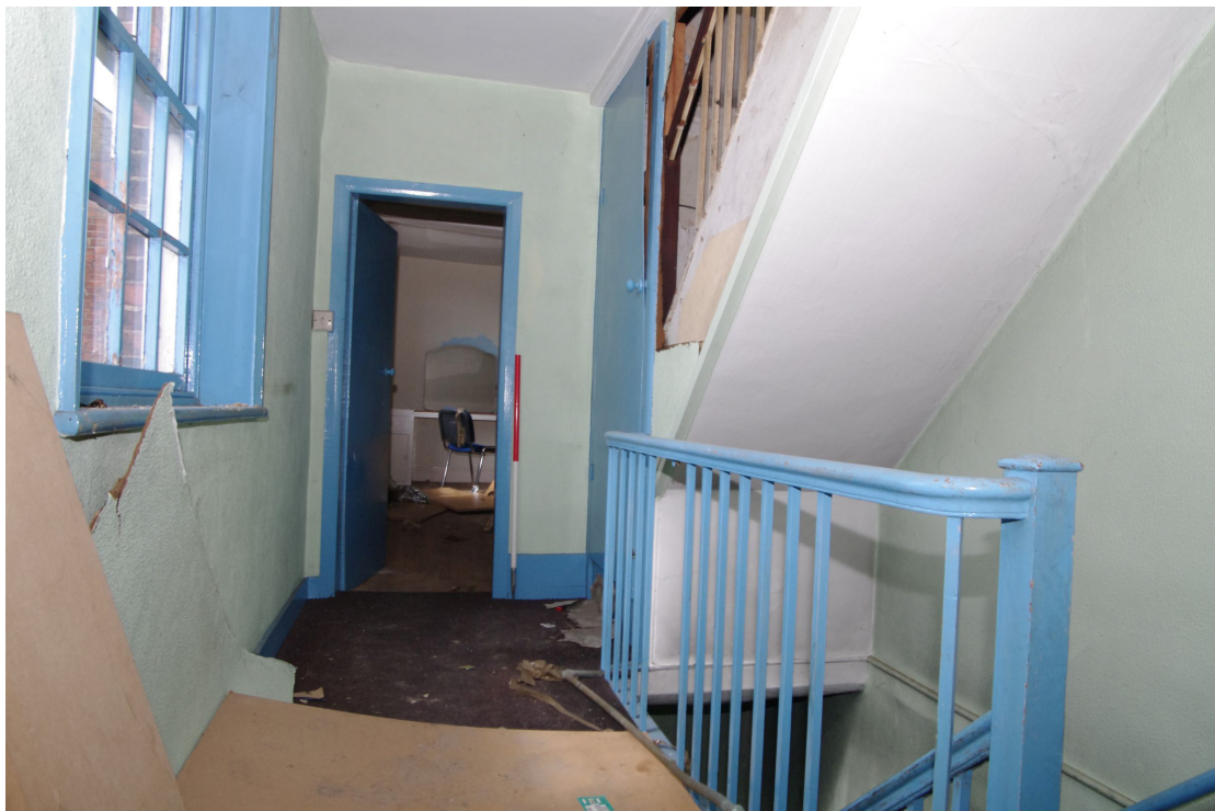
Figure 53 Room F1 Looking south-west towards Room F2. Note stairs to second floor servant's quarters to right of 1m scale
