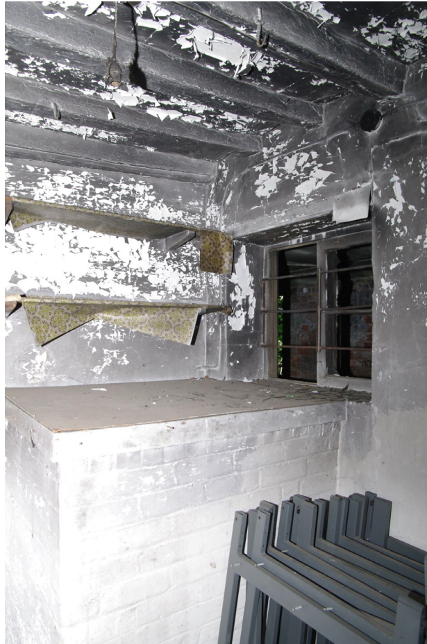
Figure 40 Room G3 Looking north. The brick base forms the roof of the cellar stairs
