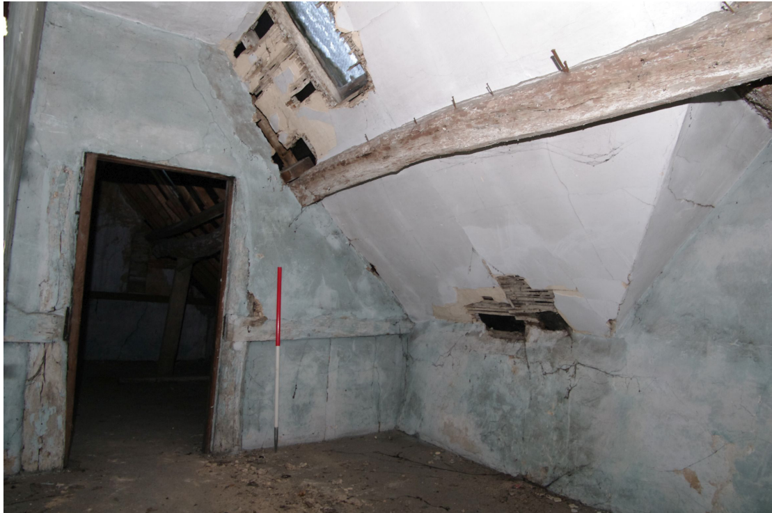
Figure 70 General view of Room S2 Looking west. Doorway leads to Room S3
