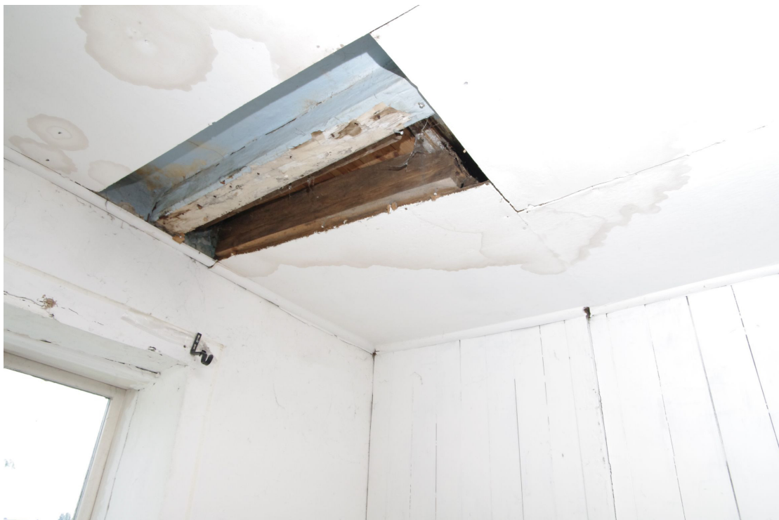
Figure 65 Room F6 ceiling and former staircase scar Modern ceiling covering masks the original location of the stairs which had a dogleg
