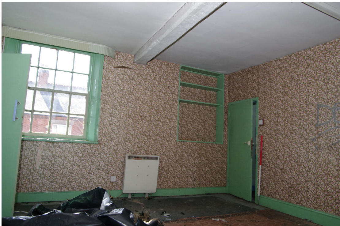
Figure 57 General view of Room F3 Looking south-west. Door on right leads to landing Room F1. Note smaller blocked window used for shelving to left of doorway
