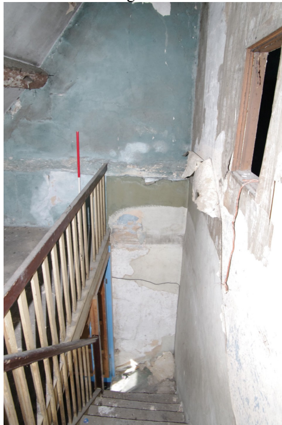
Figure 67 View down stairs to first floor from Room S1 Looking south-west. Note window on right wall to allow light into the adjacent room
