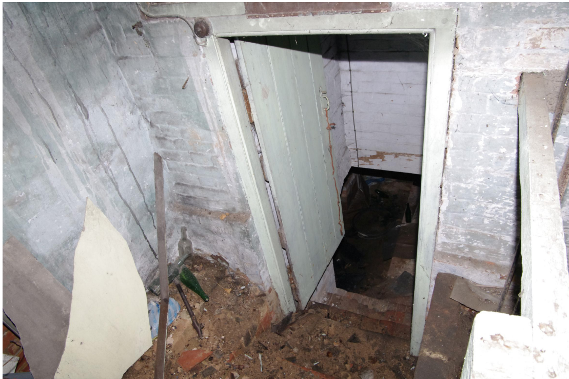
Figure 28 Cellar steps from lean-to extension at the rear Looking south-east. The cellar sits below the 18th century range
