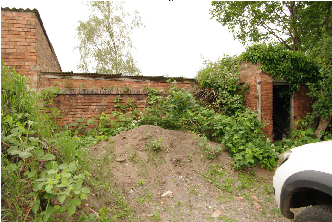
Figure 103 Outbuilding 2 Looking north. The building forms a small rectangular structure located in an angle in the boundary wall which is brick-built at this point (see following figures)
