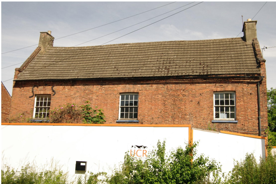
Figure 15 South-east facing elevation first floor detail Looking north-west. Note earlier and smaller infilled windows either side of the central window. The cement tiles are likely to be 1950s or later
