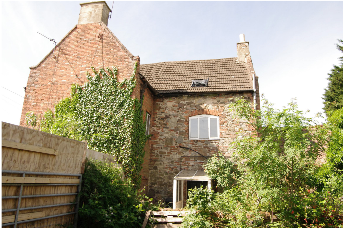
Figure 20 North-east facing elevation 18th century range on left, earlier rear range on right
