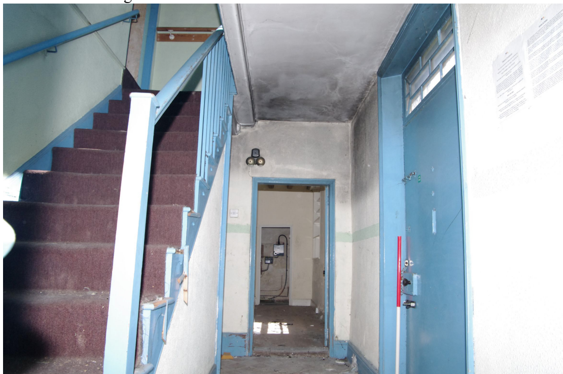
Figure 41 Hallway G4 Looking north-east. Front door on right. Room G5 ahead and corridor G2 left beyond the stairs
