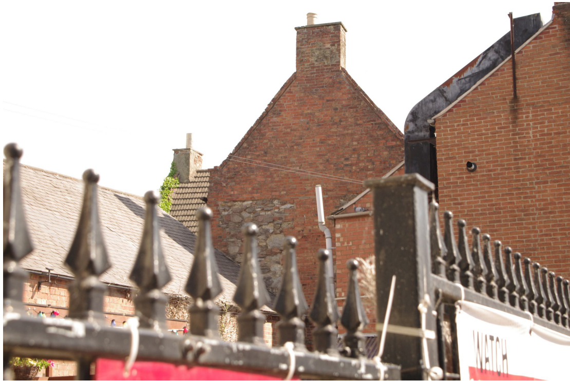
Figure 18 South-west facing gable end seen from King Street The rectangle of stonework suggests that part of an earlier range was incorporated into the 18th century range
