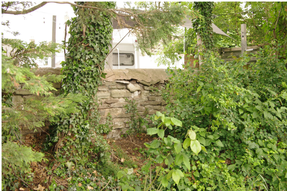
Figure 104 Boundary wall along west side of site Looking north-west. The wall along this side of the site is a mix of stone and brick
