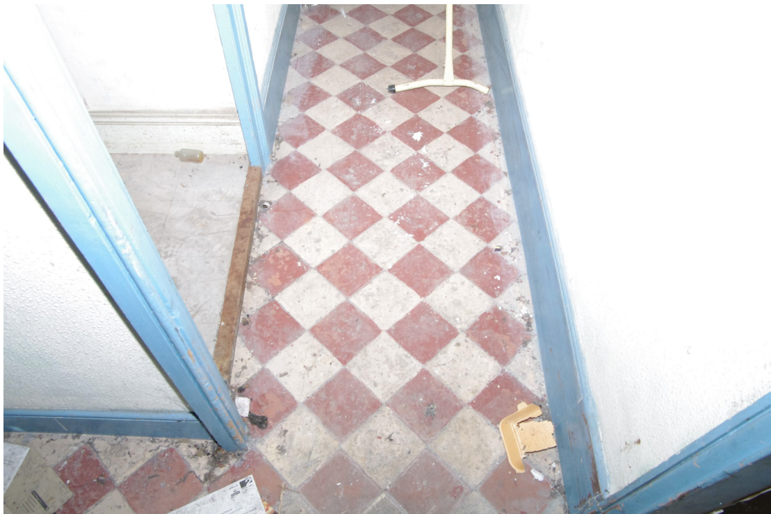
Figure 37 5½ inch square quarry tiles on floor of G2 These tiles continue into hallway G4
