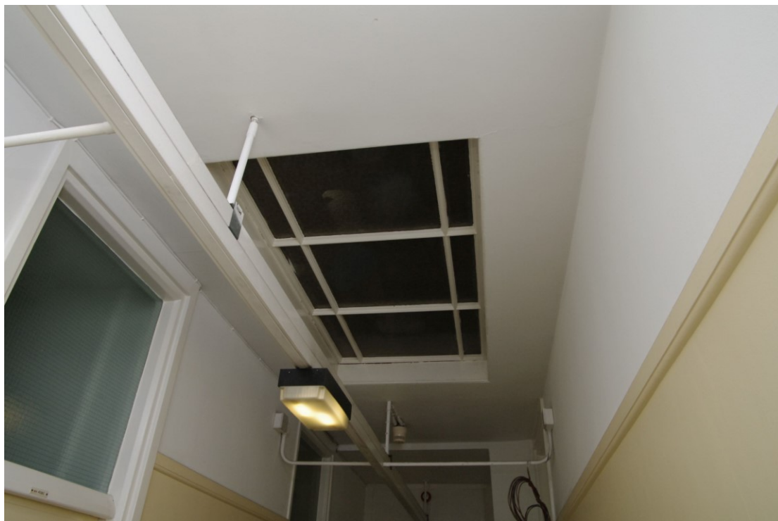
Figure 138 Third floor, later 1930s north to south corridor: skylight Looking north. Also note the narrowing of the corridor to the earlier 1930s phase
