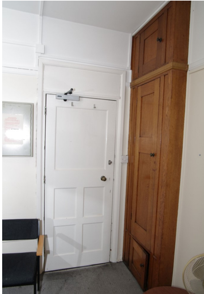
Figure 119 Second floor, 1910 north to south corridor: fitted cupboard Looking west in Room 217
