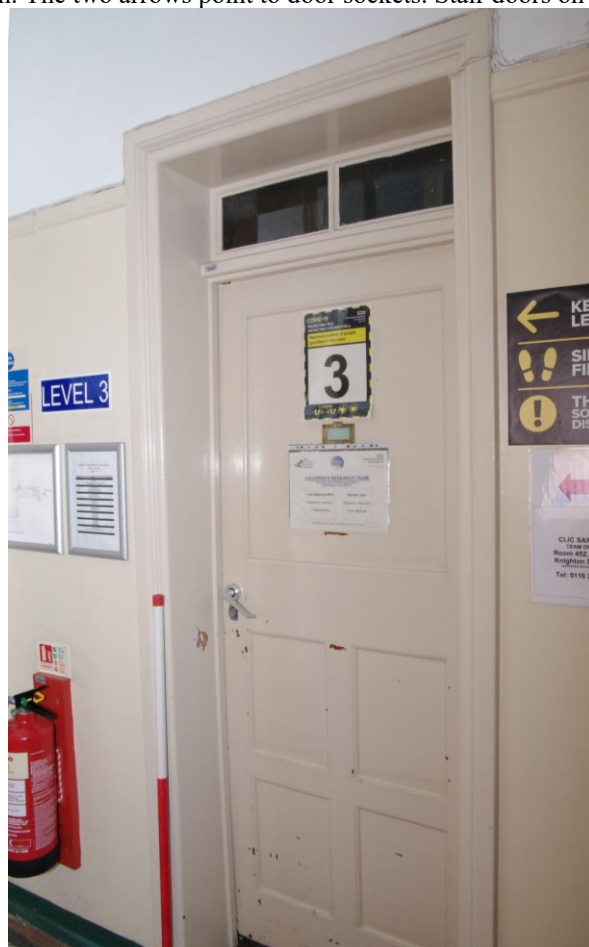
Figure 133 Third floor, 1910 north to south corridor: door detail Looking east at Room 318 (450 on the door plate). 1m scale
