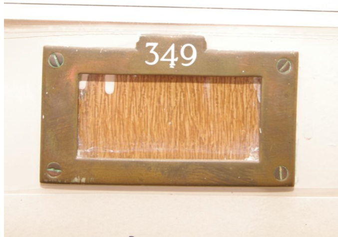
Figure 117 Second floor, 1910 north to south corridor: name and number plate holder Note that this is Room 217 on the estates plan in Fig. 114)
