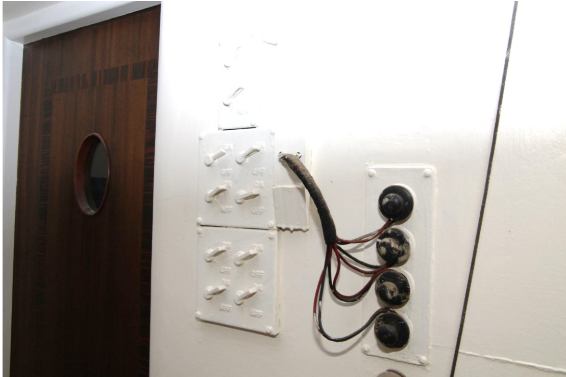
Figure 70 Recreation room/theatre: Stage light switches
