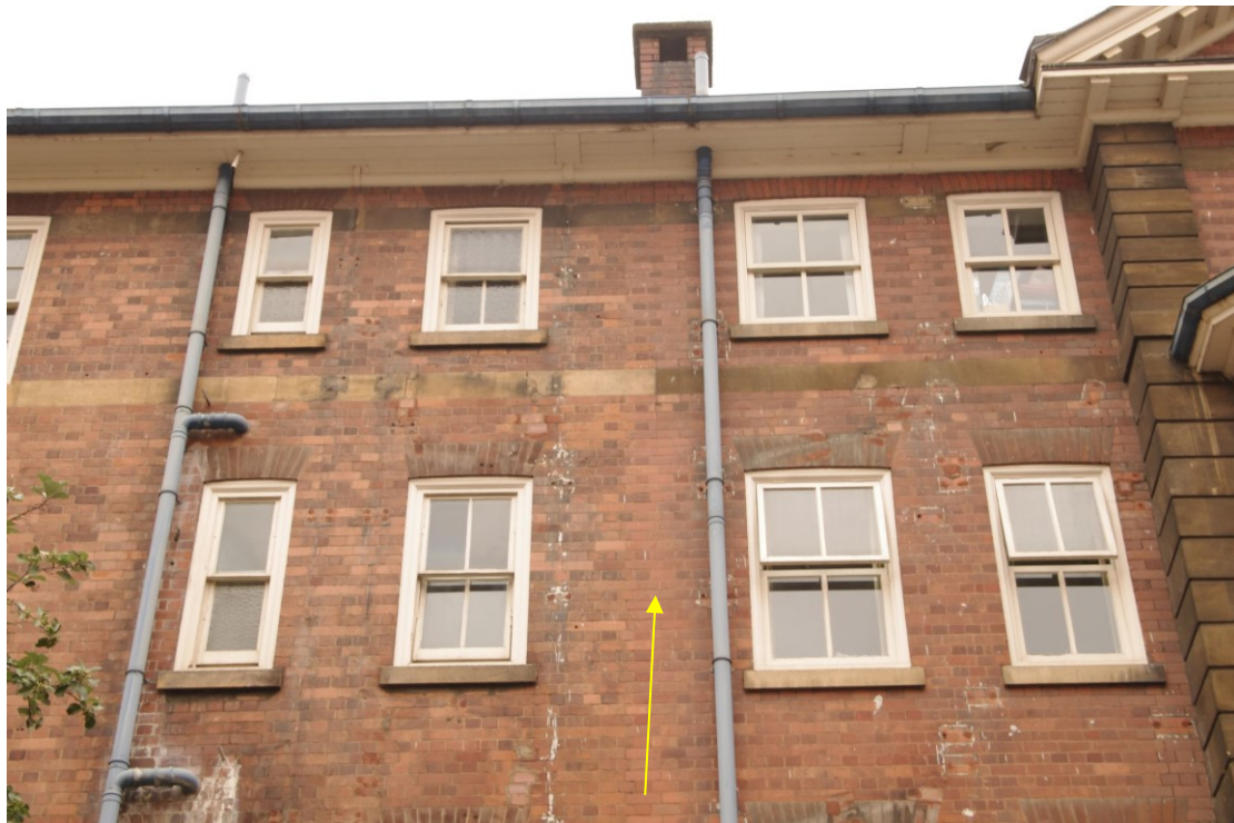
Figure 36 1930s west facing wing, joint between the two phases Looking east. Arrow points to the joint, earliest extension on left
