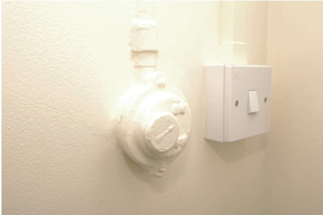
Figure 86 Ground floor: 1930s phase light switch
