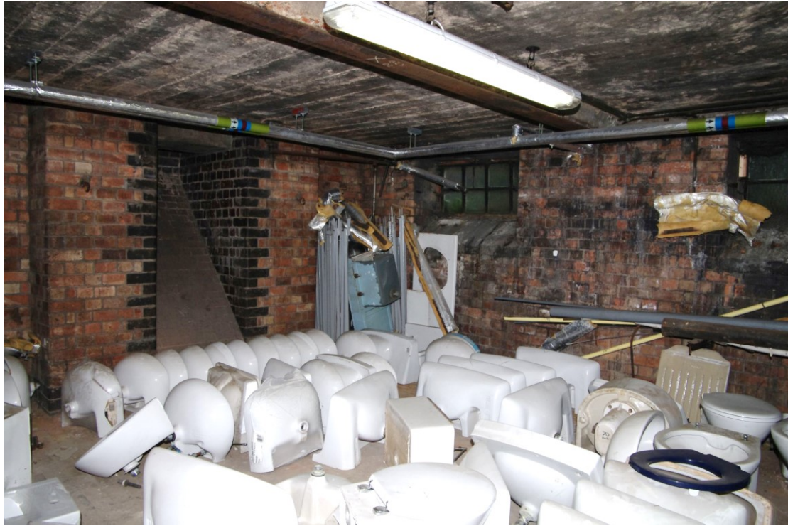
Figure 51 Basement: coal store and former chute Looking south-east. Blocked chute on left hand wall
