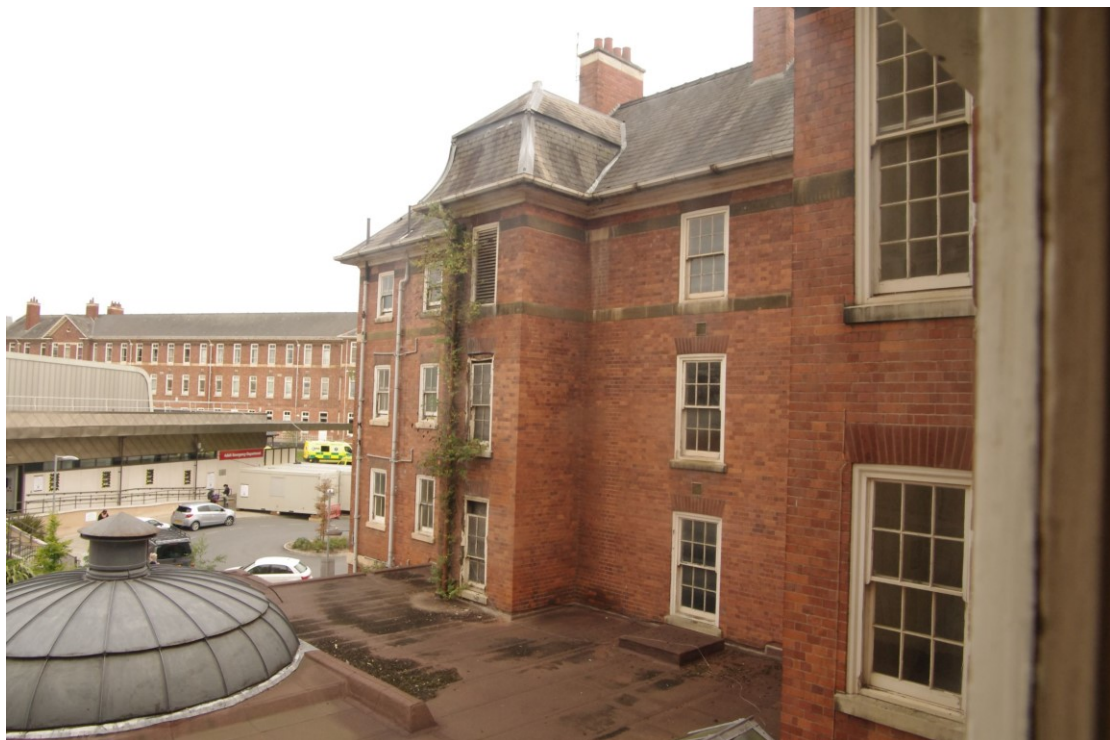
Figure 28 Rear, eastern, wing of the 1910 range Looking north-east. The projection holds a modern lift shaft. Recreation room roof on left
