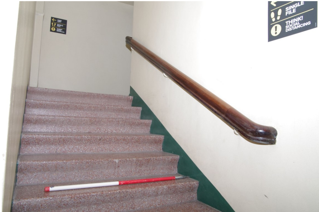
Figure 60 Ground floor: stairs to first floor from the rear east to west corridor Looking south-west. 1m scale
