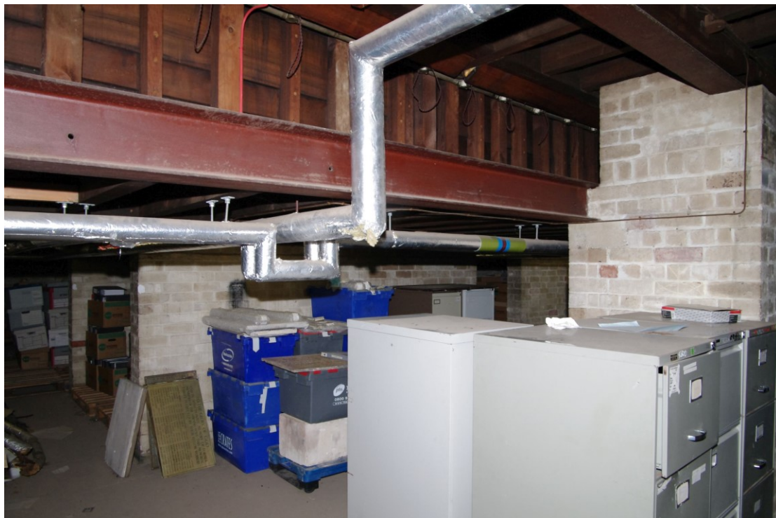
Figure 46 Basement room beneath the theatre Looking north-east. Note the step in the ceiling
