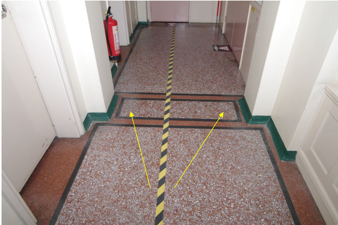
Figure 132 Third floor, 1910 north to south corridor: floor detail by stairs Looking south. The two arrows point to door sockets. Stair doors on right. 1m scale
