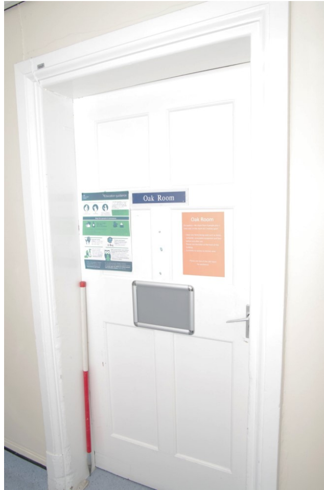
Figure 76 Ground floor, 1910 east to west corridor: door detail Note also the moulded plater skirting detail. 1m scale
