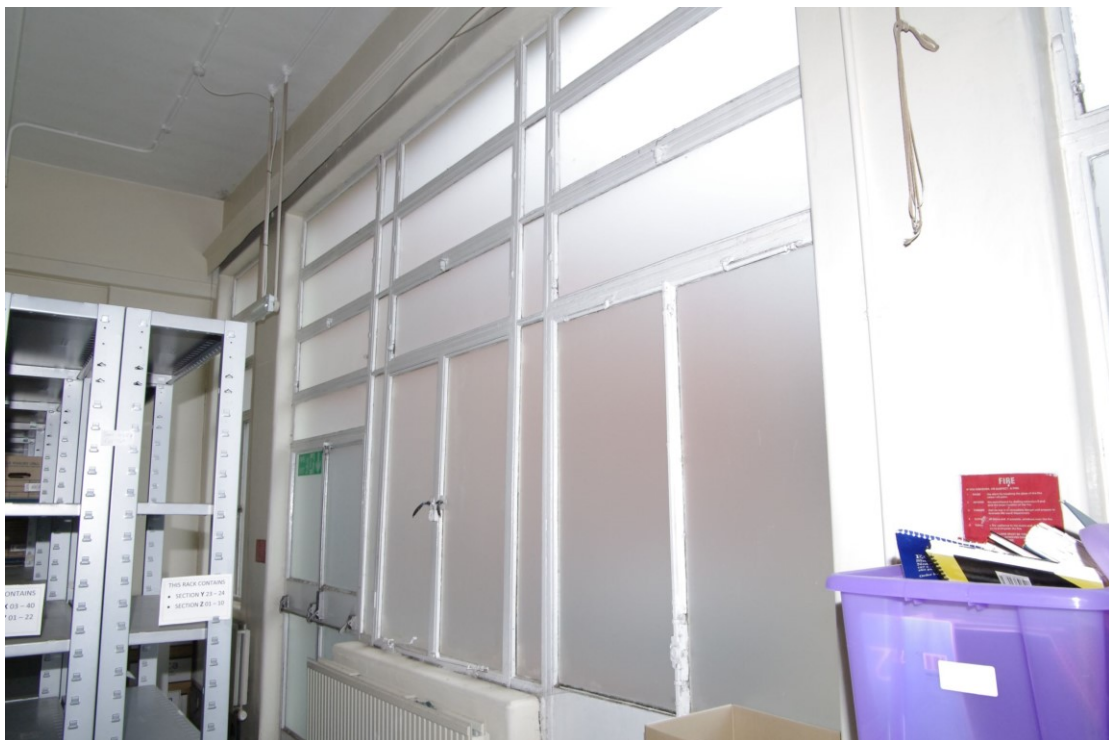
Figure 65 Recreation room/theatre: north wall window detail Looking north-west. Note the pelmet for the missing curtains. The fire doors are modern.
