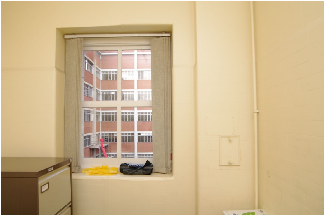
Figure 140 Third floor, earlier 1930s north to south corridor: washroom detail Looking west. Note painted-over bricks
