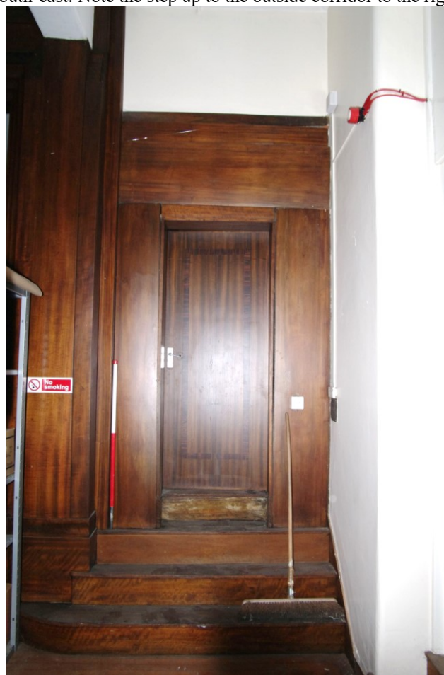
Figure 67 Recreation room/theatre: door to the changing rooms in the wings Looking east at the southern door. 1m scale
