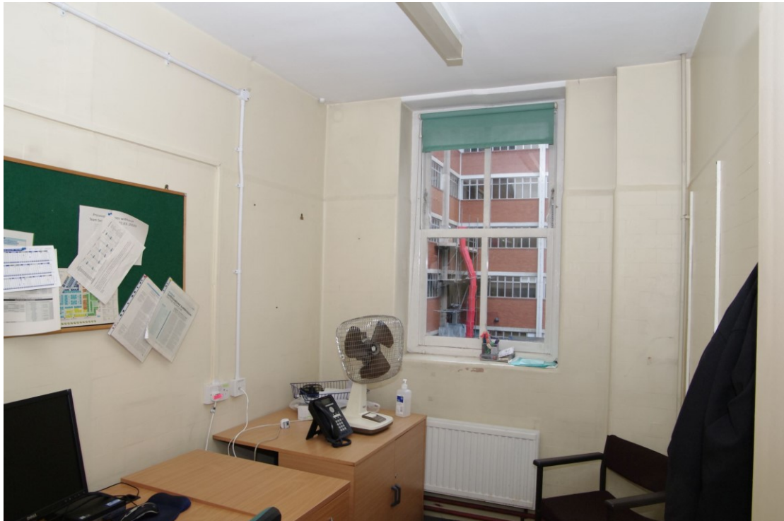
Figure 111 First floor: later 1930s phase, glazed brick lined room Looking west in Room 143. The bricks have been painted over
