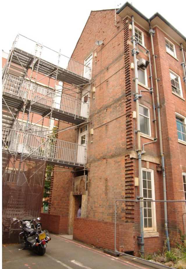
Figure 37 South facing gable end of 1930s wing Looking north-west. Note the alternating projecting brick courses for future keying of new brickwork
