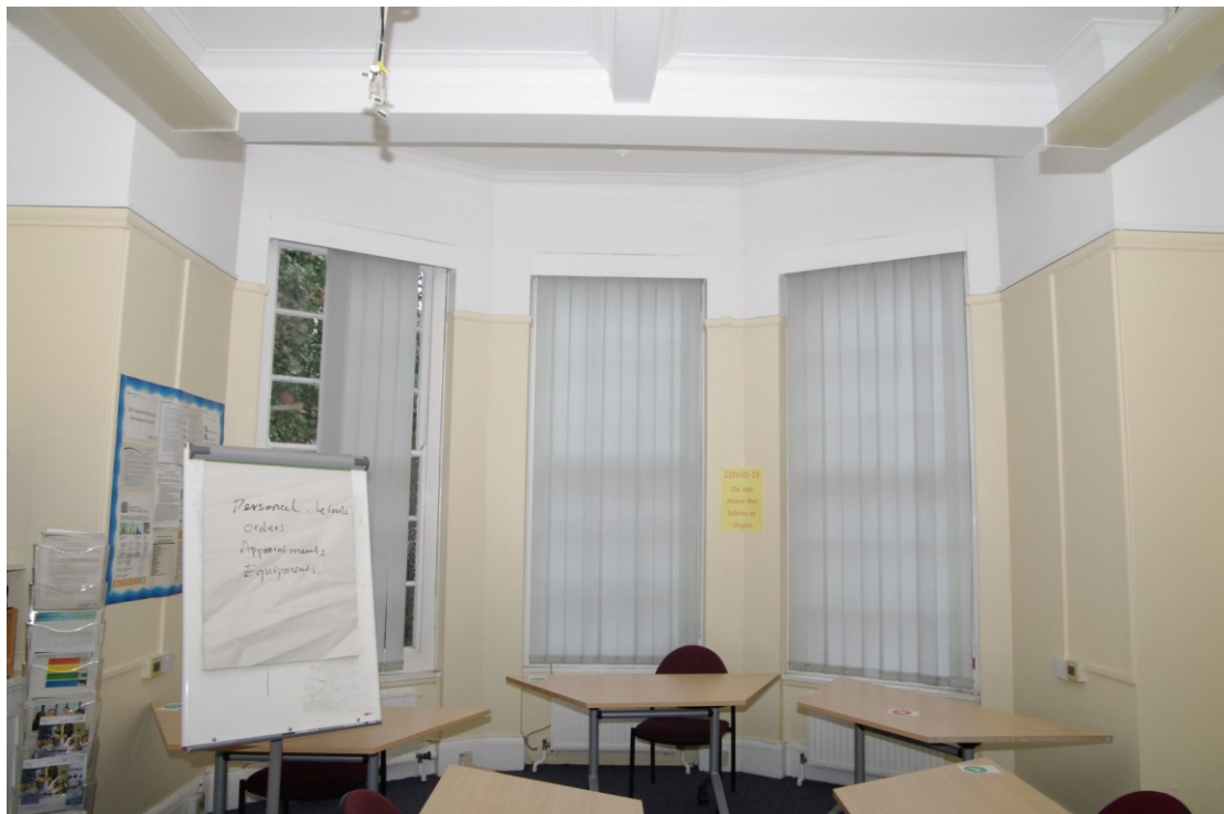
Figure 79 Ground floor, 1910 east to west corridor: Room 047 Bay window detail. Compare with Figure 80
