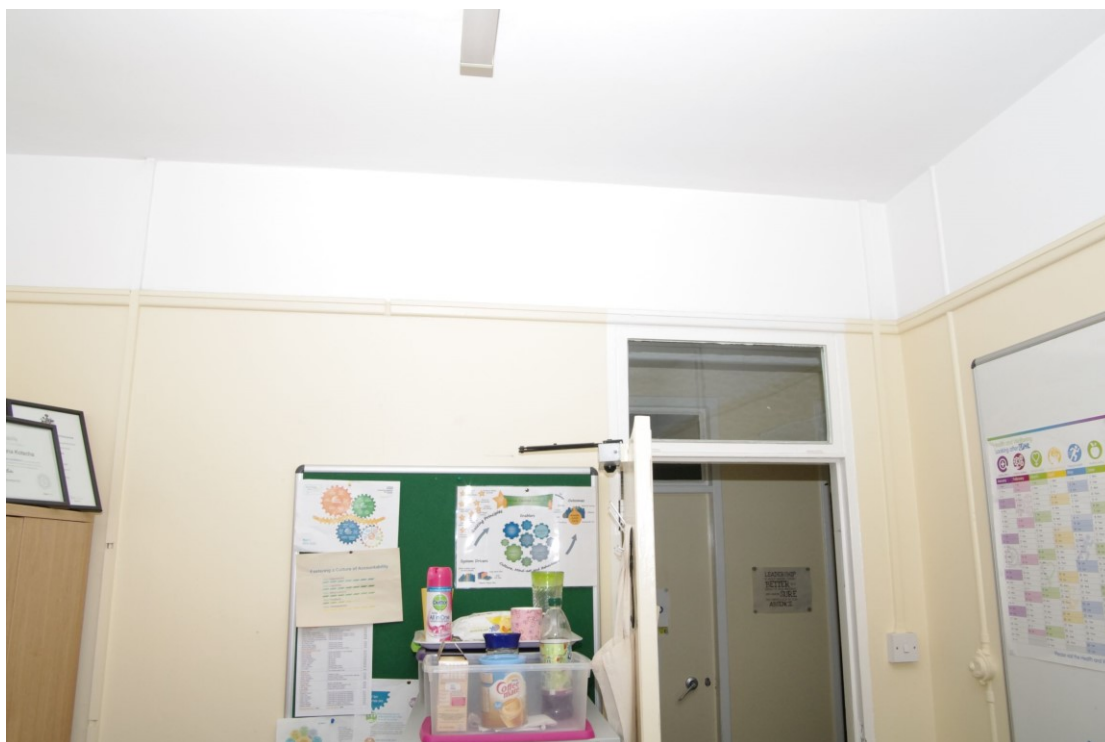
Figure 139 Third floor, earlier 1930s north to south corridor: office detail Looking west in Room 324. Note fanlight still in place and original light switch
