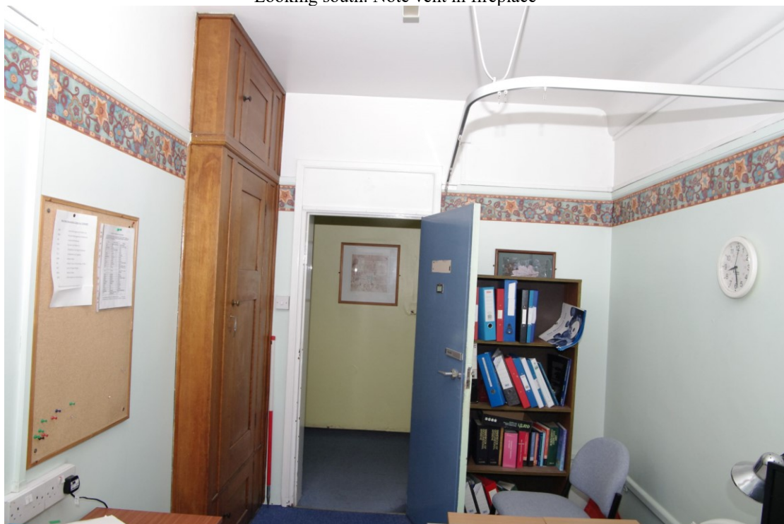
Figure 104 First floor: office on 1910 east to west room Looking north in Room 151. Note curtain rail on right. 1m scale
