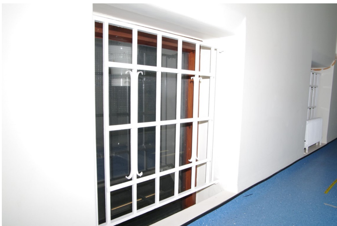
Figure 30 Former external window in central hall Seen from the first floor corridor
