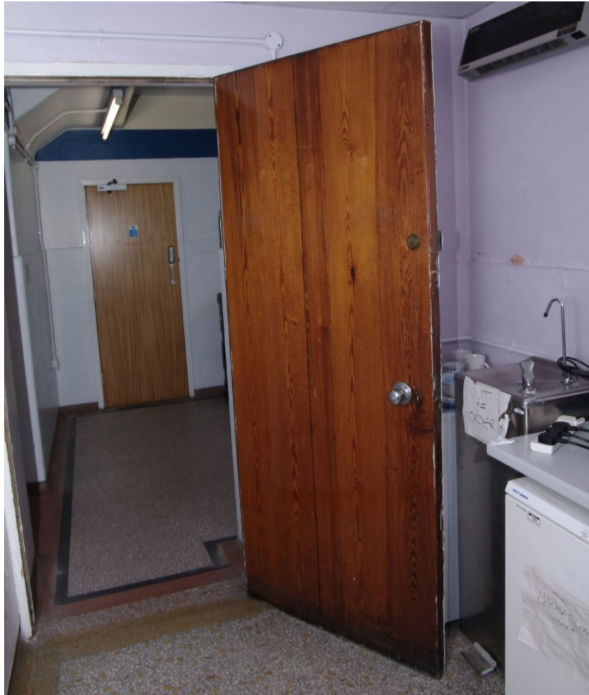
Figure 31 One of the few remaining original doors Room to south of the east fire escape. Note original terrazzo floor
