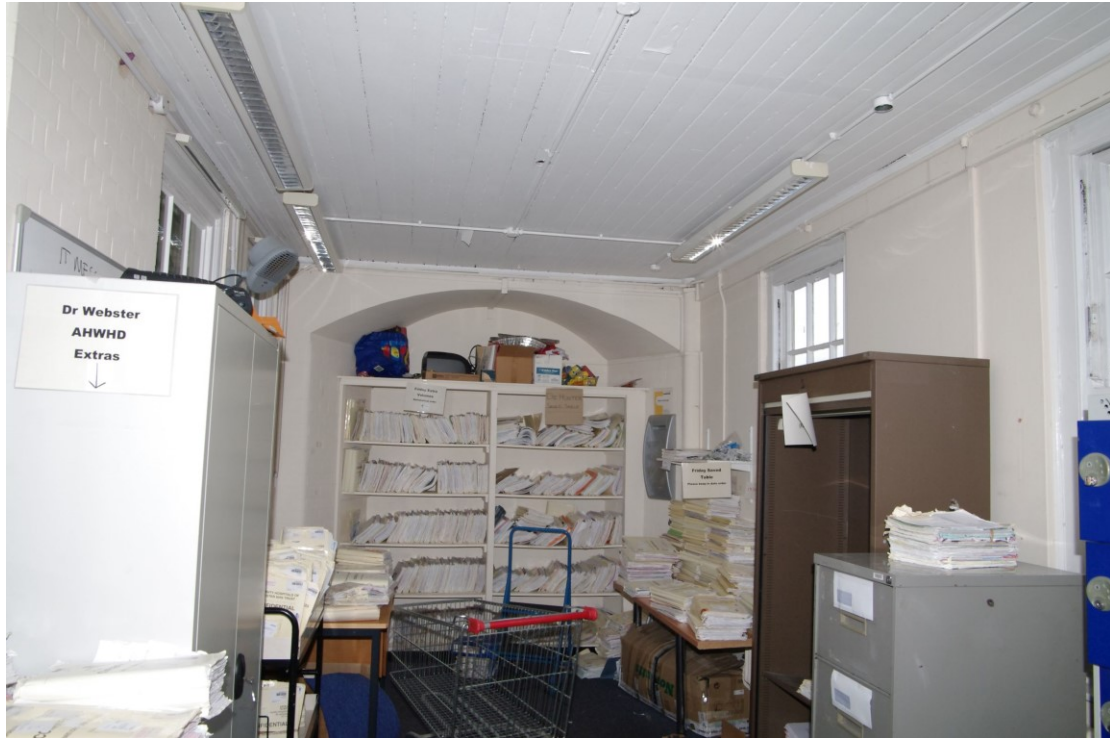
Figure 25 Blocked entrance in SE corner of building Looking north. The painted over sign in Fig. 18 is in the far right corner
