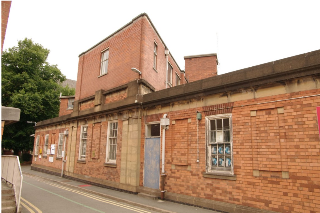
Figure 16 Close-up of south facing elevation Looking north-east. Note that the door has been modified from a window
