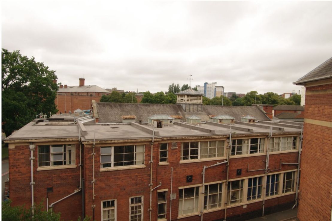
Figure 10 Knighton Street Building roofscape Looking east. Note central hall roof and tall vent
