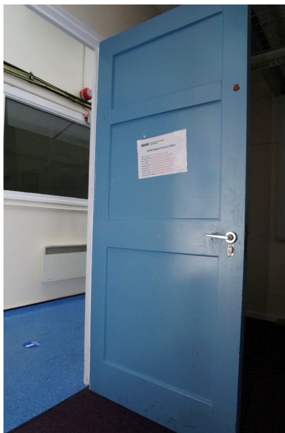
Figure 39 First floor panelled door Located on the northern corridor although others survive elsewhere
