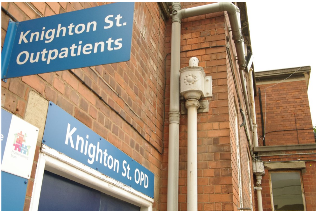
Figure 21 Decorative rainwater hopper This pattern is seen around this building and on the adjacent Knighton Street Offices
