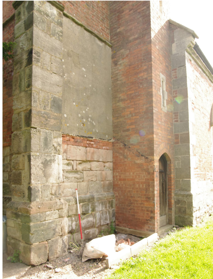
Figure 13 Location of proposed extension Looking north-east. A new clock chamber and belfry access door will be created in the brick wall to the left of the existing door.
