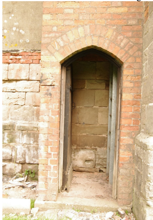
Figure 14 Open door of clock chamber and belfry access tower Looking north. The visible stonework within the doorway forms parts of a buttress which projects approximately 0.2m beyond the main wall of the tower
