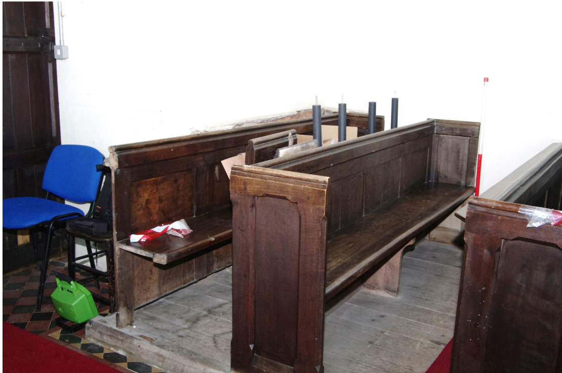
Figure 21 Pew detail on north side of nave Pews and pew platform are to be removed
