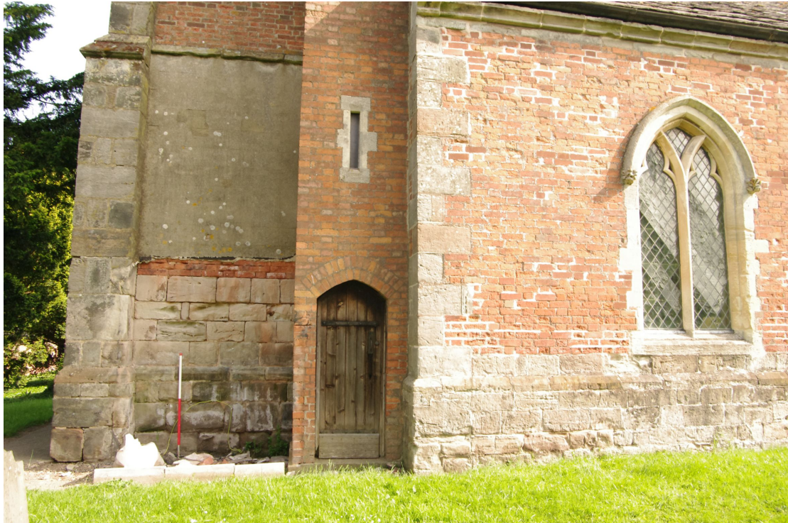
Figure 11 Location of proposed extension in SW corner Looking north. The existing clock chamber and belfry access door will be blocked, a new doorway into the tower and church will be created to the right of the 1m scale.
