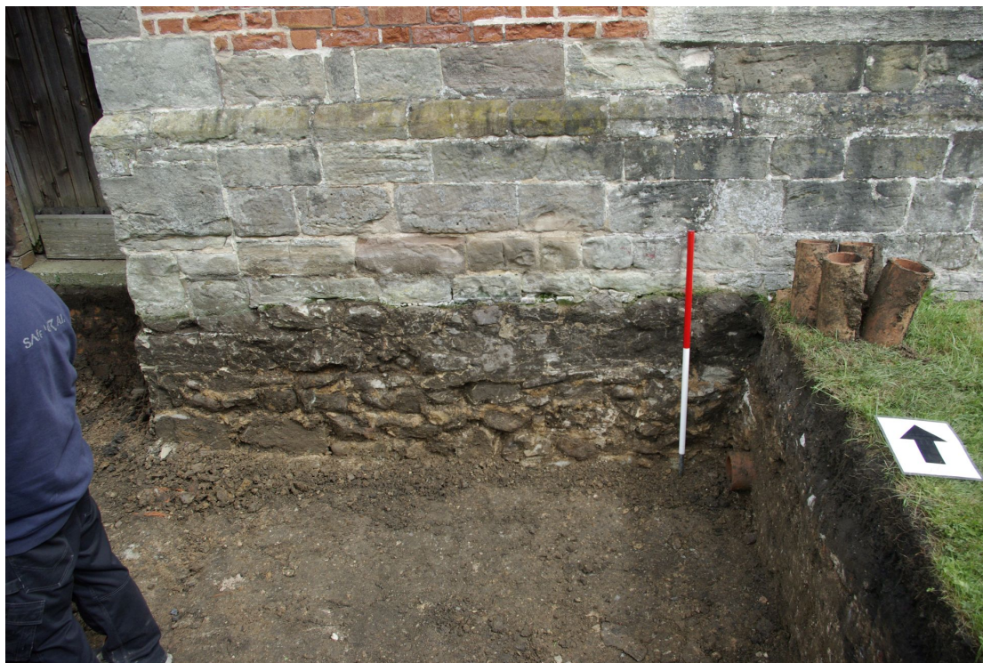
Figure 27 After removal of drain Looking north. 1m scale. The removed drainpipes are standing at the side of the trench. Note the stub of the drain extending from the side of the trench
