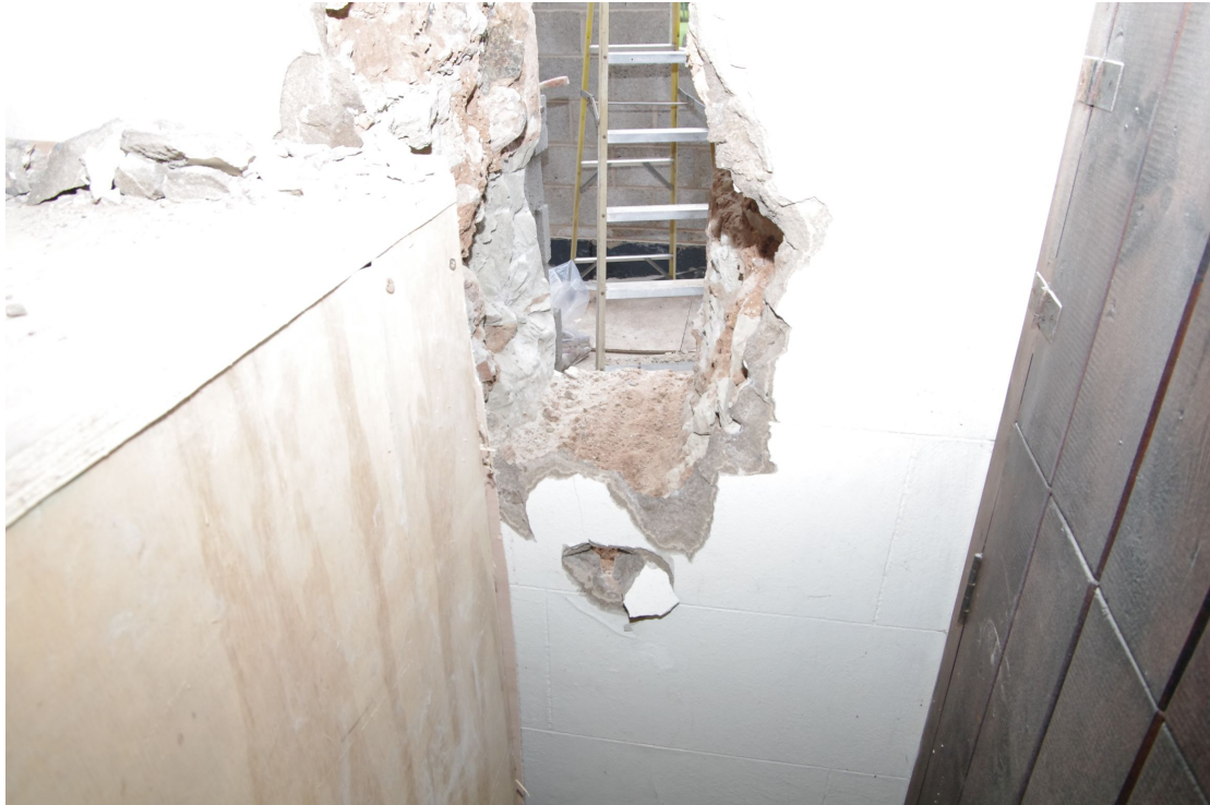
Figure 50 Close up of the plaster skin on the internal face Looking south
