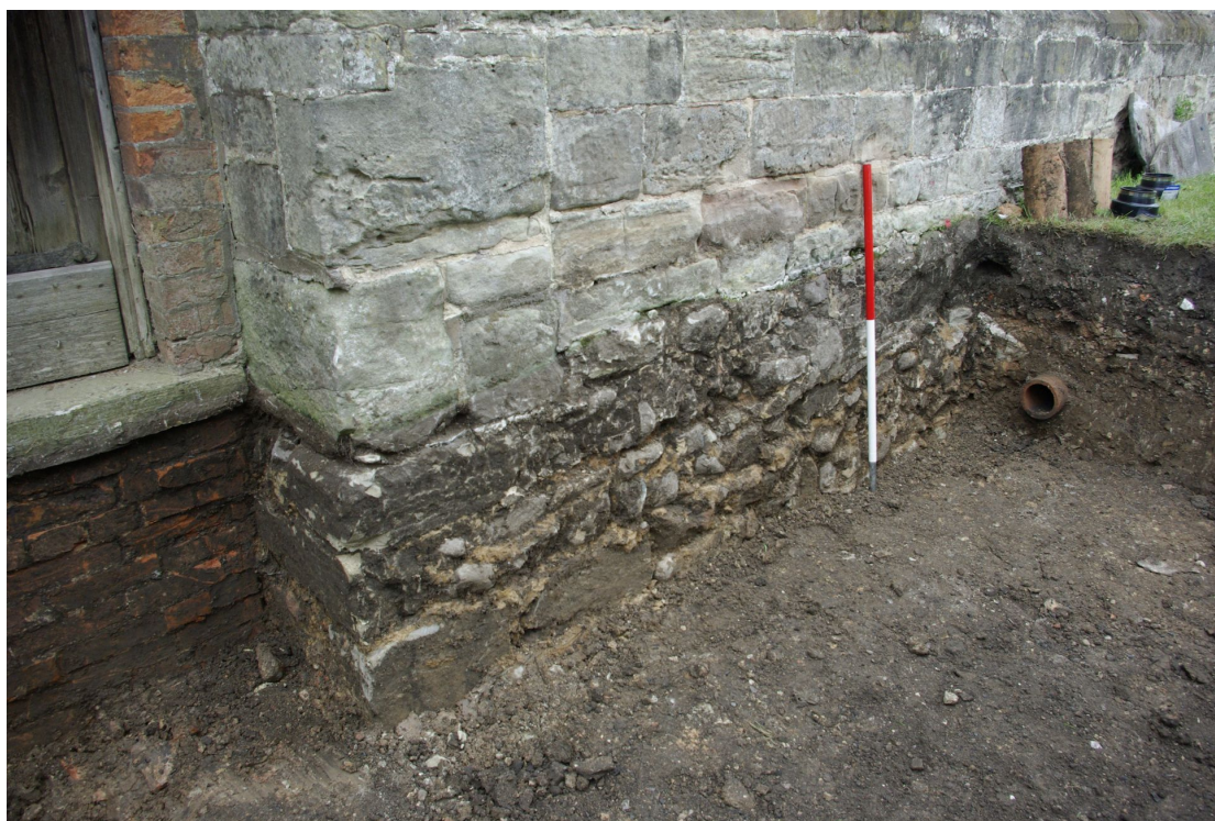
Figure 28 Exposed base of nave wall Looking north-east. 1m scale. Tower on left
