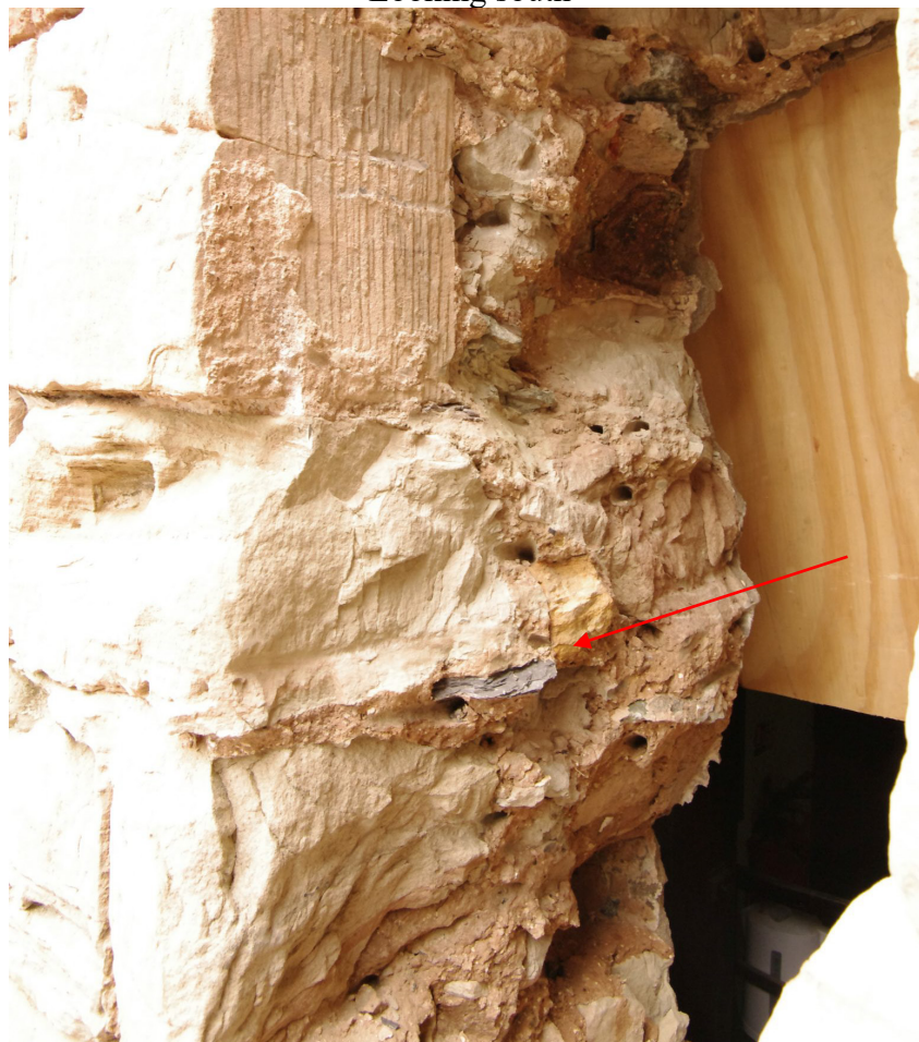
Figure 51 Piece of slate used as levelling material The red arrow points towards the slate
