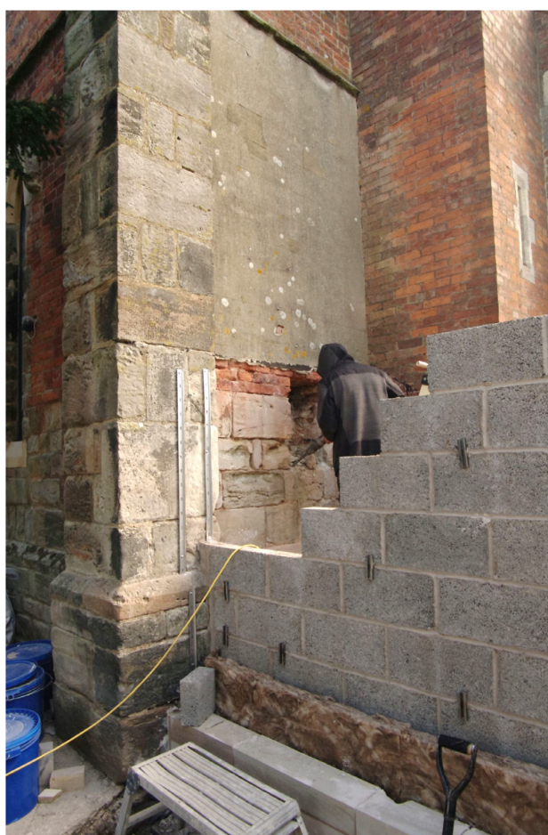
Figure 45 Initial hole being made in the south wall of the tower Looking north-east. Note the presence of the new extension by this stage
