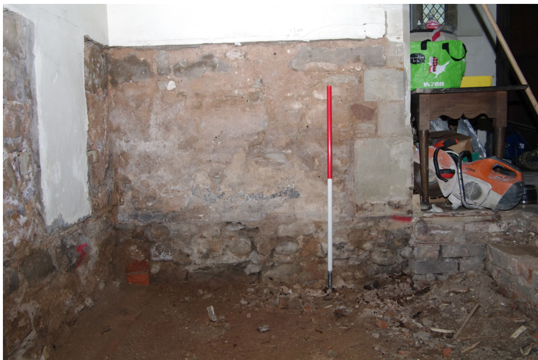
Figure 43 Tower wall on south side of aisle Looking west. Note how quoin stones stop at floor height. 1m scale
