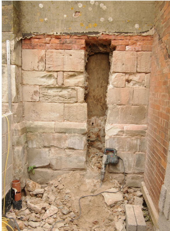
Figure 46 Full-height slot through tower wall The hole does not penetrate through the wall although a board is against the inner face in this picture
