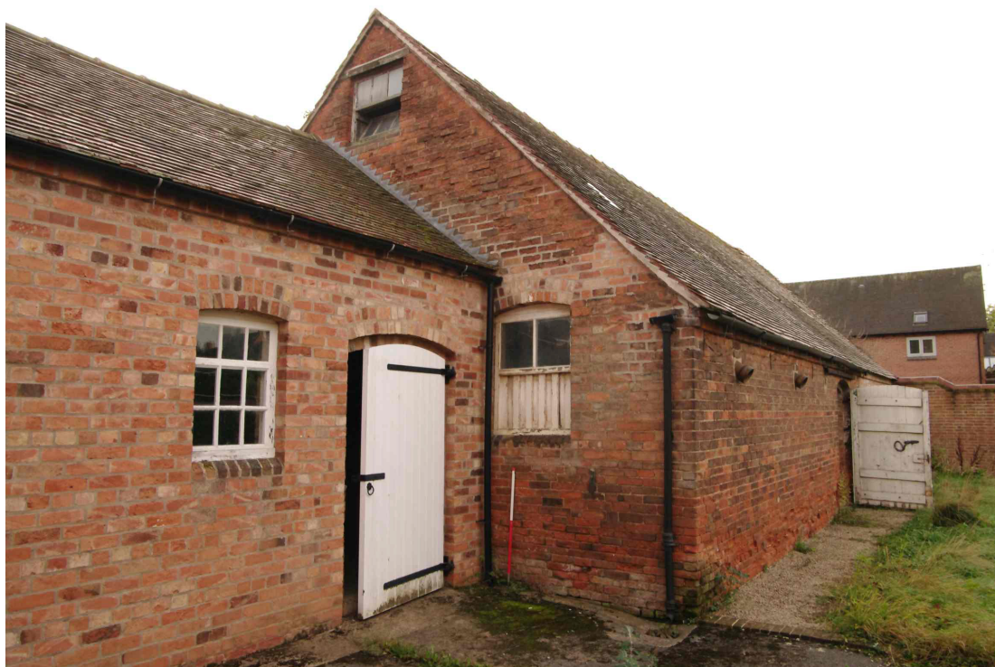
Figure 48 North facing gable end of south barn Looking south-east. 1m scale. Middle barn on left. Modern houses on right beyond the brook
