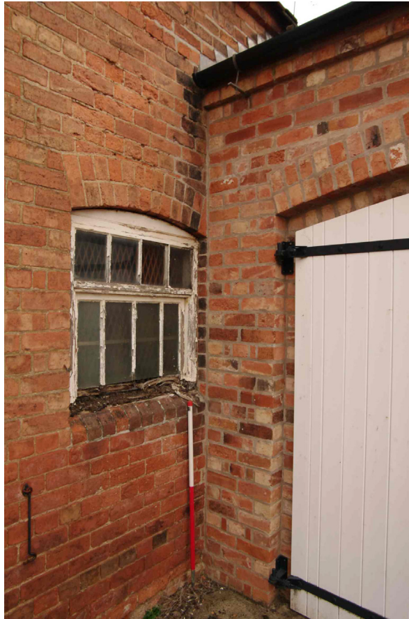
Figure 27 Junction of north barn and middle barn Looking north-east. 1m scale. The location of the (rebuilt) wall and the closeness of the window suggests that the middle barn is a later phase
