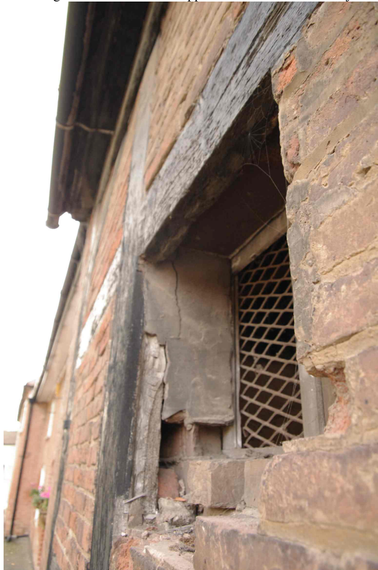
Figure 18 Close-up of timber frame and later inner brick skin Looking east along north facing elevation
