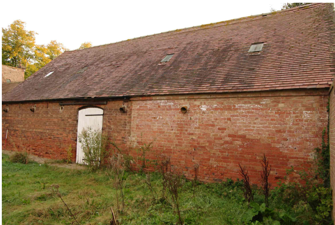
Figure 43 West facing elevation of the south barn Looking north-east. 1m scale. The wall on the extreme right of the picture is a modern wall built along the edge of the brook
