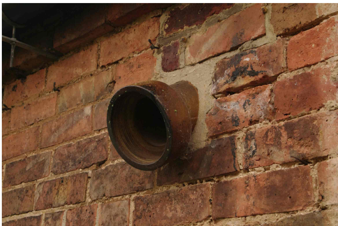
Figure 44 West facing elevation of the south barn. Vent detail The vents are made from ceramic drain sections and are likely to be mid to late 20th century replacements
