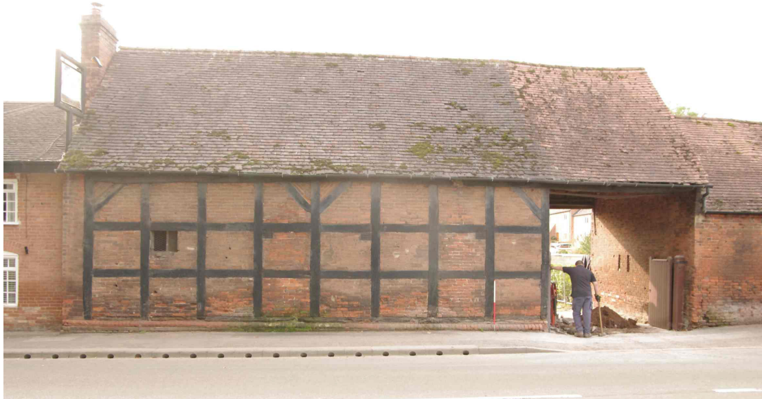
Figure 17 General view of north facing elevation Looking south. 1m scale. See Appendix 1 for details of each joint
