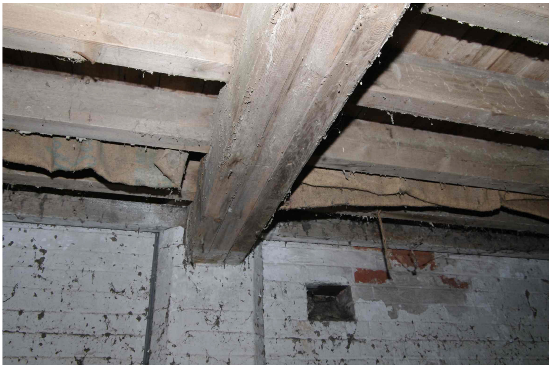
Figure 32 North barn, ground floor. Beam detail Looking north. Both beams are constructed using a ply of three narrow timbers
