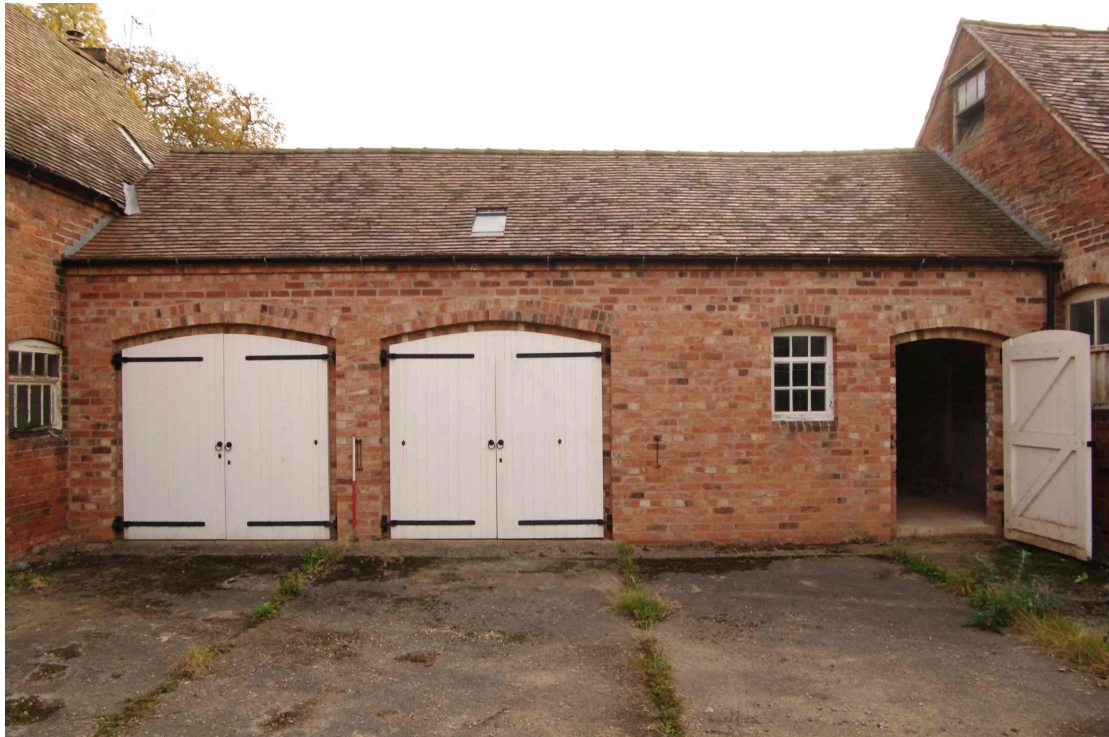
Figure 36 Middle barn, west facing elevation Looking east. 1m scale. This wall has recently been rebuilt but appears to follow the earlier wall line and has used old bricks. It is not known if the doors and windows follow an earlier layout. The woodwork is all modern
