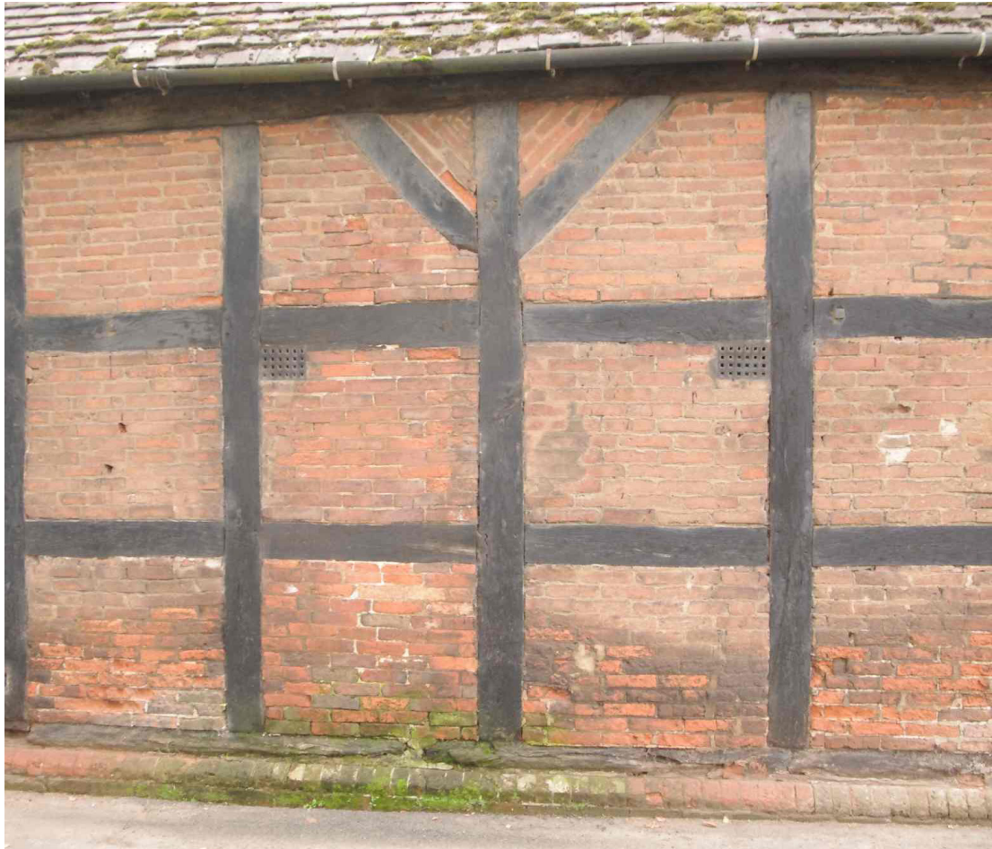
Figure 19 Close-up of brick infilling Looking south at north facing elevation. Note the brick plinth supporting the sill-beam
