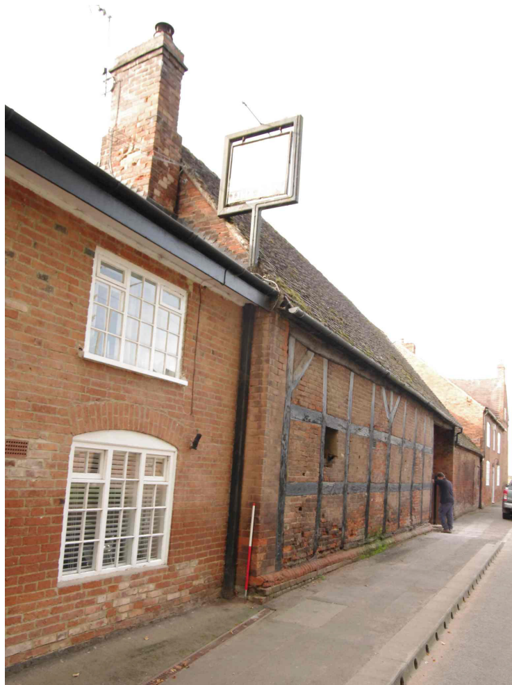
Figure 15 North facing elevation and joint with former public house Looking south-west. The brickwork behind the 1m scale is late 19th or 20th century
