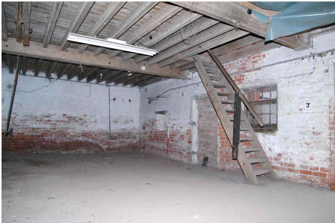
Figure 29 General view of north barn ground floor Looking south-east. 1m scale. Note blocked door and window. Also the saddle trees and empty sockets in the far corner
