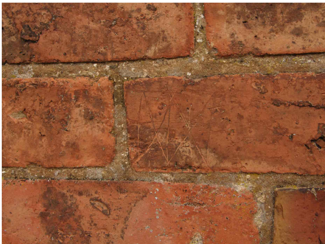
Figure 47 Possible apotropaic mark on west facing elevation Located approximately midway between the doorway and the north-west corner of the barn
