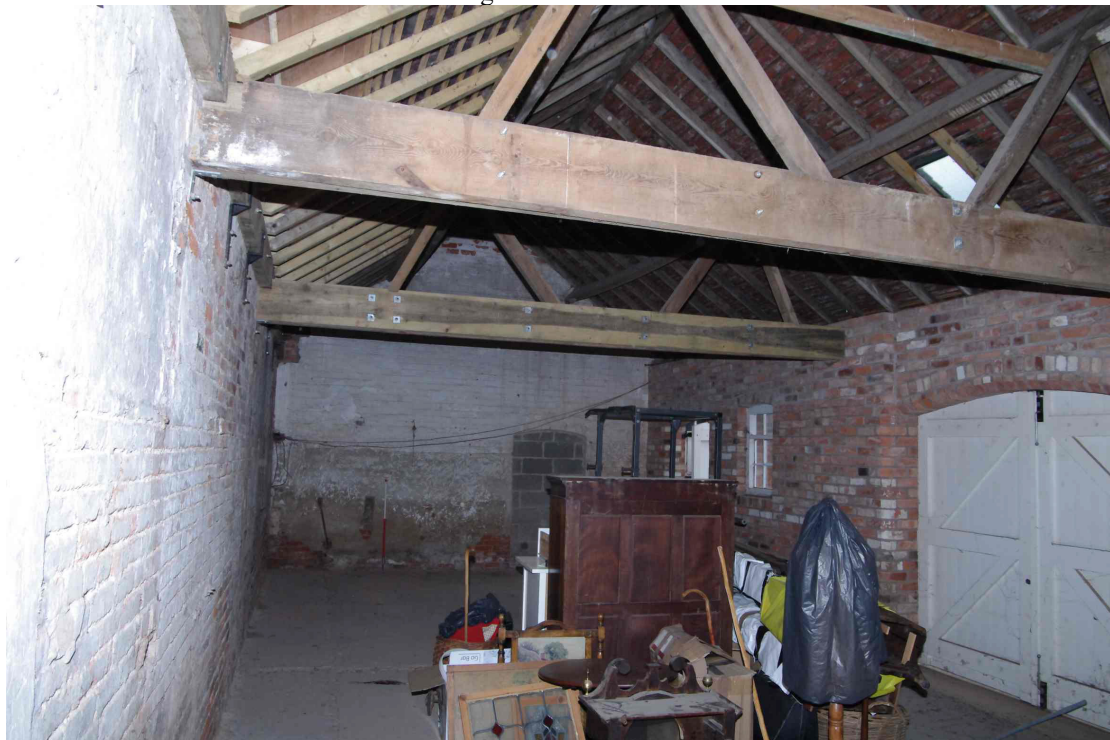
Figure 38 Inside the middle barn Looking south-west. Only the west wall (on right) appears to have been rebuilt along with the roof structure. Note blocked door to south barn on end wall
