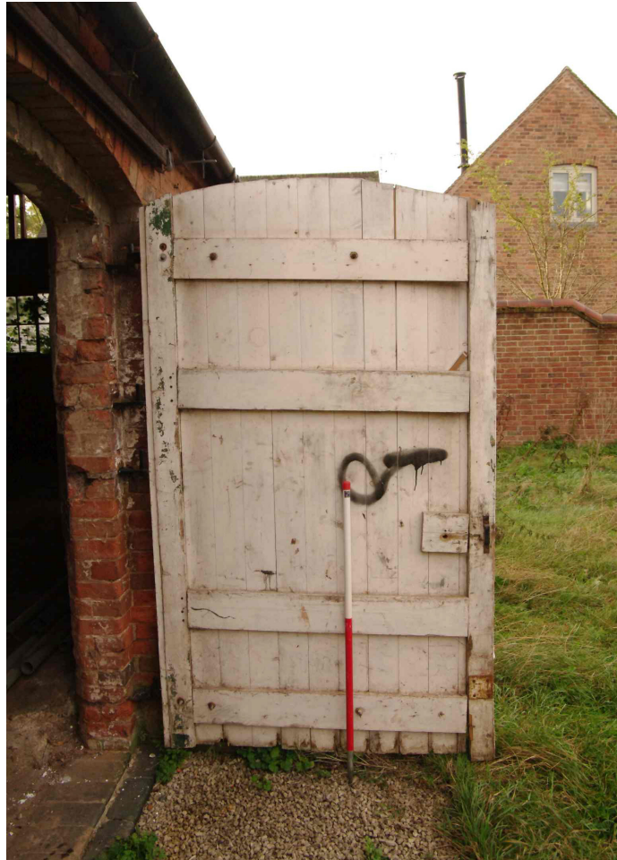
Figure 45 South barn door detail Door located on the west facing elevation. 1m scale
