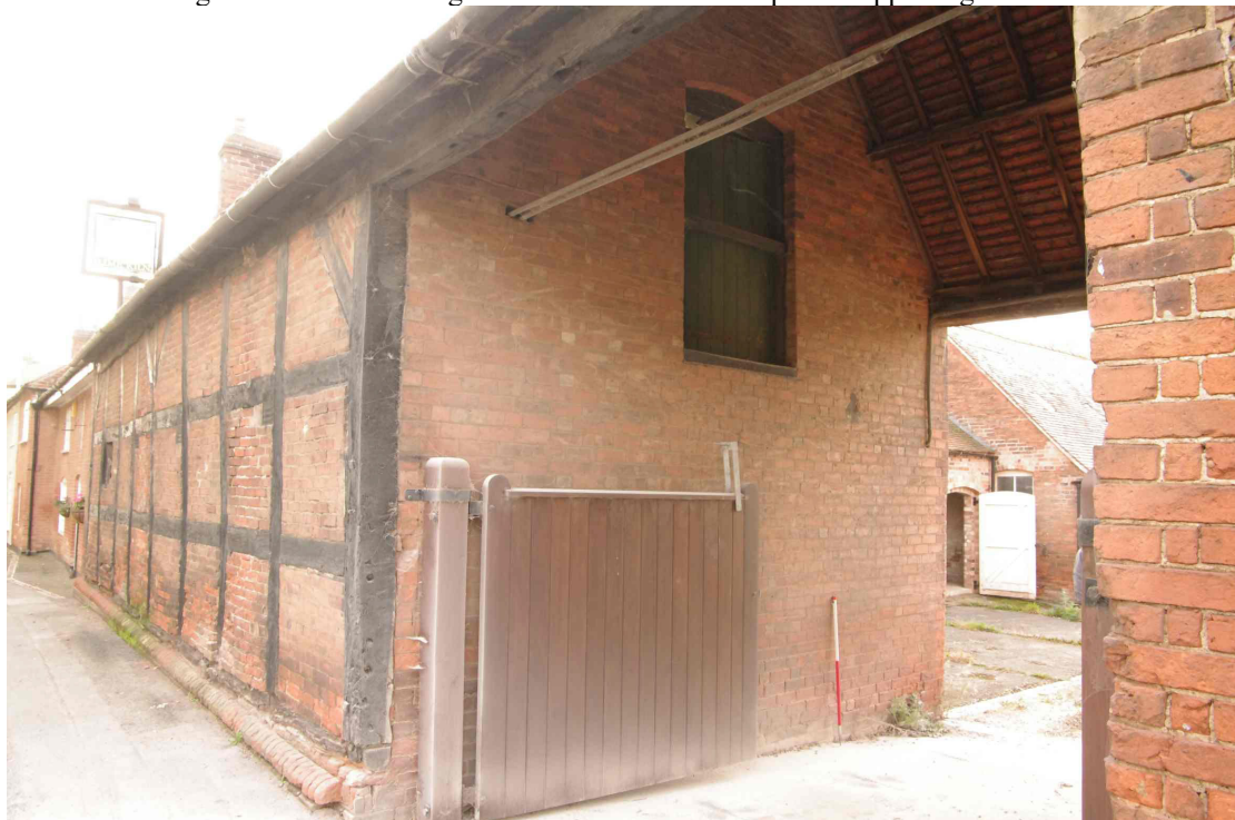
Figure 20 Covered entrance into yard Looking south-east. 1m scale. Note re-used timber used as a lintel above the entrance
