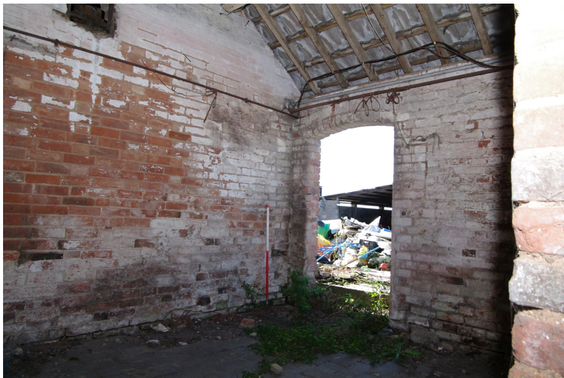
Figure 45 Building 5. Cross-passage from the yard Looking south-west. Note the bearing box top left. Building 2 can be seen through the doorway
