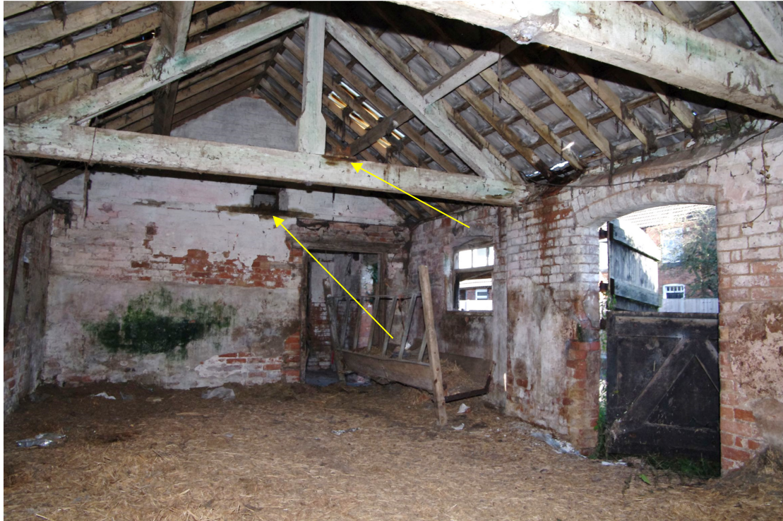
Figure 47 Building 5. Centre room Looking north towards the cross-passage doorway. The two arrows point towards the bearings
