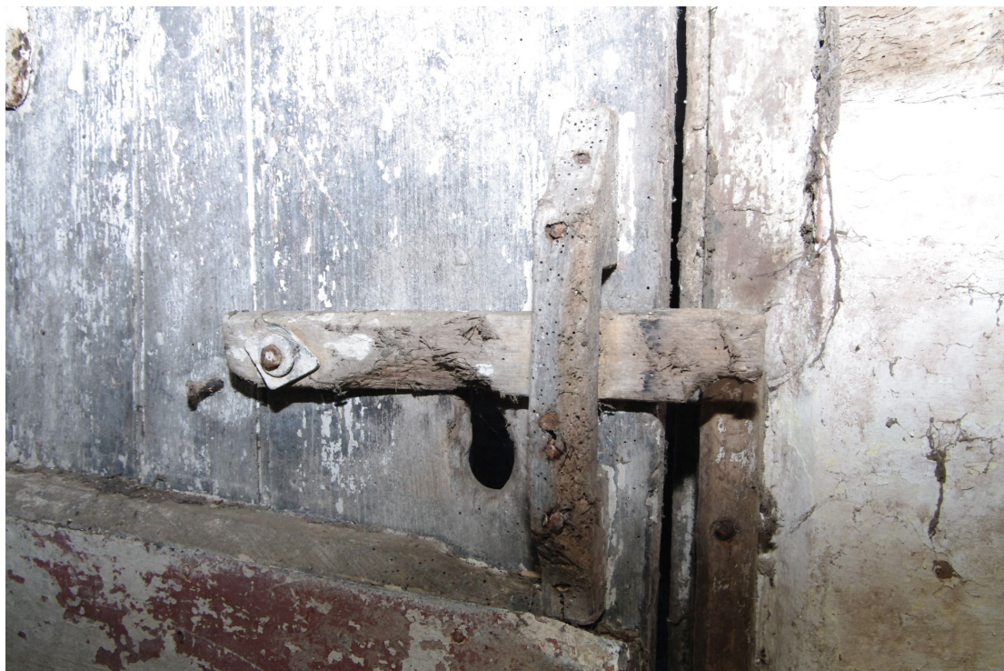
Figure 44 Building 5. Door detail at southern end of north room The latch and catch are both wood
