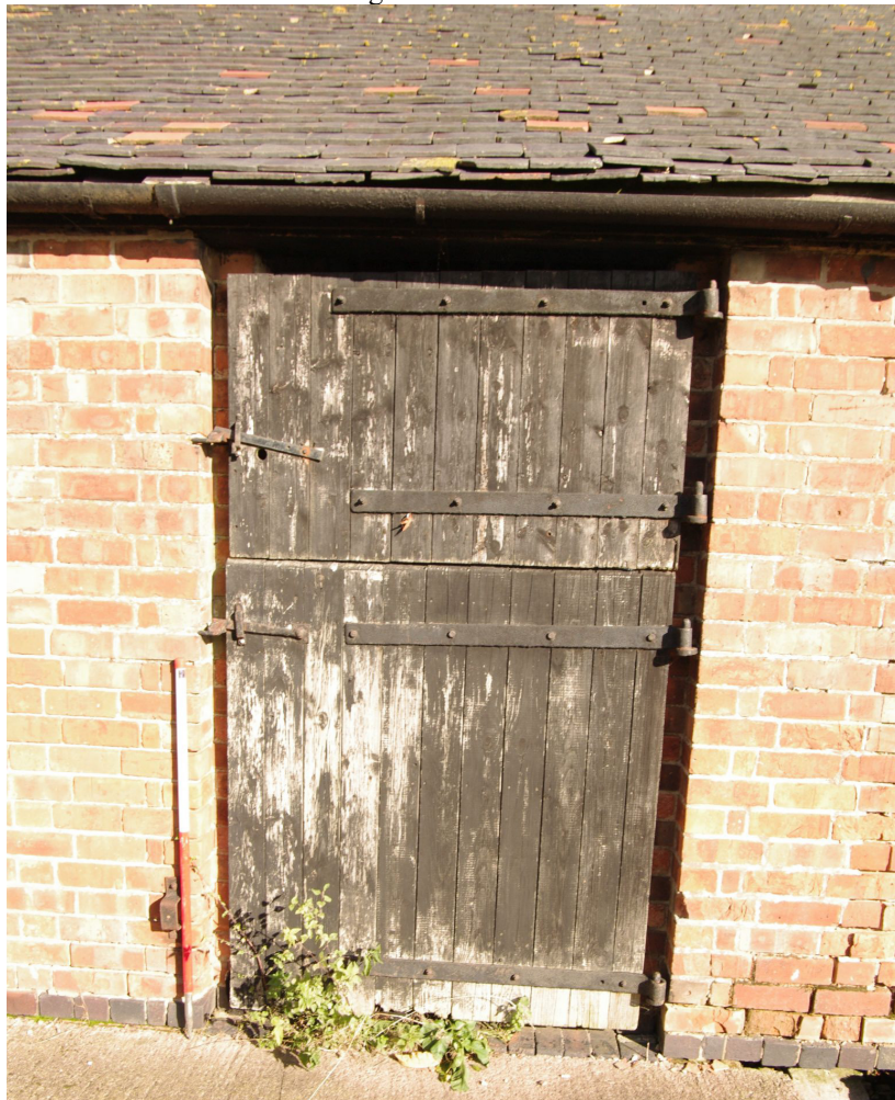
Figure 71 Building 7 south-west facing elevation of single storey range Door detail. Looking north-east. 1m scale
