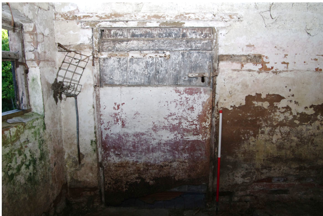
Figure 43 Building 5. Door detail at southern end of north room Looking south-east. 1m scale. The lower part of the door has a modern covering but still shows the hand-made hinges and wooden latch (see Fig. 44 below)
