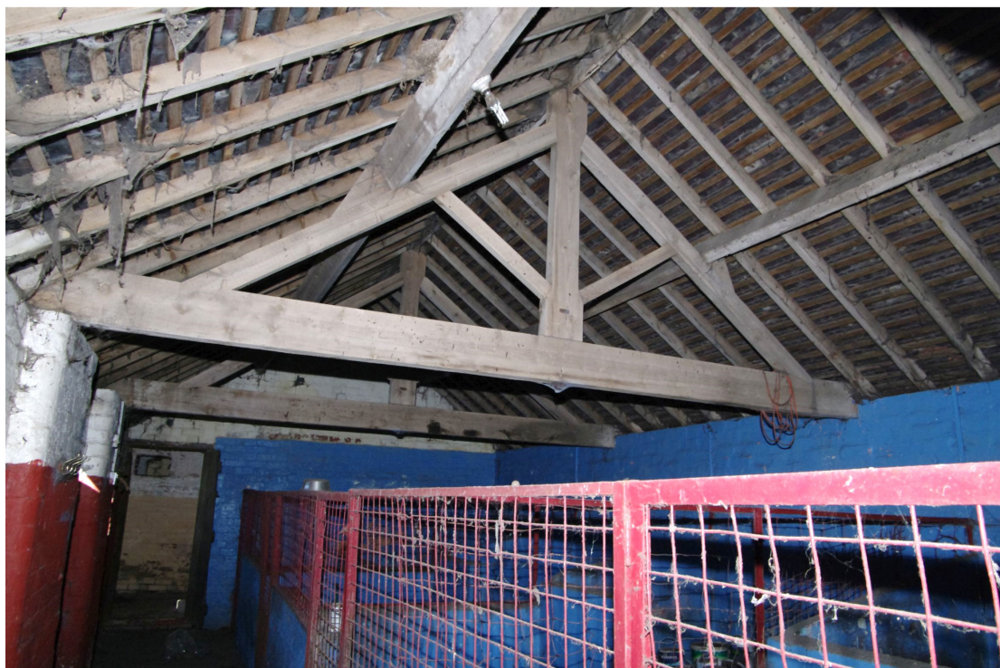
Figure 88 Building 7. Room 8 roof structure Looking north-west. The doorway to the far left leads into Room 7
