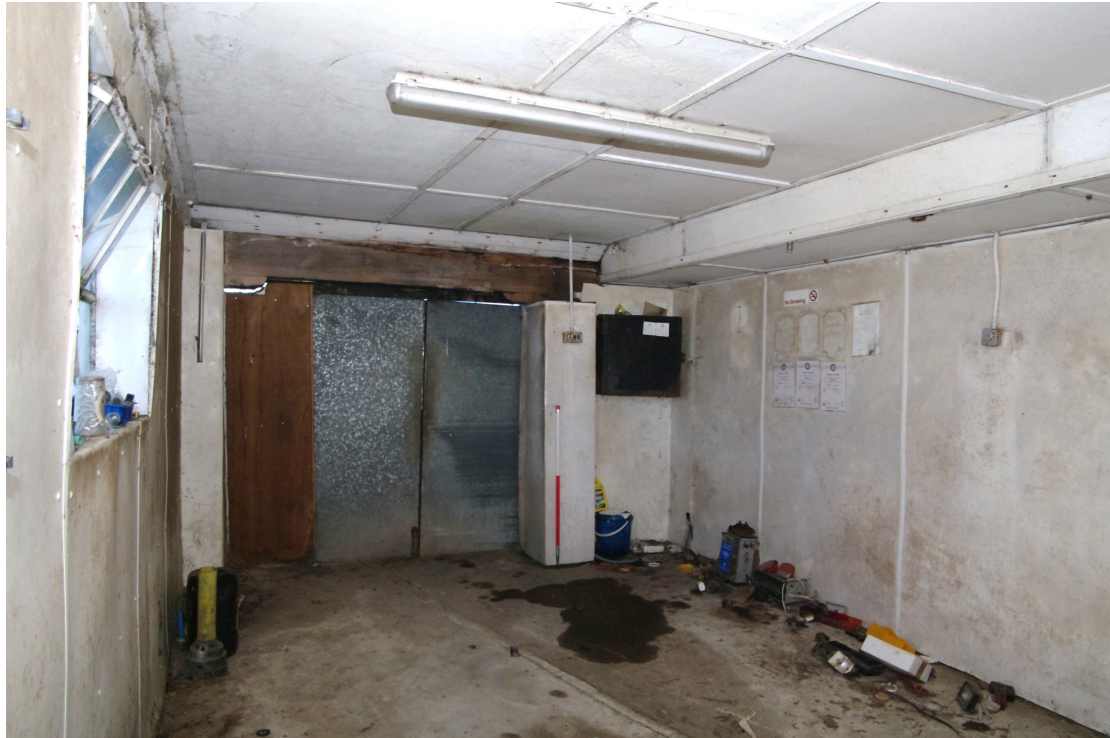
Figure 17 Building 1 side room Looking north-east. 1m scale. The room has been lined for dairy work
