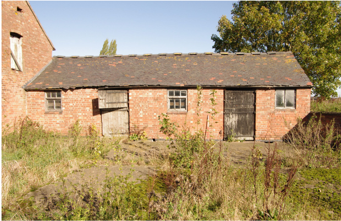
Figure 70 Building 7 south-west facing elevation of single storey range Looking north-east. 1m scale
