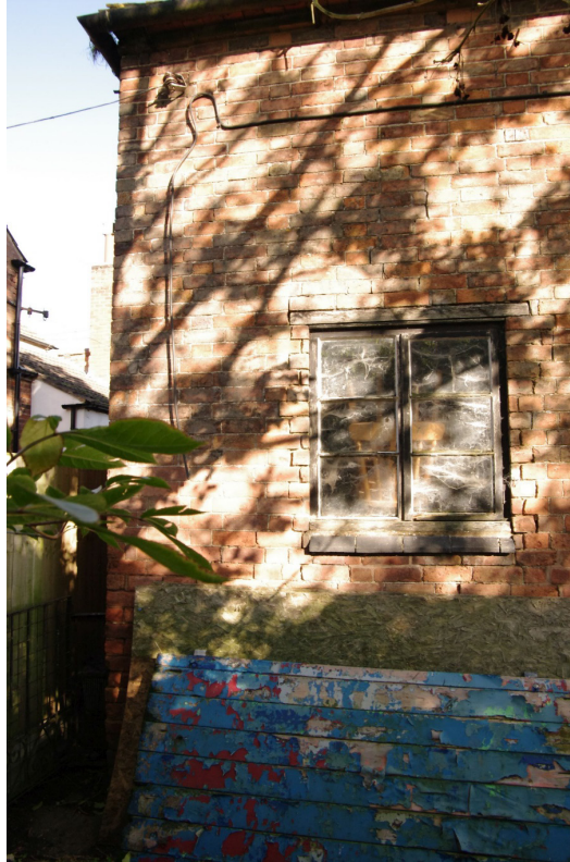
Figure 68 Building 7 south-west facing elevation of two storey range Looking north-east at ground floor window at northern end of building
