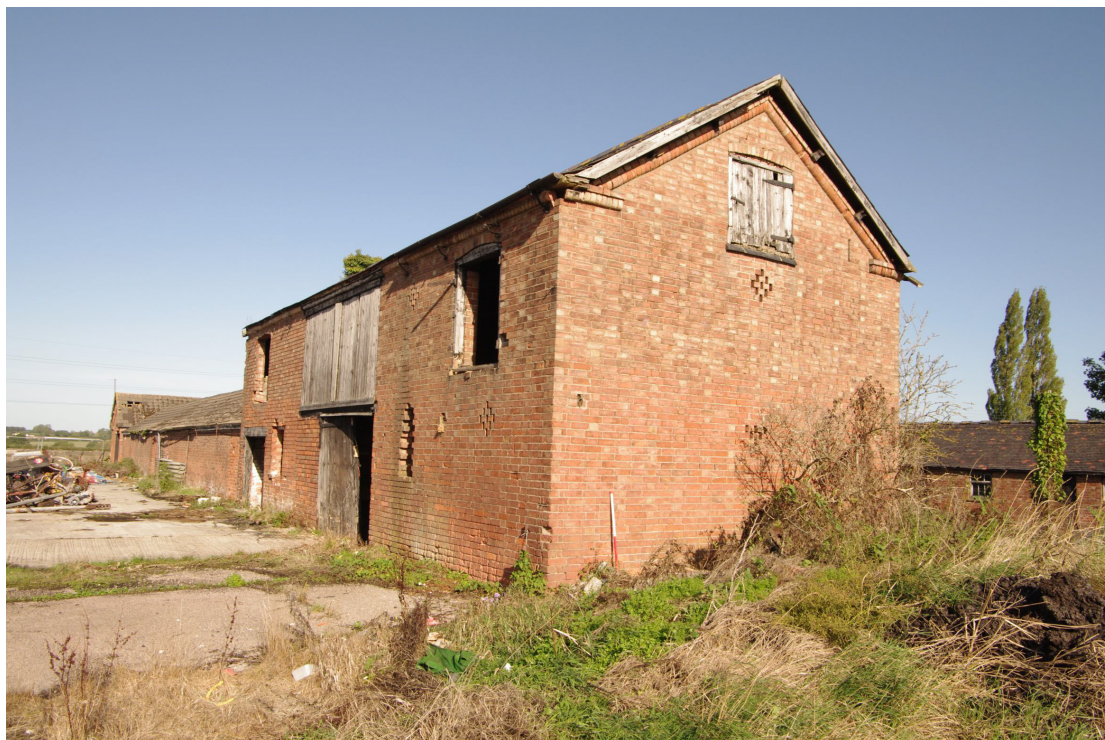
Figure 53 Building 6 south-west and south-east facing elevations Looking north. Building 7 on far right. 1m scale
