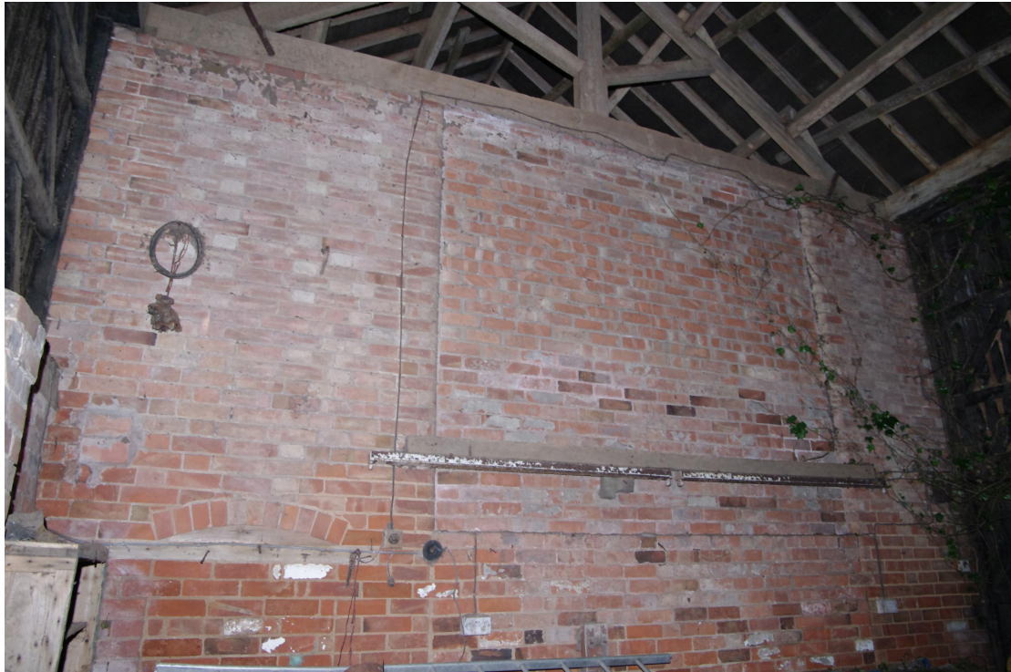
Figure 61 Building 6 Wall on northern side of central space Looking north. Note the blocked ground floor doorway and partial blocking of the first floor hayloft area. Note also the timberwork either side which blocks the upper levels of the former threshing doors
