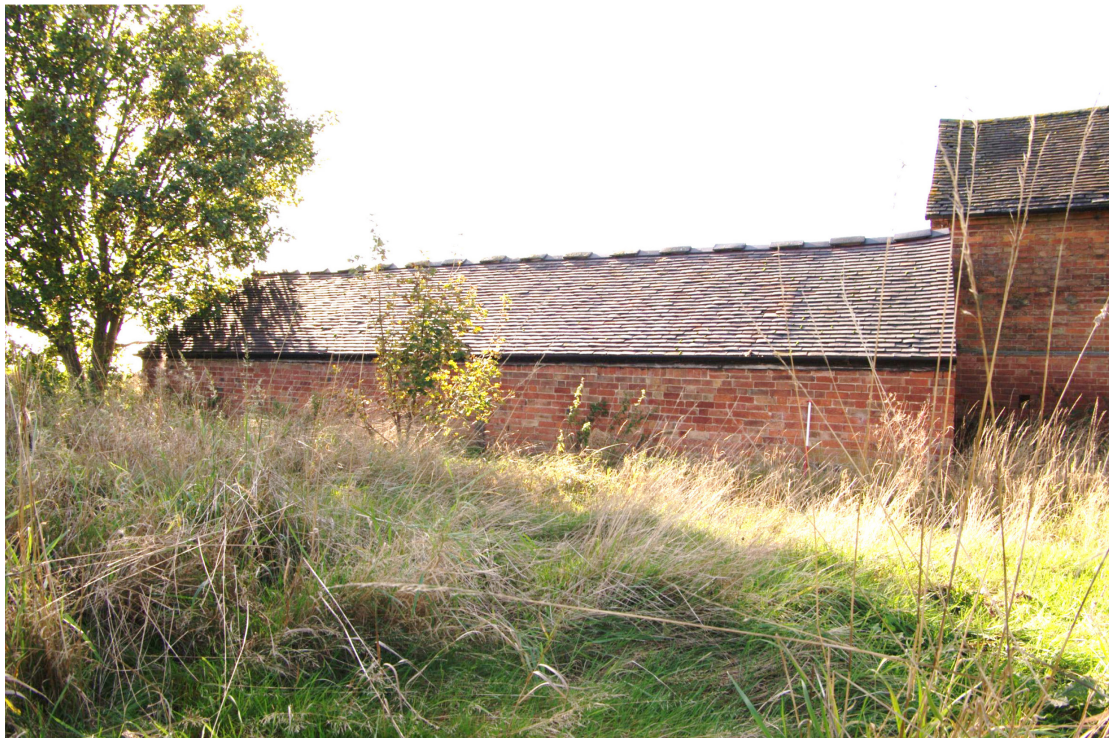
Figure 73 Building 7 north-east facing elevation of single storey range Looking south-west. 1m scale
