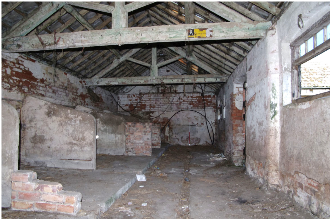
Figure 40 Building 5, northernmost room Looking north-west. Note concrete stalls, later 19th century roof structure and enamel sign on beam (see Fig. 41 below). 1m scale
