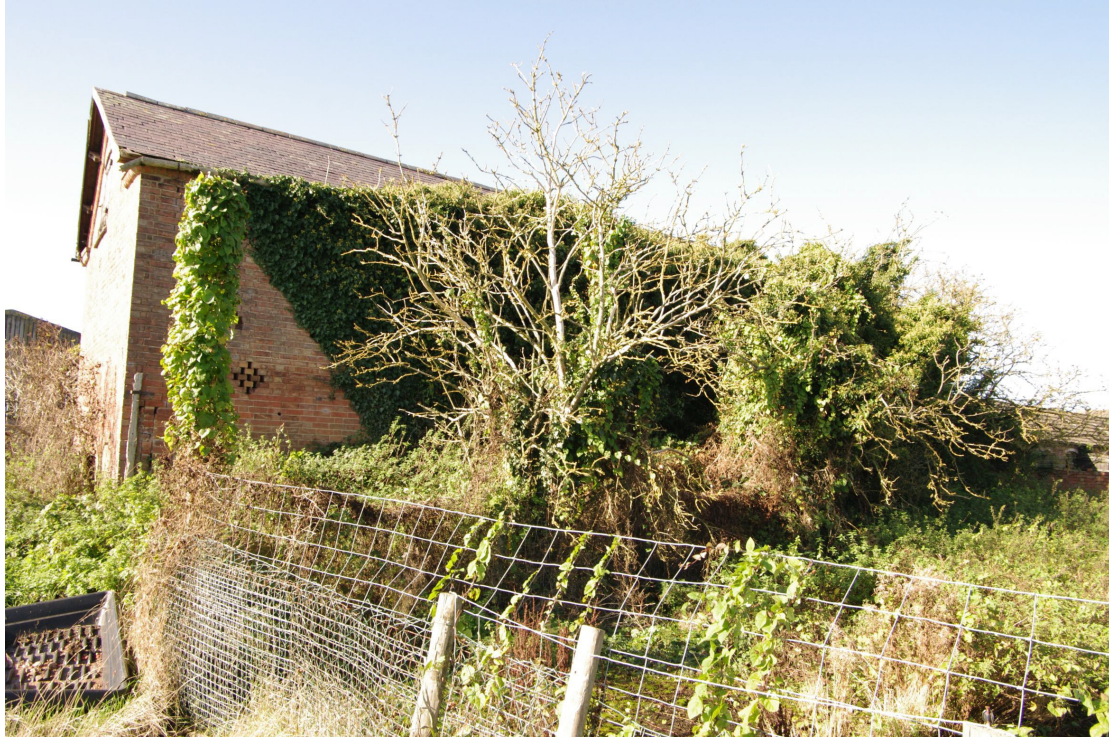
Figure 55 Building 6 north-east facing elevation Looking north-west. Beneath the vegetation is another partially blocked central doorway and a blocked ground floor doorway to the north of the central opening
