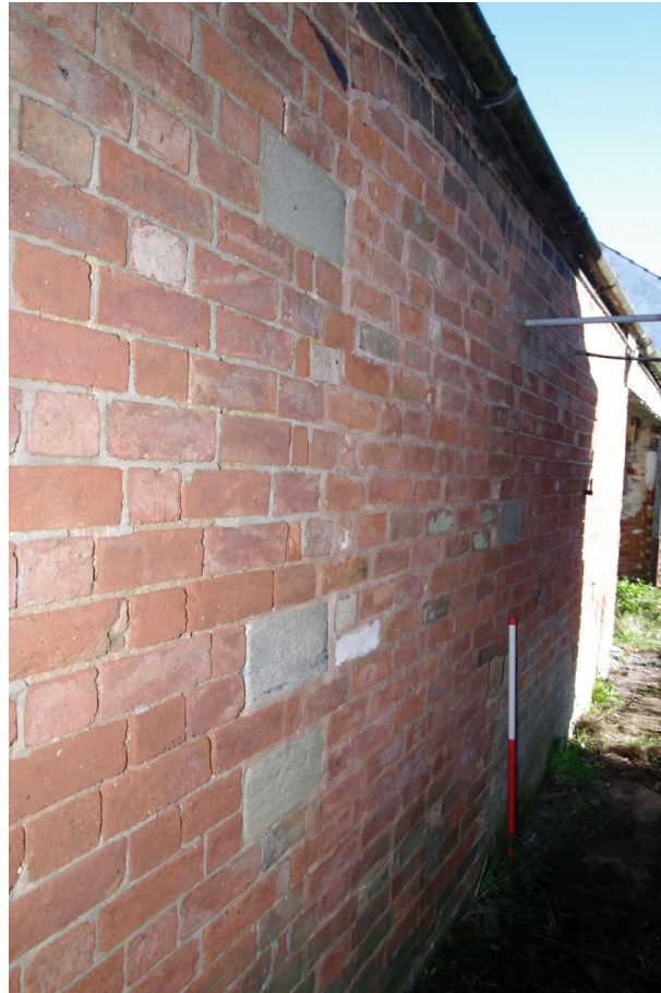
Figure 25 Passageway between Buildings 4 and 5 Looking north-east. Noted bricked up doorway to left of 1m scale, this might suggest that Building 4 (on left) is earlier than building 5 (on right)
