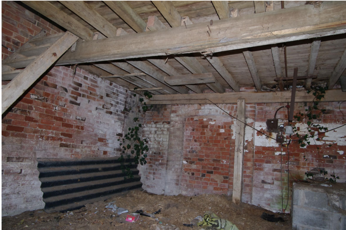
Figure 57 Building 6. Ground floor room on north side Looking north-east towards blocked doorway on north-east facing elevation
