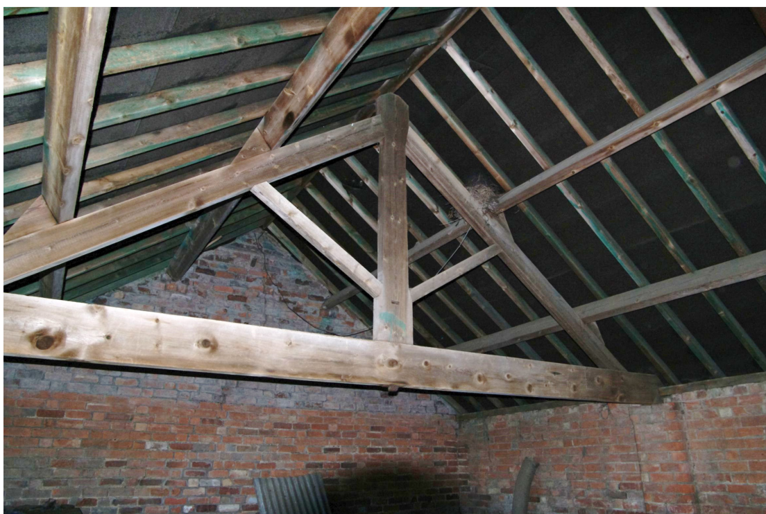
Figure 16 Building 1 roof structure Looking west. The bolted timbers are typical of late 19th century agricultural structures
