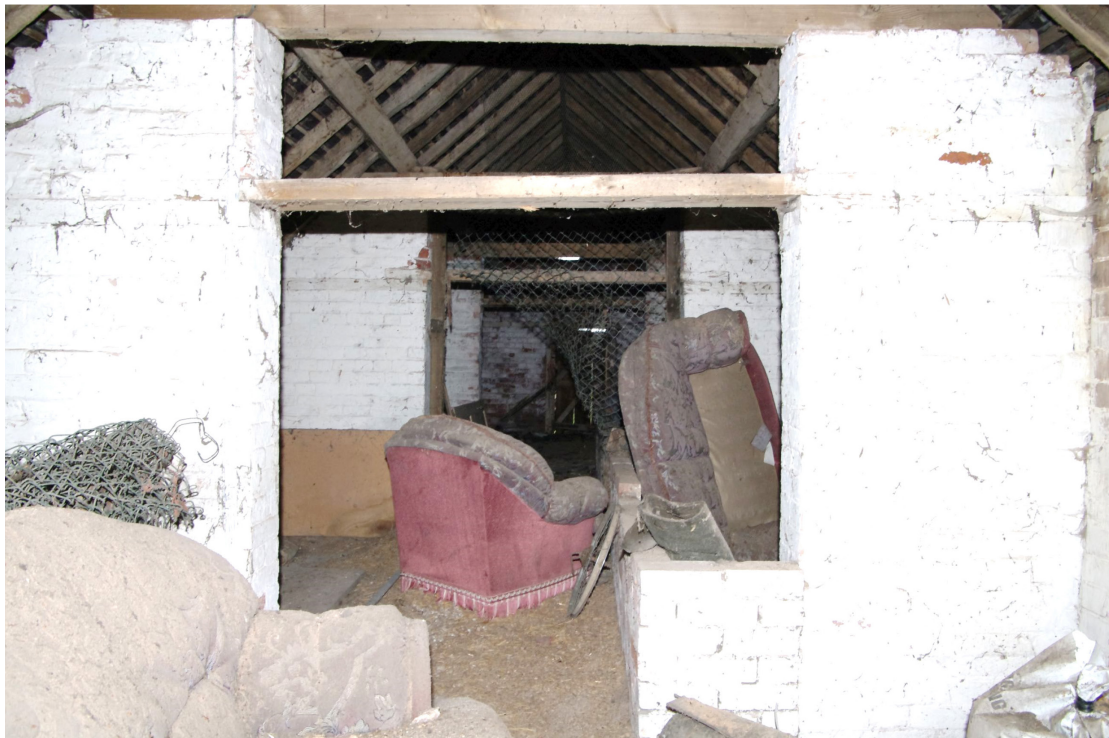
Figure 91 Building 7. Room 10 Looking south-east along the first floor of the two storey range
