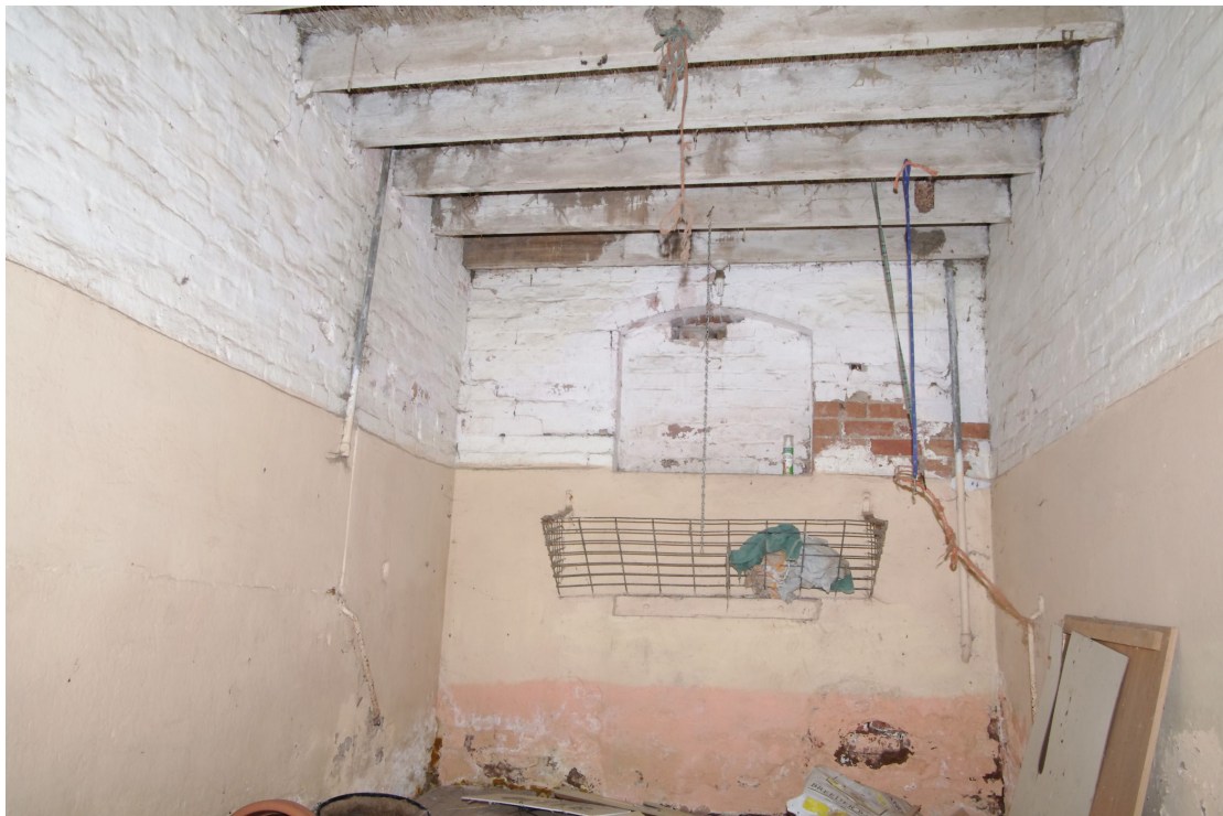
Figure 81 Building 7. Room 3 Looking north-west. The small window has been blocked due to the addition of the outside lean-to Room 1 behind it
