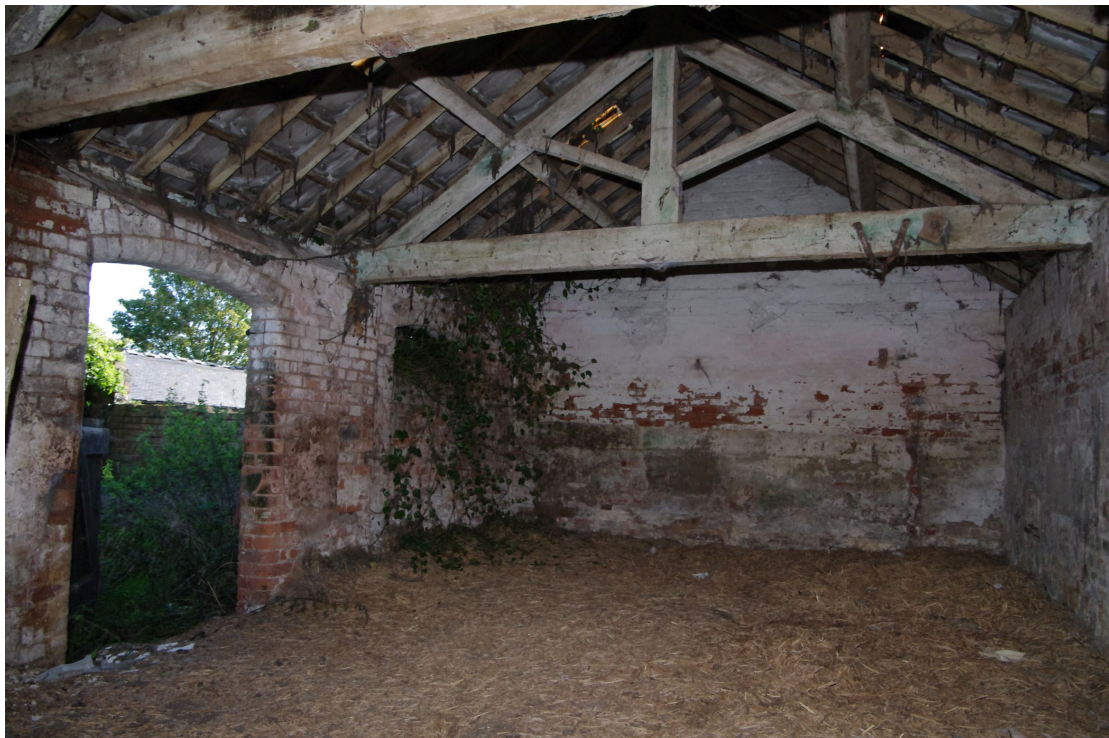
Figure 48 Building 5. Centre room Looking south-east. The roof structure appears to be later 19th century
