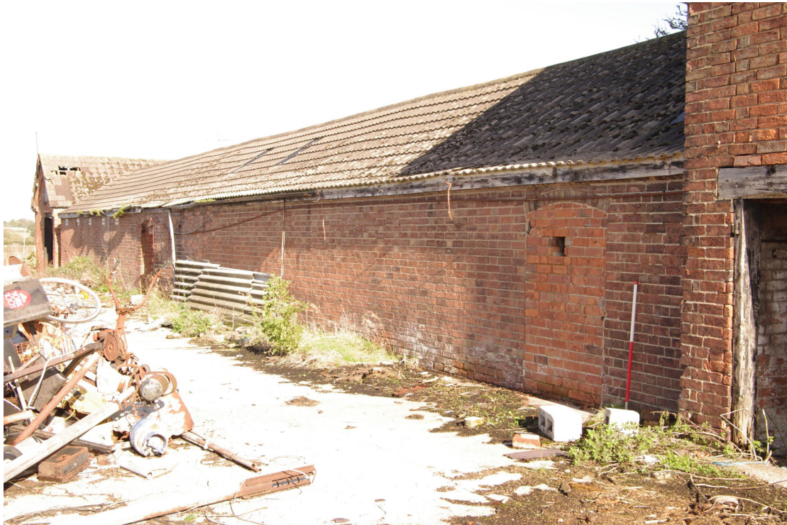
Figure 39 Building 5 south-west facing elevation Looking north-east. Note blocked doorway to left of 1m scale, one of only two doors on this face
