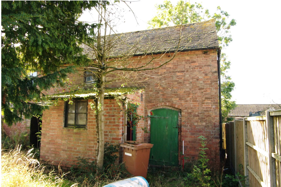
Figure 76 Building 7 north-east facing elevation of two storey range. Northern end Looking south-west. 1m scale
