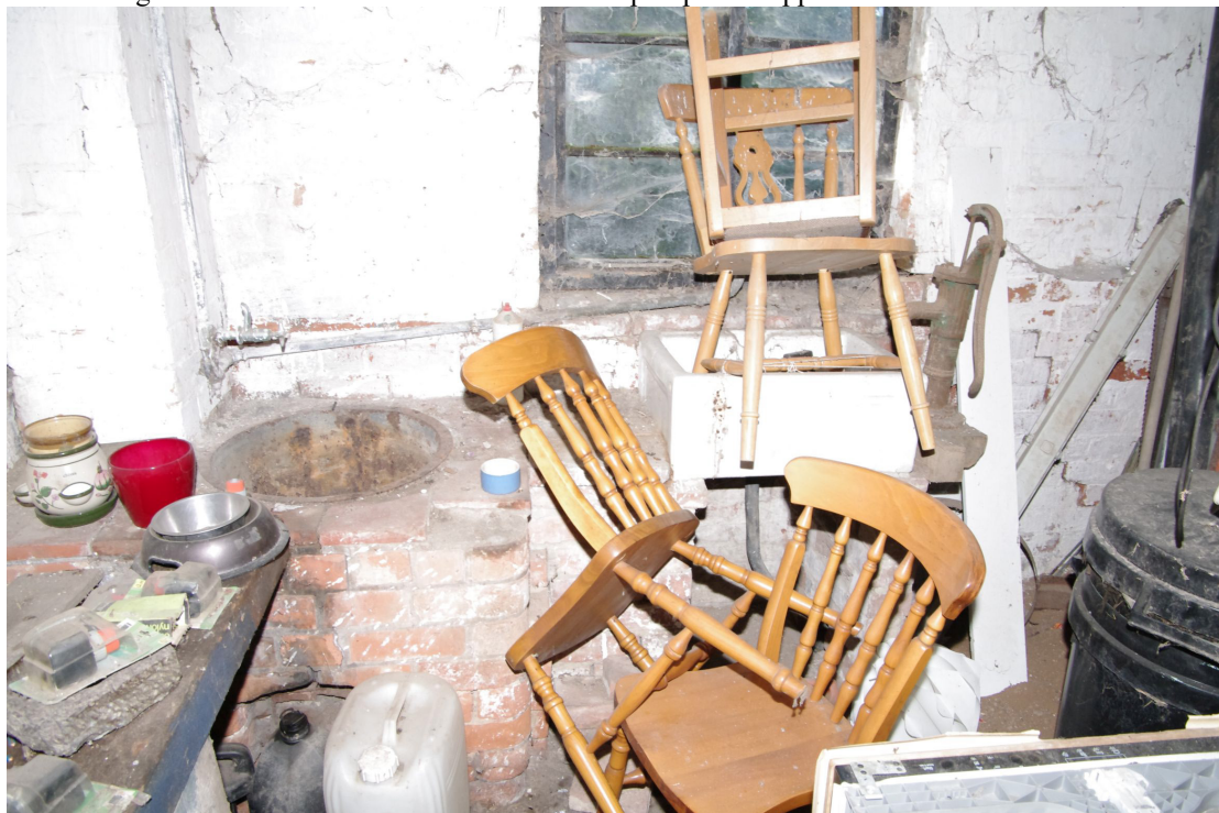
Figure 79 Building 7. Room 2 water pump
