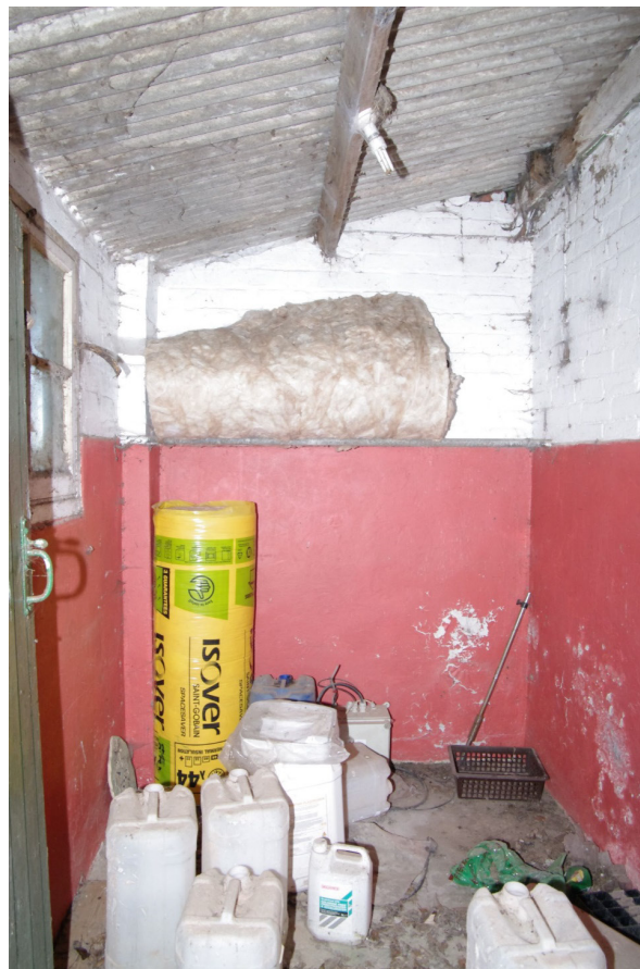
Figure 77 Building 7. Room 1 Looking south-east. This room is a small added-on lean-to structure
