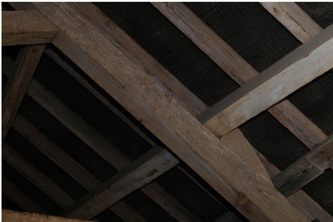
Figure 60 Building 6 rase marks on principal rafter and purlin Looking south-east from first floor room
