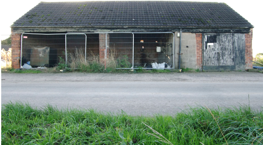
Figure 10 Building 1 former cart shed Looking south-east. 1m scale The right hand end forms a separate room
