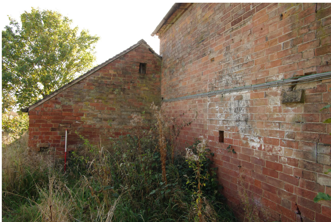
Figure 74 Building 7 north-west facing gable end of single storey range Looking south-west. 1m scale. The brickwork shows evidence of a now removed lightweight lean-to being fitted into the corner of the two ranges
