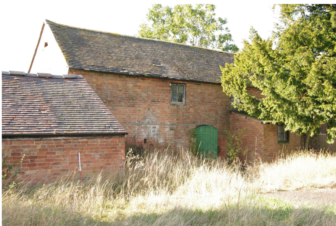
Figure 75 Building 7 north-east facing elevation of two storey range Looking north-west. 1m scale
