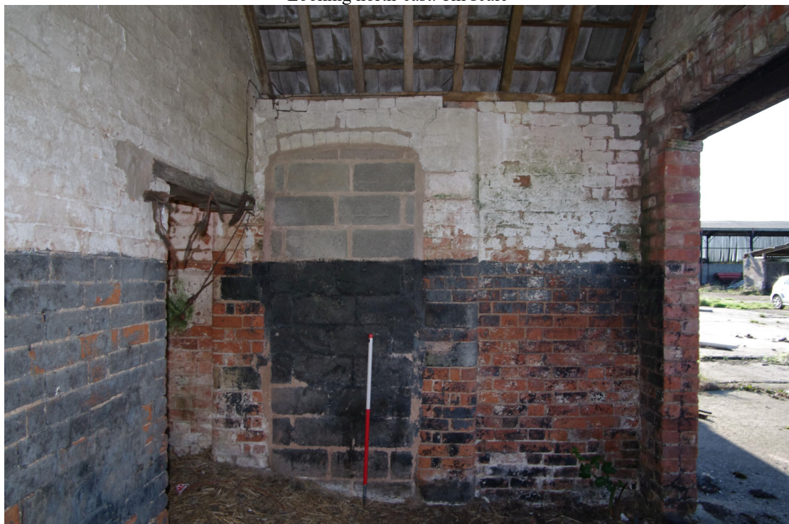
Figure 32 Building 4: western end room Looking south-east. Blocked doorway (seen in Fig. 25) behind 1m scale. Note modern steel lintel on opening to right
