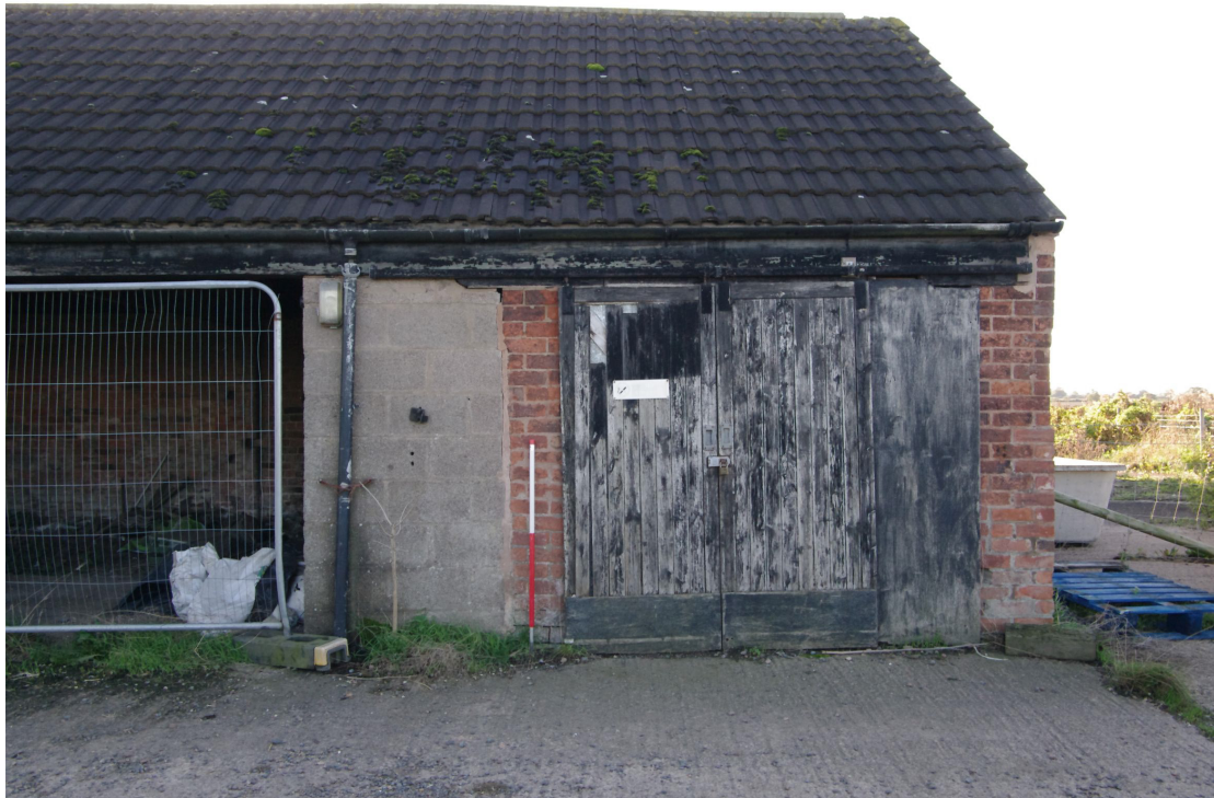
Figure 11 Enclosed western end of Building 1 Looking south-east. The concrete blockwork to the left of the 1m scale is modern and has extended the size of the end room
