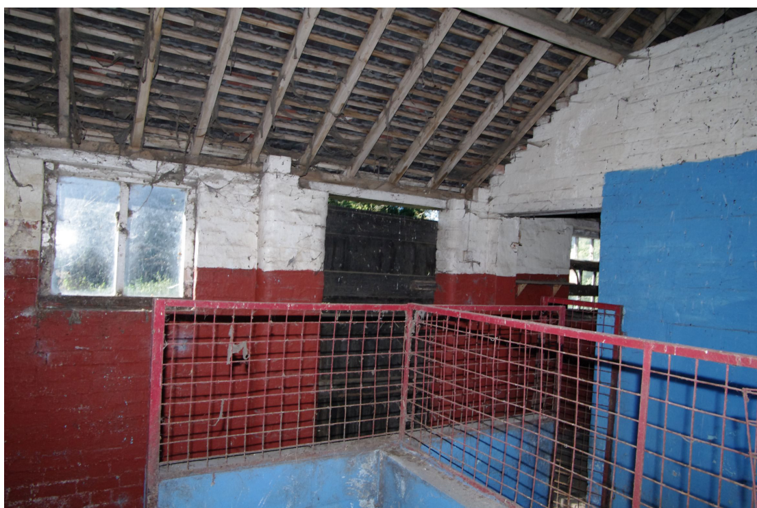
Figure 89 Building 7. Room 9 Looking west. The door to the right leads into Room 8
