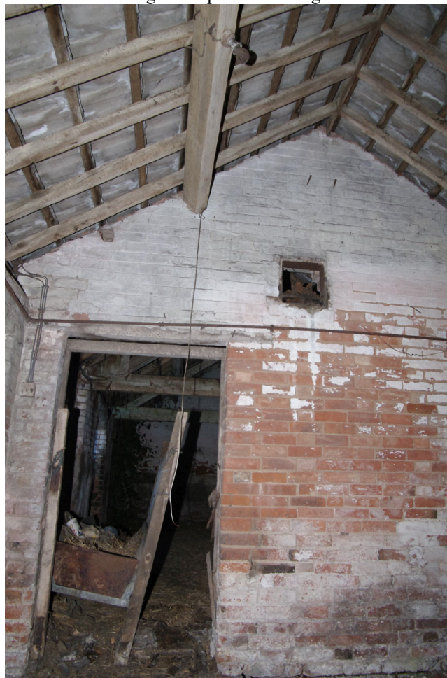
Figure 46 Building 5 south wall of cross-passage Looking south-east. Note bearing box in gable
