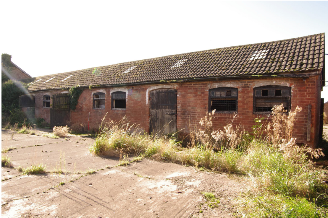
Figure 35 Building 5 north-east facing elevation Looking south-west. The gable end of Building 6 can be seen on the far left. 1m scale
