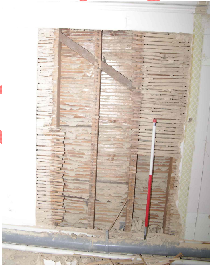
Figure 23 Plaster and laths removed on the bathroom side of the wall Looking west. 1m scale. This will be the full width of the new door
