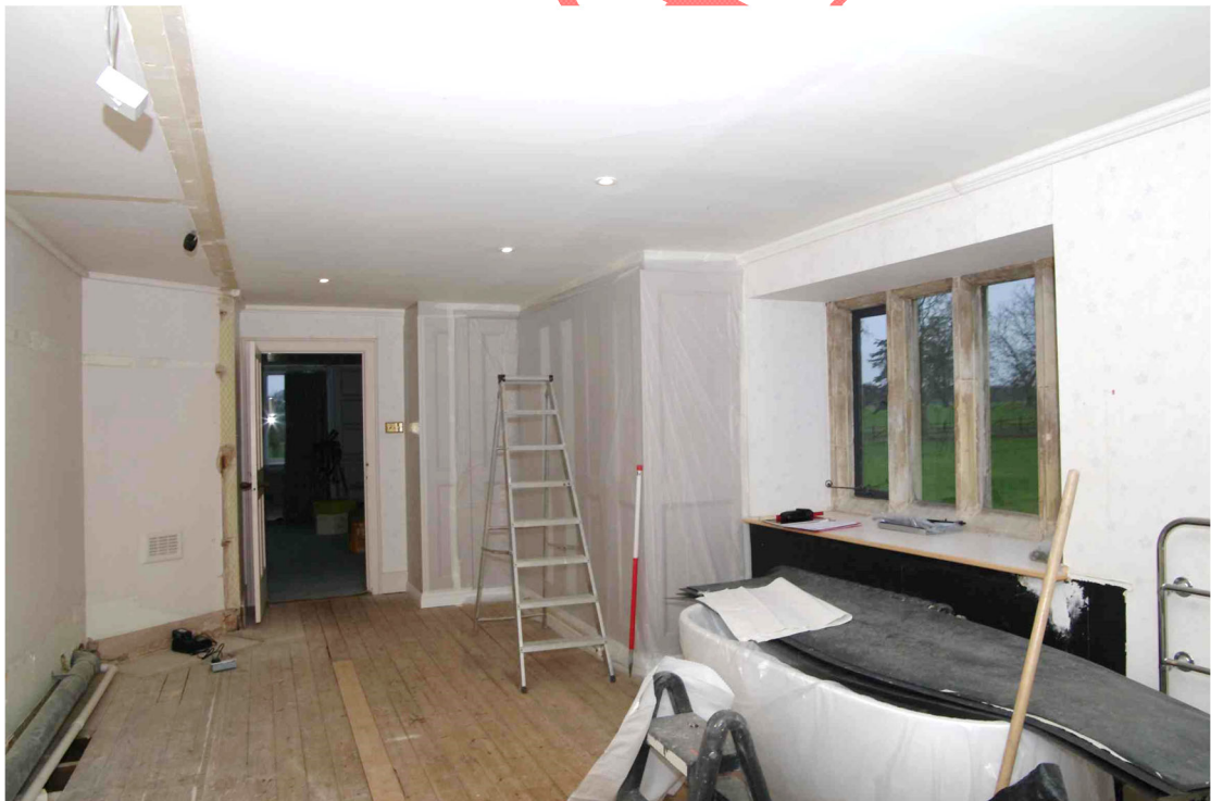
Figure 13 General view of bathroom Looking south-west. 1m scale. Note corner fireplace on left
