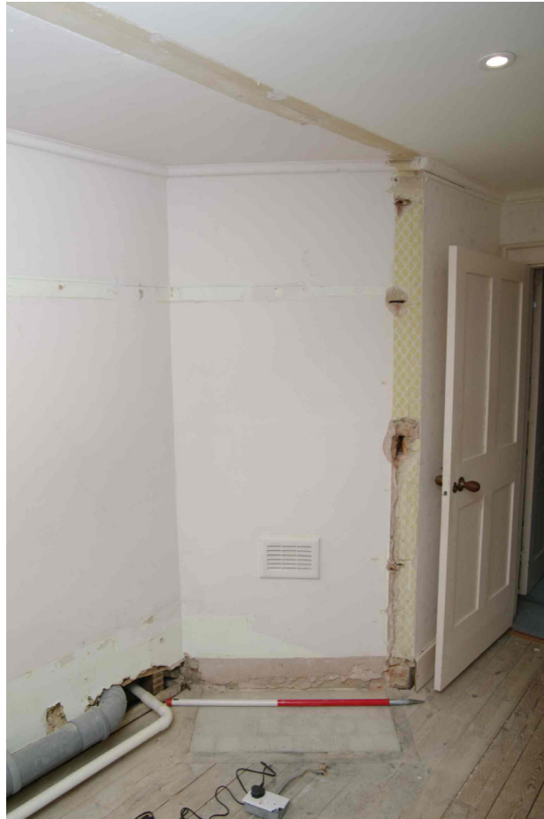
Figure 14 Blocked fireplace in the bathroom Looking south-east. 1m scale
