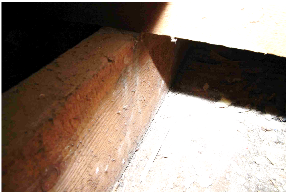
Figure 26 Transverse joist sitting on earlier floorboards in bathroom Looking through the existing bathroom floor
