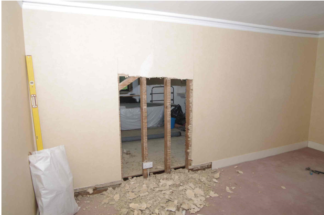
Figure 24 Plaster and laths removed from dressing room side Looking north-west. The opening is not yet up to its full 2m height in this picture
