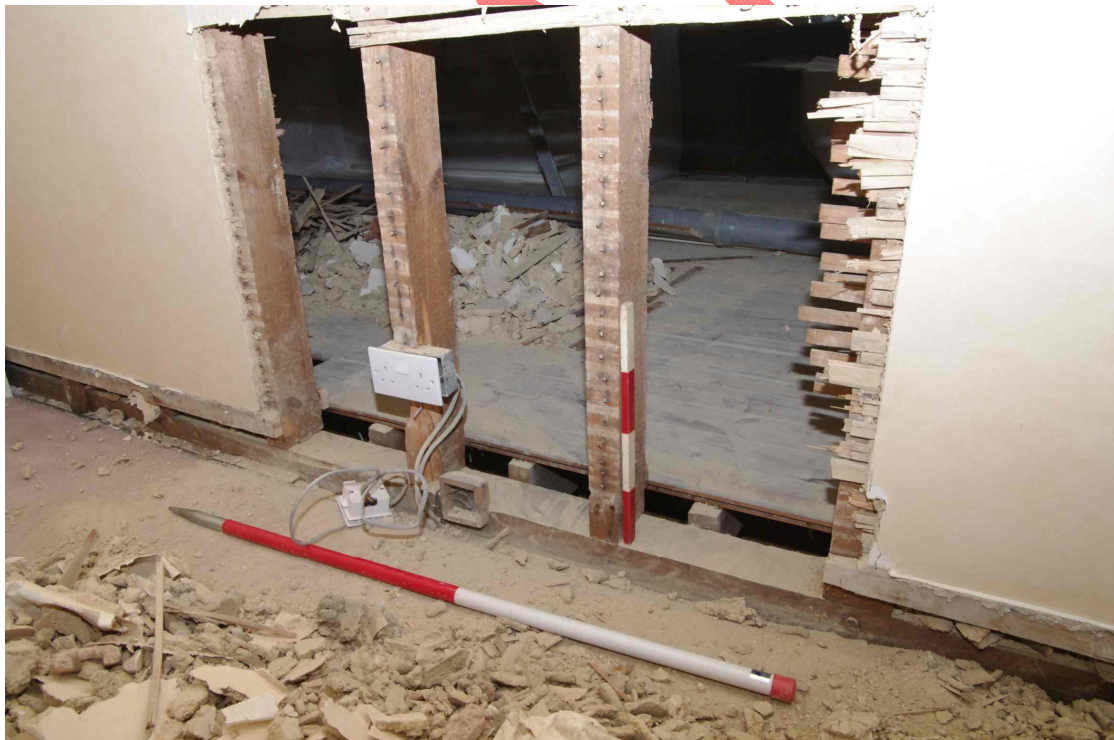
Figure 25 Difference in bathroom floor height seen from dressing room Looking south-east. 1m scale. Note the small wooden box for early electrical socket
