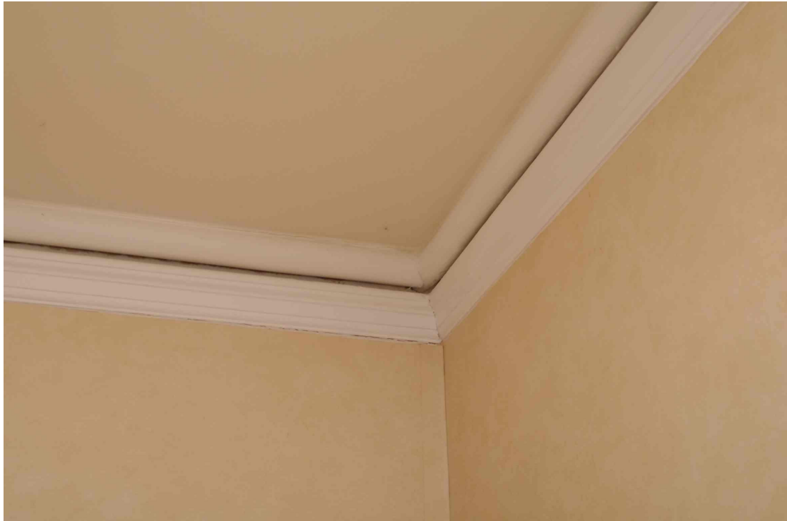
Figure 18 Beading detail in the dressing room ceiling Looking north-east. The beading on the left is a modern copy fitted to the modern stud wall
