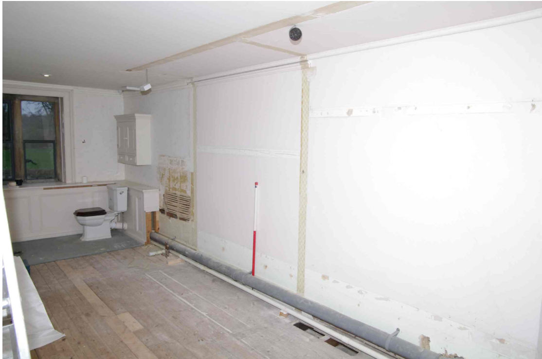
Figure 12 General view of bathroom and affected wall Looking north-east. The new doorway will be where the 1m scale is located. The mark on the ceiling shows where modern fitted cupboards were located
