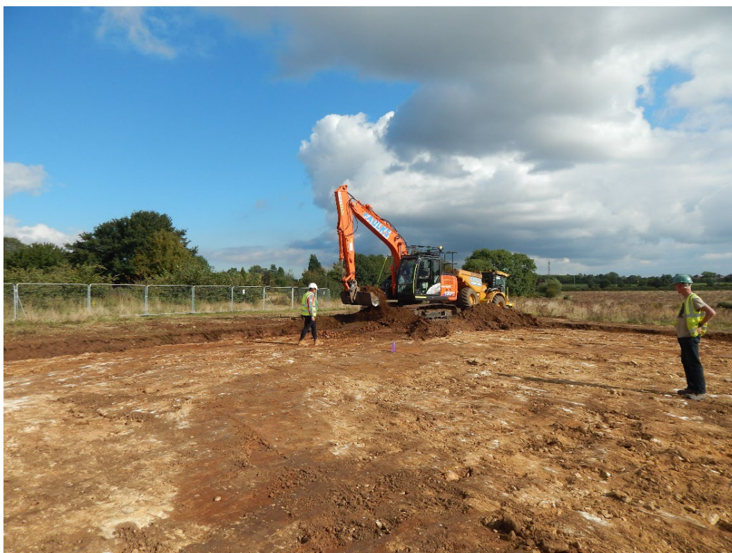
Figure 4: Photographs of topsoil stripping in progress. Above: Area A looking east; Below: Area B looking east.
