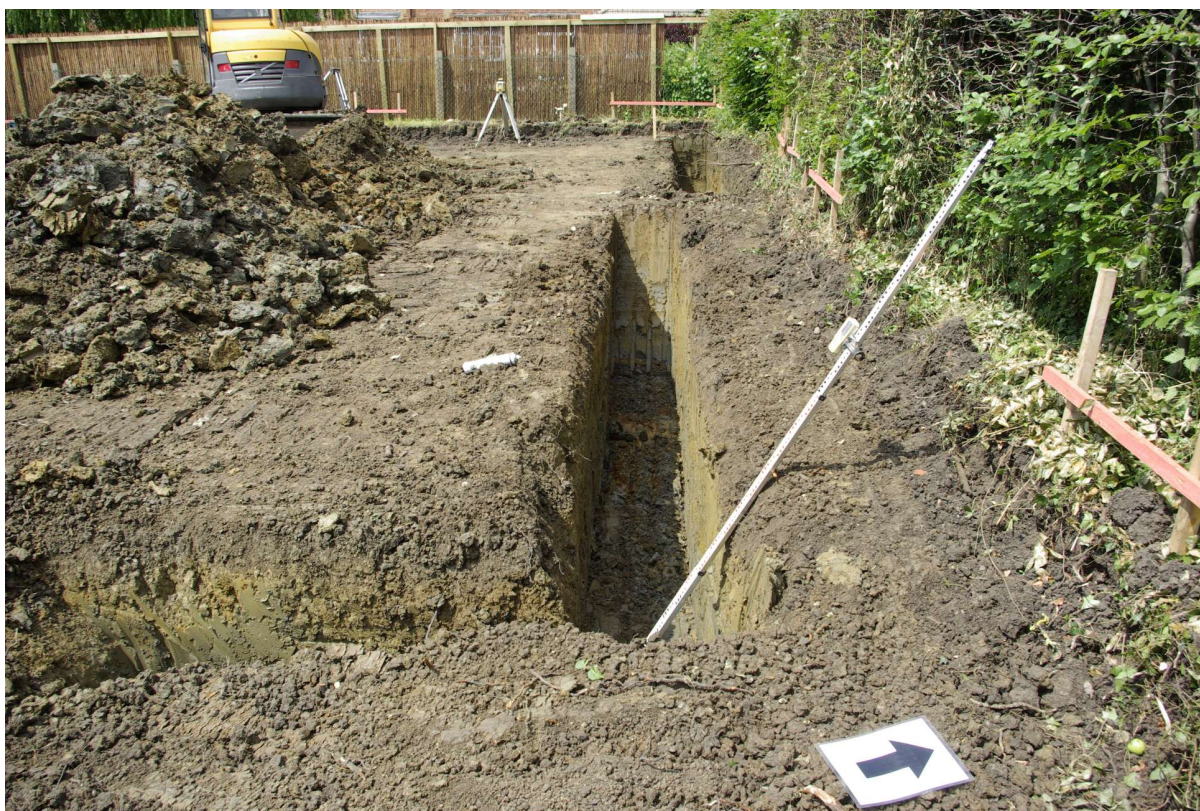
Figure 7 Foundation trenches along northern edge of development Looking west. House trench in foreground, garage beyond
