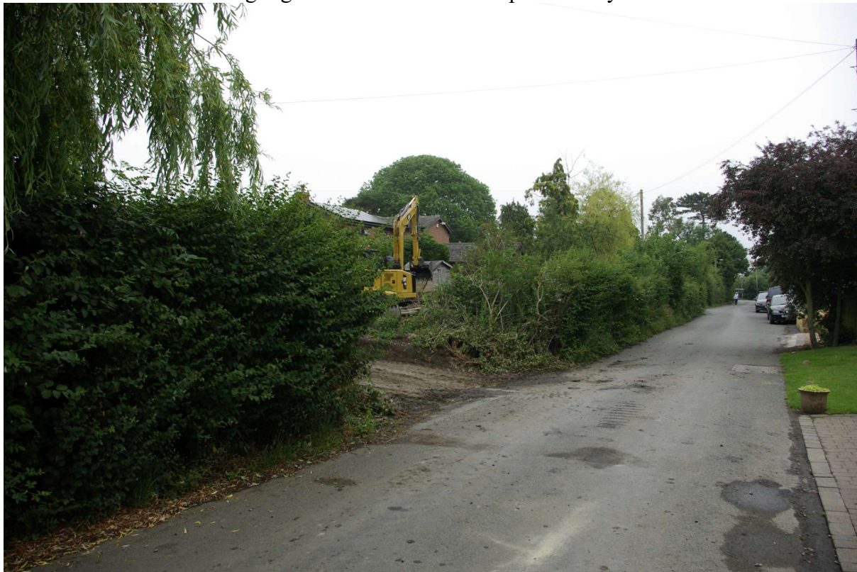
Figure 3 General view of the site Looking south-east along Dairy Lane. The hedge line on the left marks the edge of the site. Newly opened entrance on left
