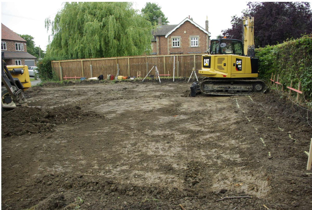
Figure 6 Northern part of site stripped down to natural Looking west. Excavator is digging the foundations for the garage. Parallel lines on right of picture show where the house foundations will be excavated
