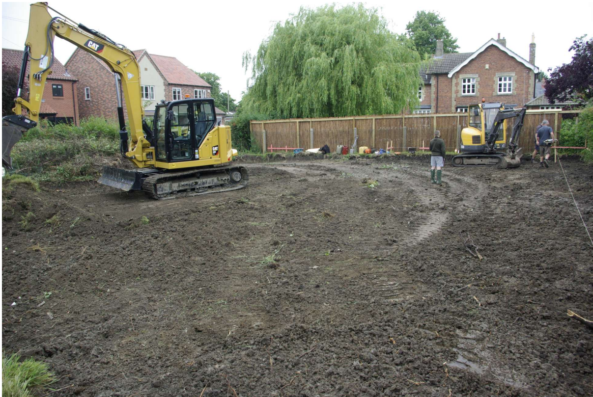
Figure 4 General view of site following turf strip Looking west. New site entrance behind excavator on left. Rutland House on right
