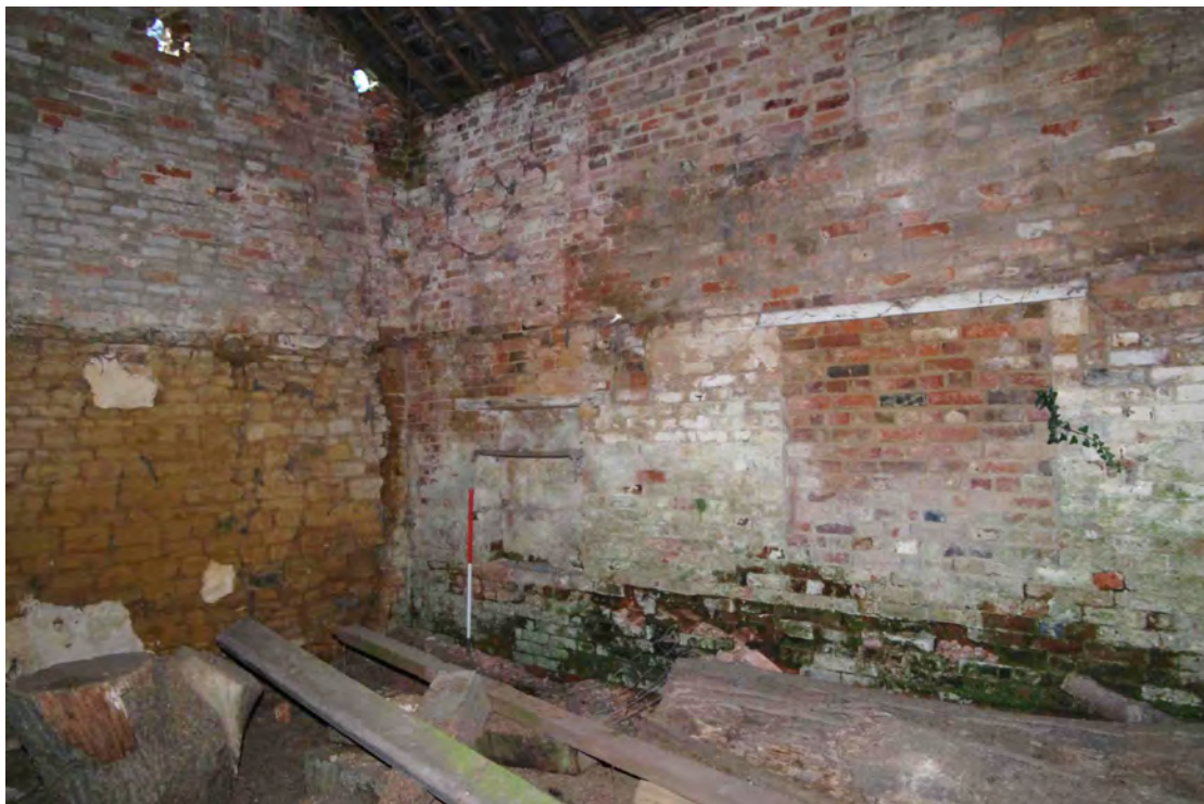
Figure 67 Building 4, general view of southern room. Looking south-west. 1m scale. Note stone base of gable wall and blocked windows
