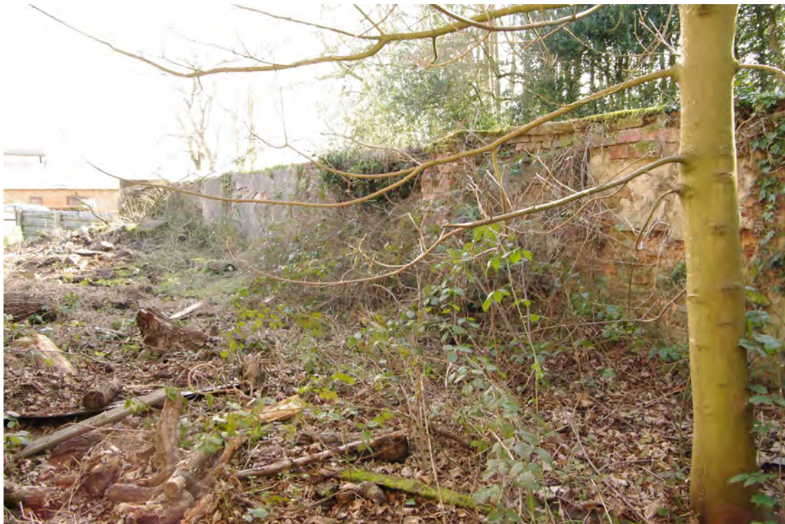
Figure 90 Inner face of boundary wall along Thornby Road Looking south-east. Note render towards the left of the shot
