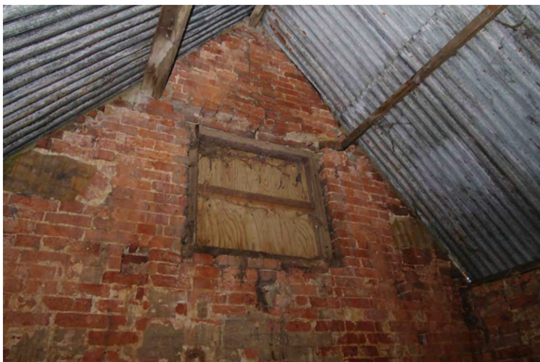
Figure 48 Building 2, hayloft door on west gable end Looking west. Note floor joist sockets in brickwork below the door
