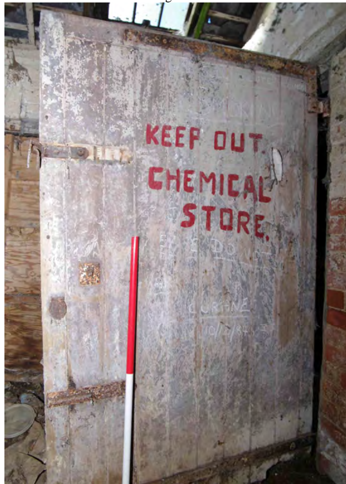
Figure 37 Building 1, door and hinge detail The door is located at the northern end of the main room. 1m scale
