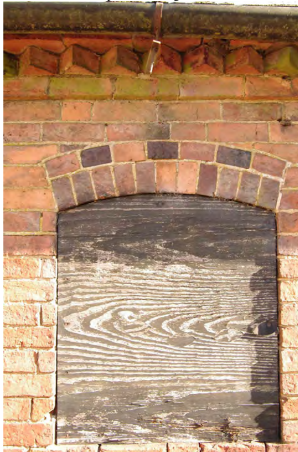
Figure 25 Barn 1, NW facing elevation window and eaves detail Looking south-west. Note the decorative use of blue bricks in the arch
