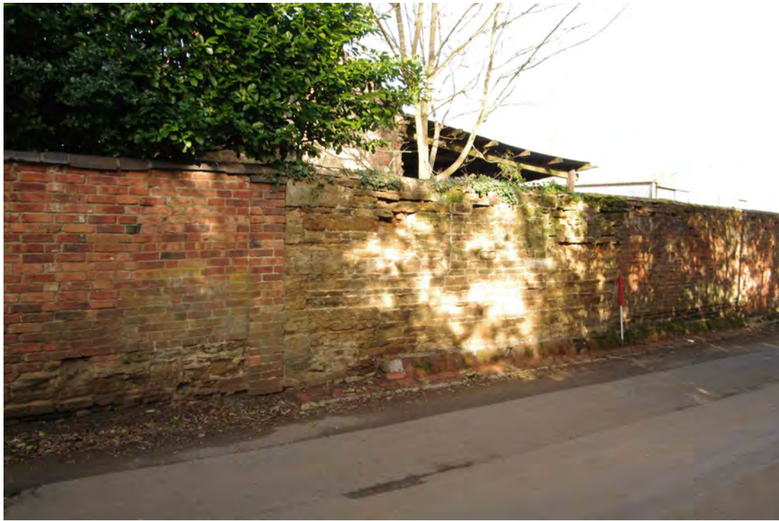
Figure 91 Boundary wall seen from Thornby Road Looking north-east. 1m scale. The brick wall on the left belongs to the adjacent Old Vicarage
