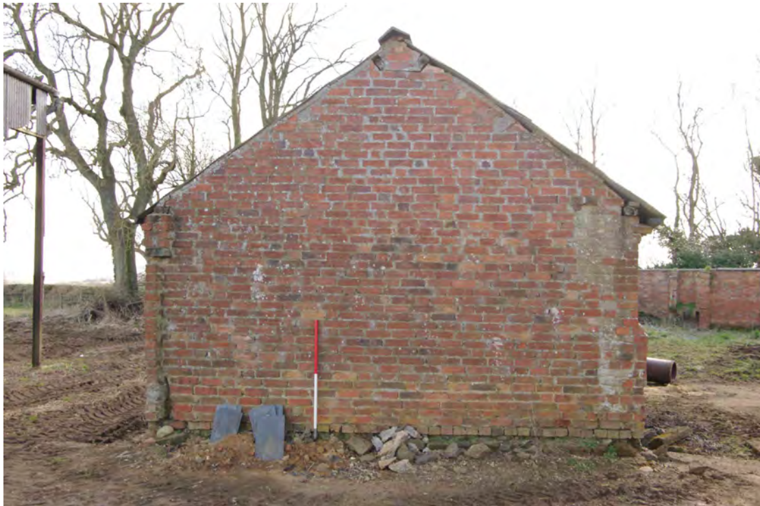
Figure 27 Building 1 north-east facing gable end Looking south-west. 1m scale. Note stub of wall on left and rebuilt corner on right from when this was attached to other buildings in the now-demolished fold yard
