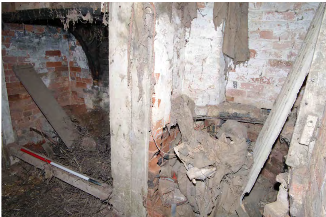
Figure 73 Building 4, remnant of former copper to east of fireplace Looking north-west. 1m scale
