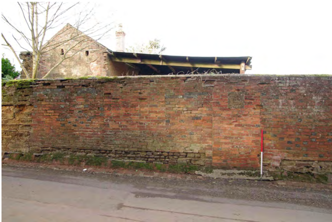
Figure 92 Boundary wall Looking north. Building 4 beyond the wall. Note how the brick portion of the wall sits on a rounded stone base. The 1m scale stands in front of a blocked doorway with an inserted date stone (see next figure)
