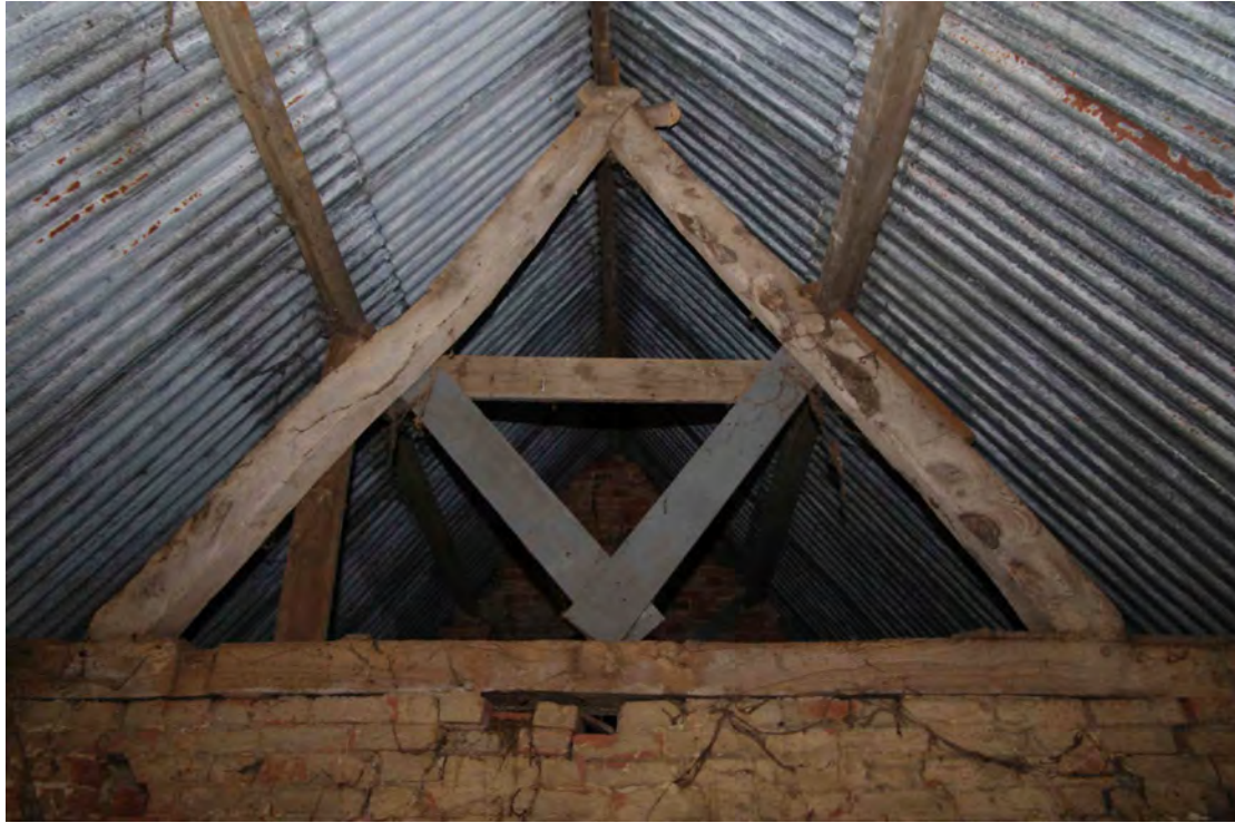
Figure 49 Building 2, roof structure Looking east. The plank bracing in the centre of the structure is modern
