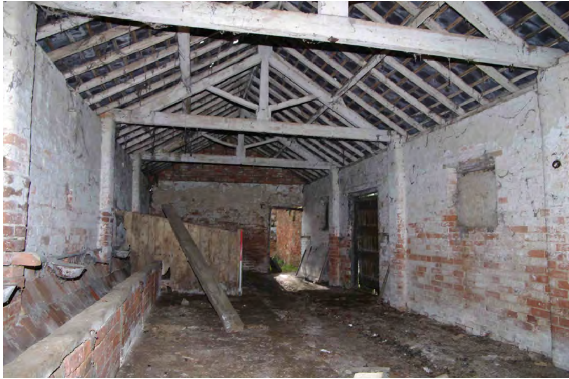
Figure 34 Building 1, general internal view Looking south-west. 1m scale. Note flat lintels to doors and windows compared with the arches seen outside
