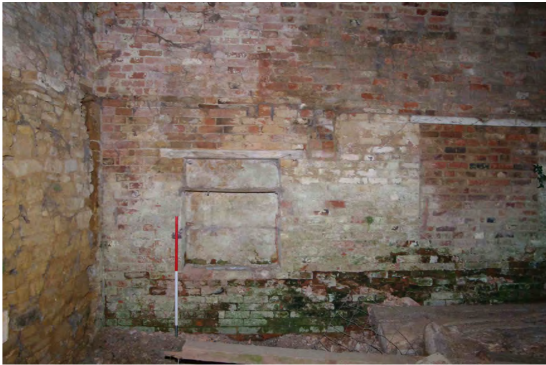
Figure 74 Building 4, blocked windows on west wall. Looking west. 1m scale. Note blocked windows indicated by lintels
