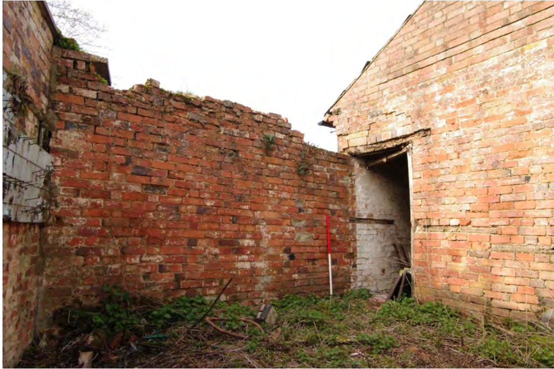
Figure 32 Building 1, south-west facing gable end Looking north from within open-roofed area. 1m scale
