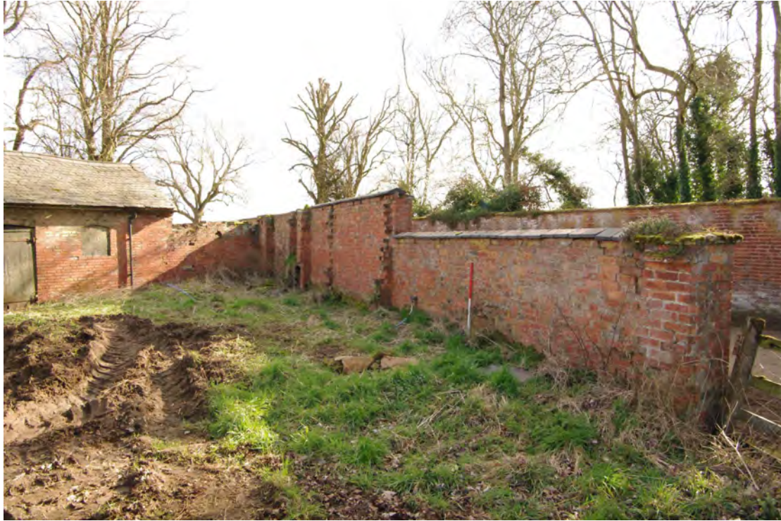
Figure 95 Eastern arm of the boundary wall Looking south-east. 1m scale. Building 1 on left
