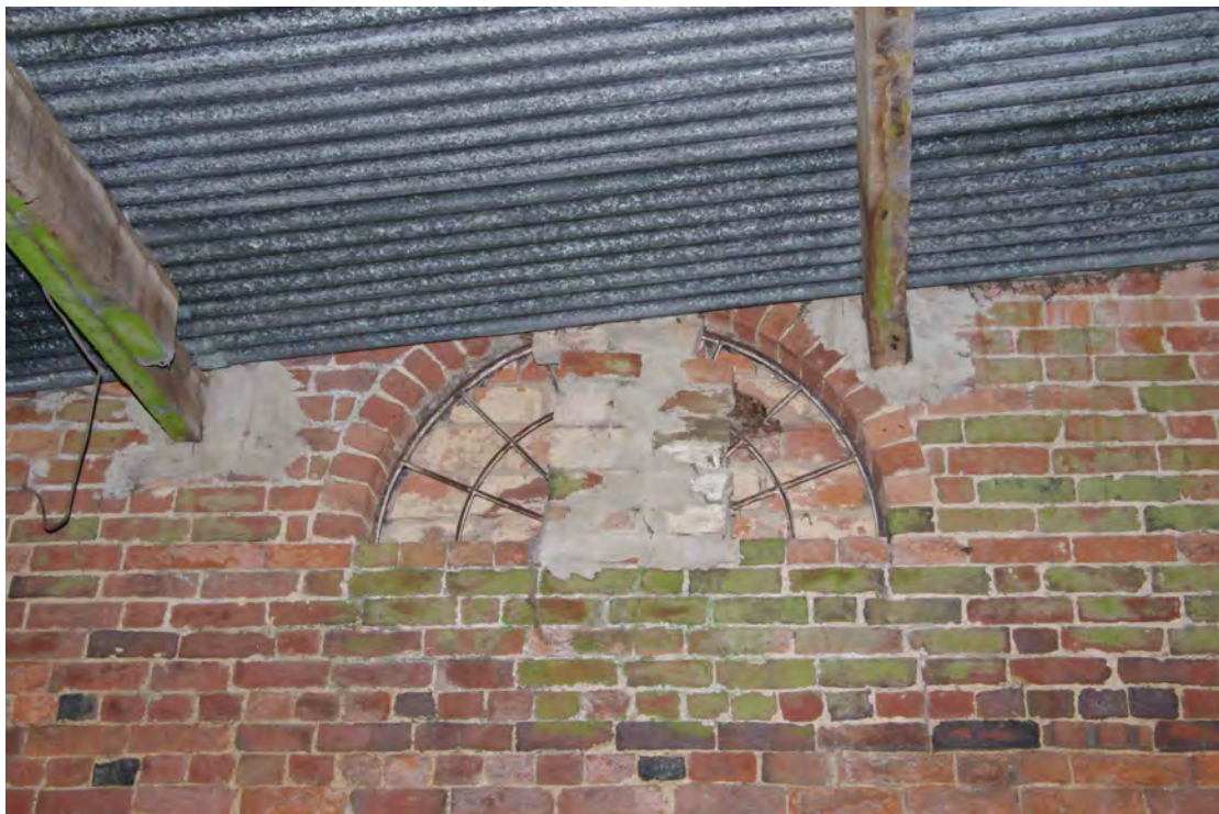
Figure 87 Building 4, blocked window on south side of north end bay Looking south. This is the other side of the window shown in Figure 84
