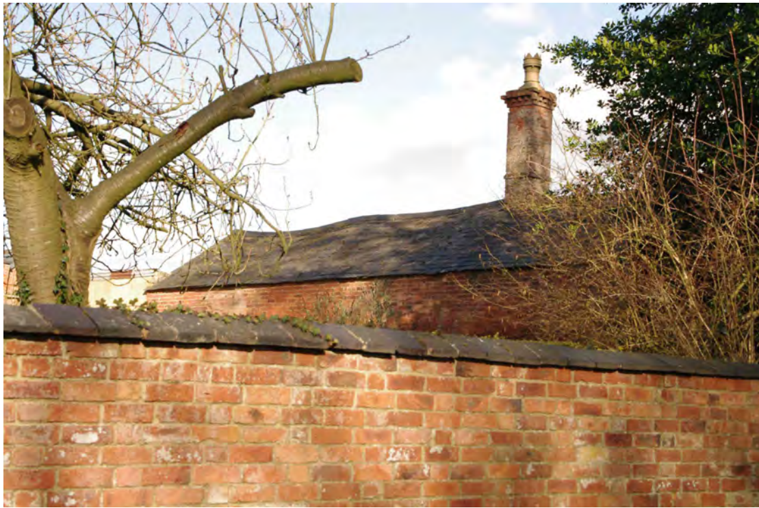
Figure 66 Building 4, west side of roof Looking north-west over Vicarage wall from Thornby Road
