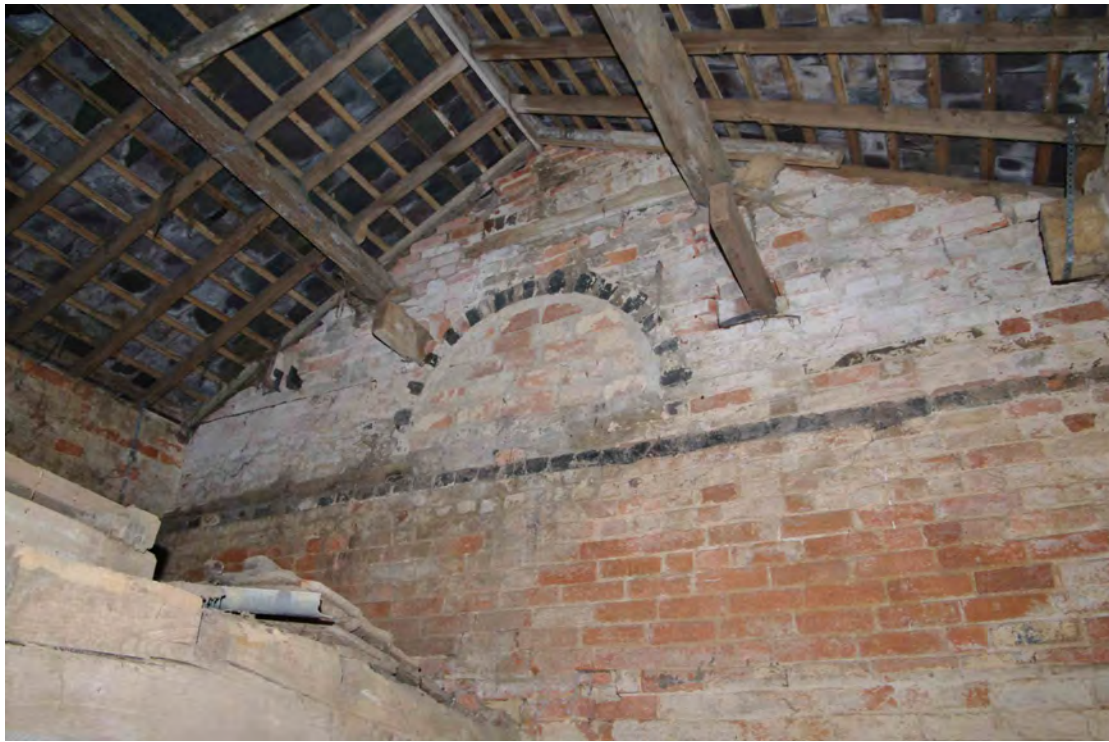
Figure 84 Building 4, north room, blocked window on north wall. See Figure 87 for opposite face. Looking north-west
