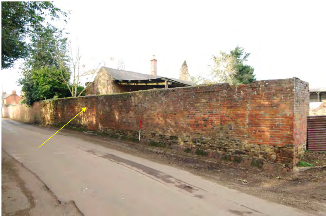
Figure 94 Full extent of western arm of the boundary wall Looking north-west. 1m scale. The arrow points to the date stone
