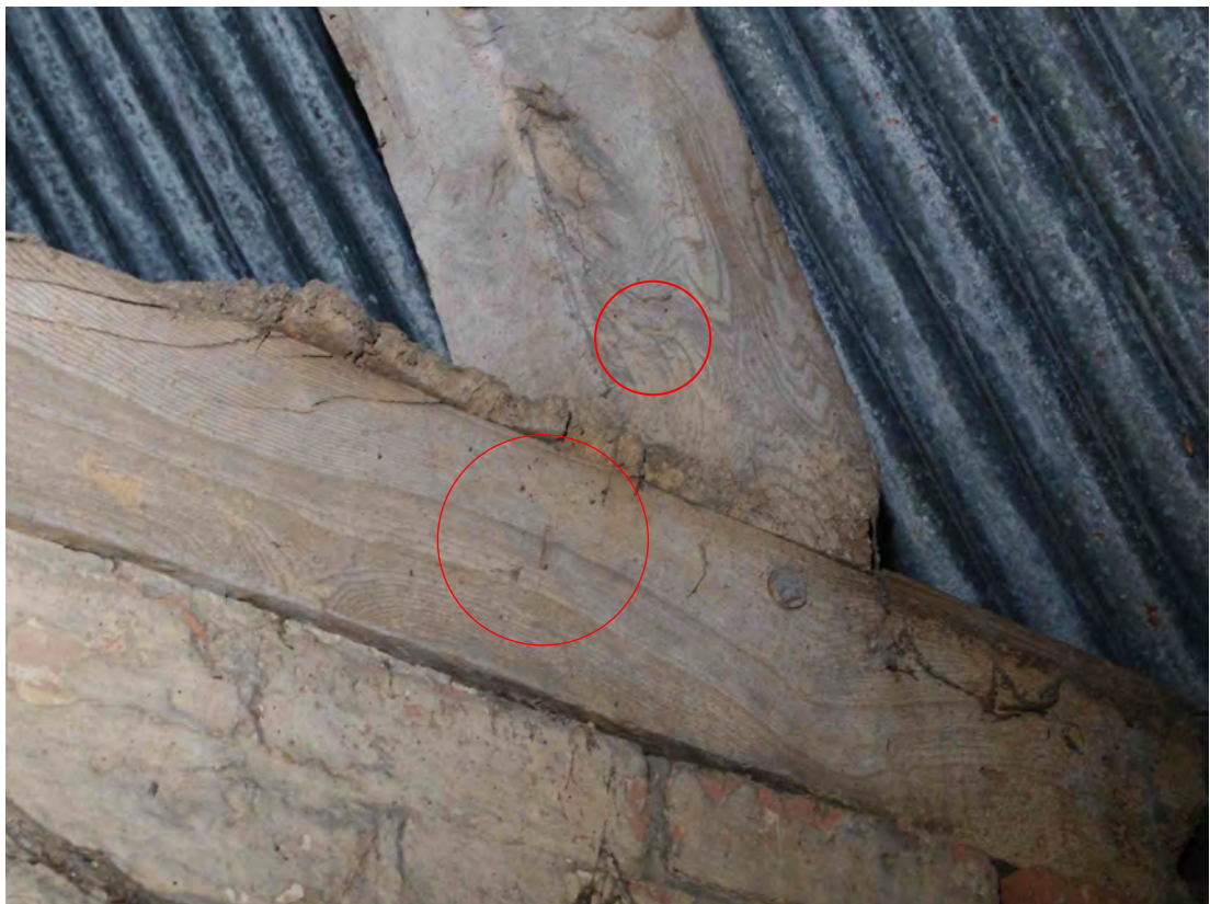
Figure 51 (Both photographs) Building 2, construction marks on roof structure The marks are on the west facing side of the timbers
