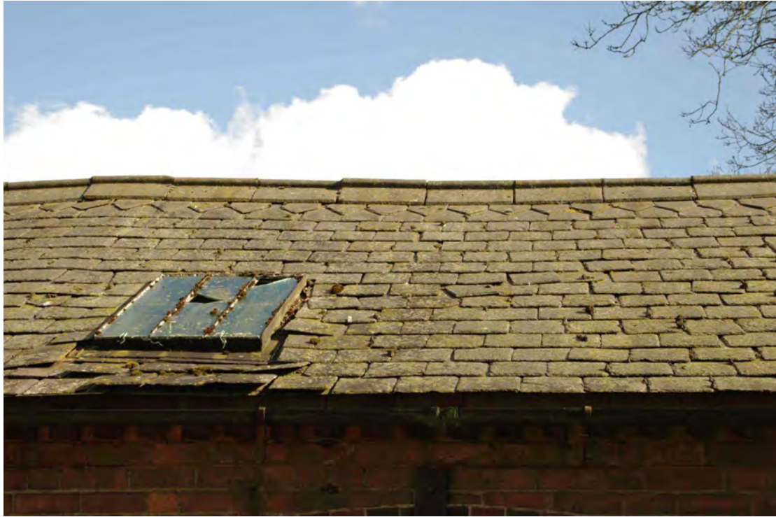
Figure 26 Building 1 decorative ridge detail and iron-framed skylight North-west facing roof shown but details same on both sides
