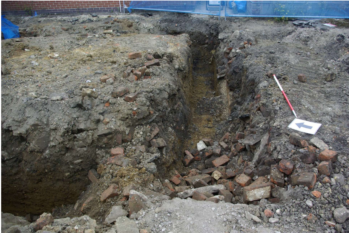
Figure 20 Plot 6 foundation trench, NE corner Looking north-east. Note drain pipe running along right hand side of trench
