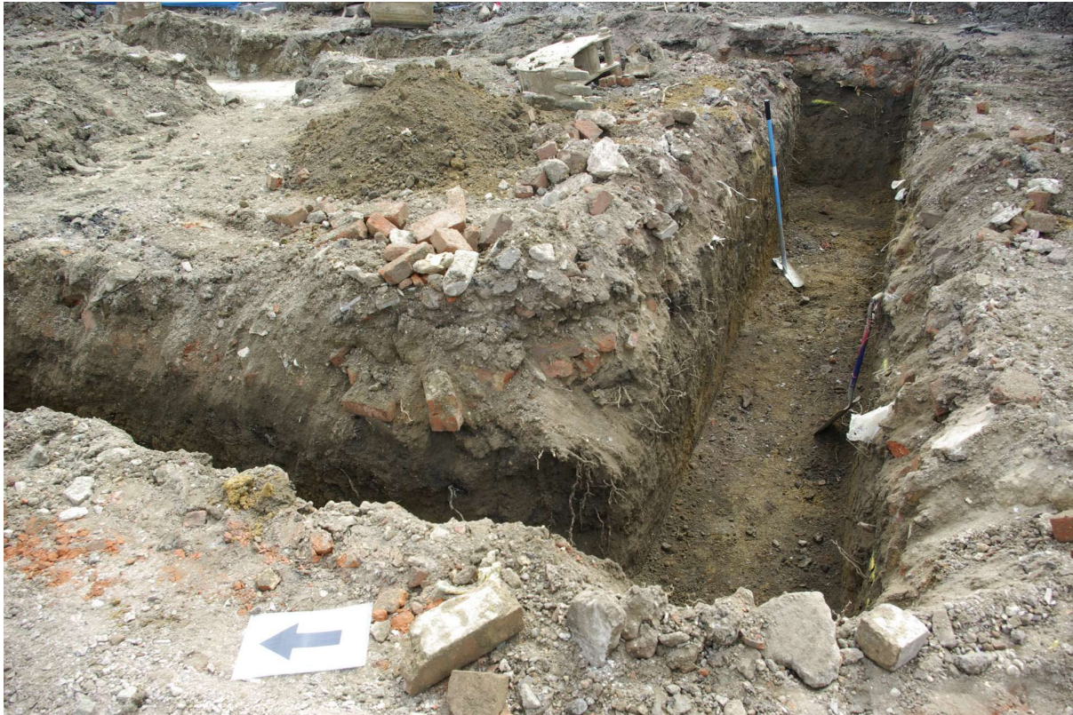
Figure 22 Plot 2 foundation trench Looking east. Note the presence of subsoil in this trench. Plot 1 is yet to be excavated on the right of the picture
