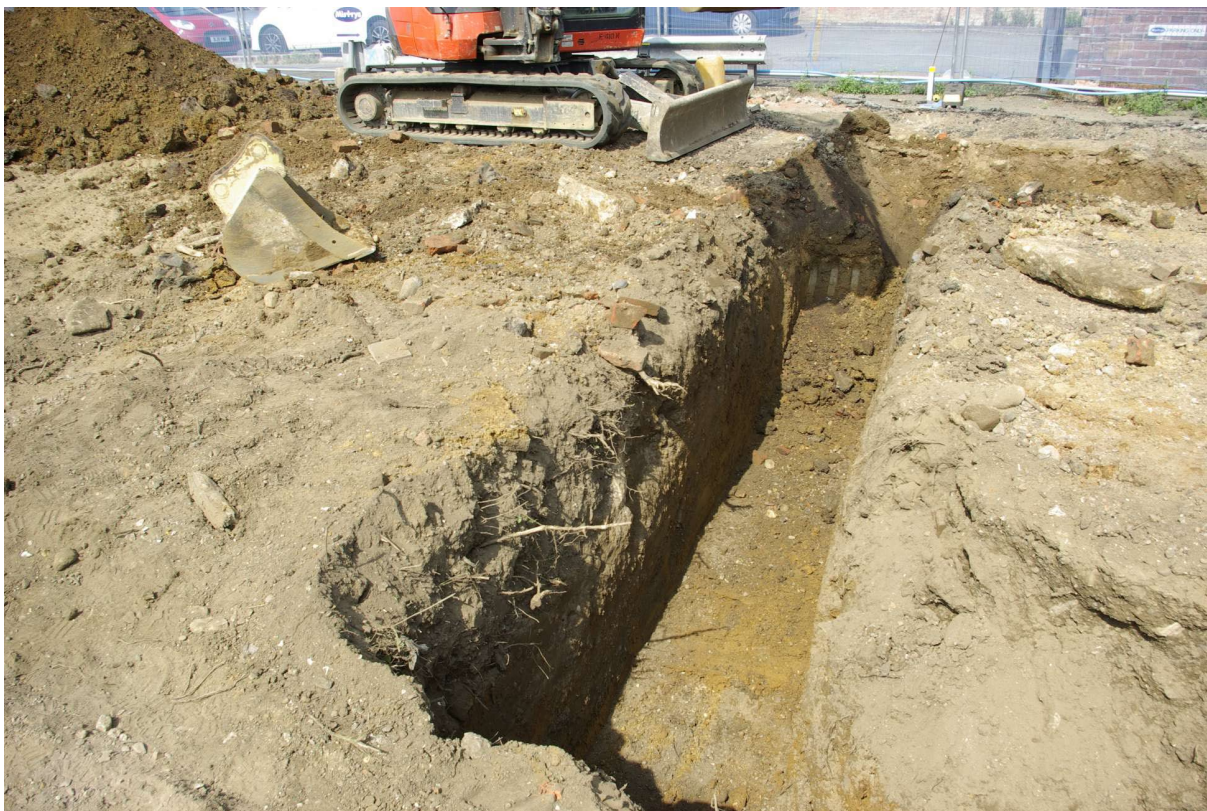
Figure 21 Foundation wall between Plots 4 and 5 Looking north-west. The base of wall (10) is just beyond the lip of the trench in the foreground
