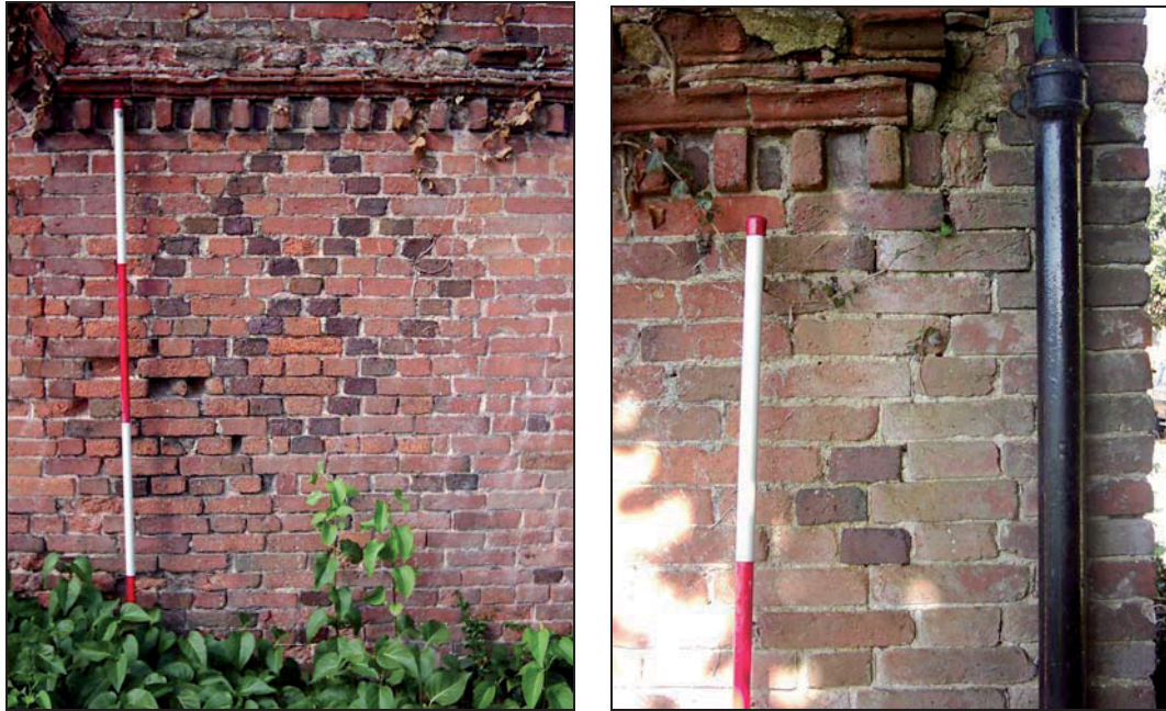
Figure 7 & 8: Diaper on south elevation and truncated diaper and stringcourse.
