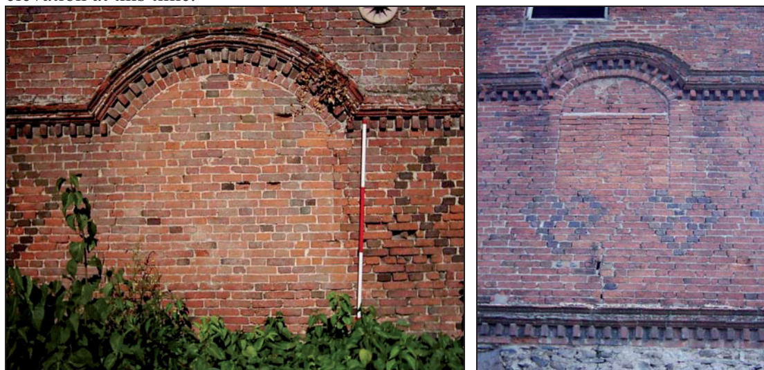
Figures 5 & 6: Blocked windows on the south and west elevations.
