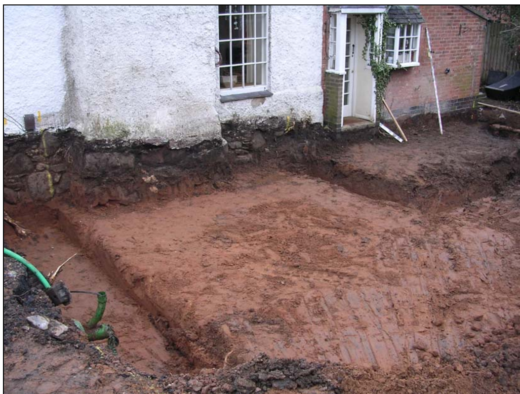
Figure 3: General view of development area, looking south-east, showing exposed footings. The pit was located within the footings on the right of the picture.
