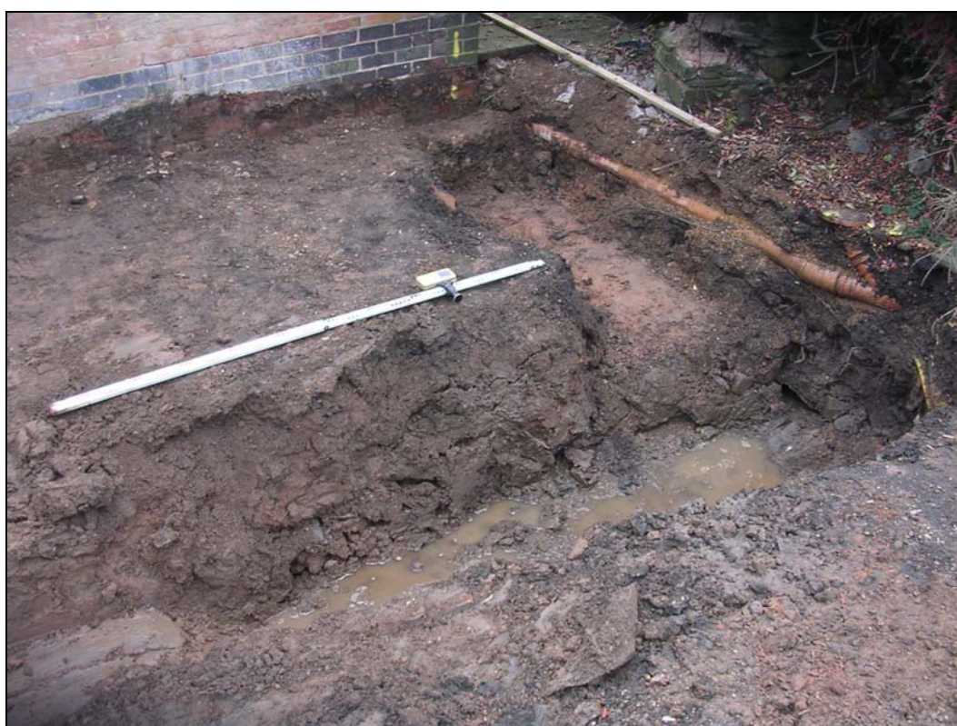
Figure 4: Footing through large rubble filled pit exposed within southern half of the development, looking south-east.
