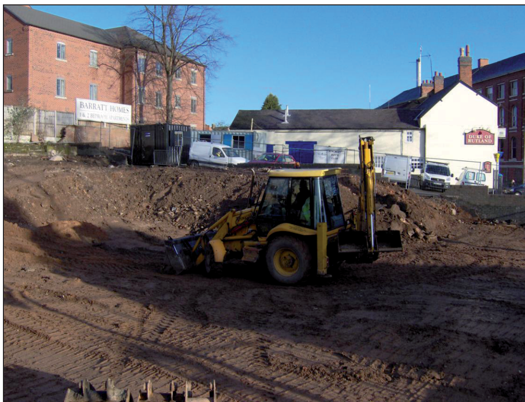
Figure 4. Area to be reduced. Duke of Rutland pub shown in Fig. 3 in rear of picture.
