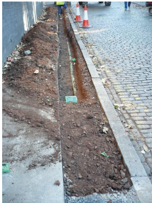
Figure 7; Welles Street view east along west pavement at Bath Lane junction end following groundwork
