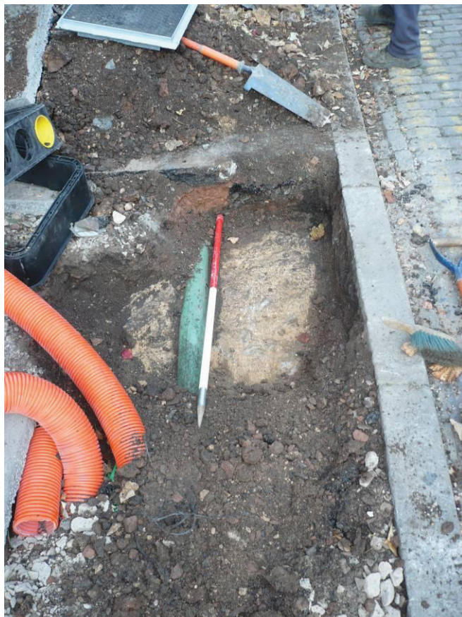
Figure 8: view east of deposit under CCTV access hatch
