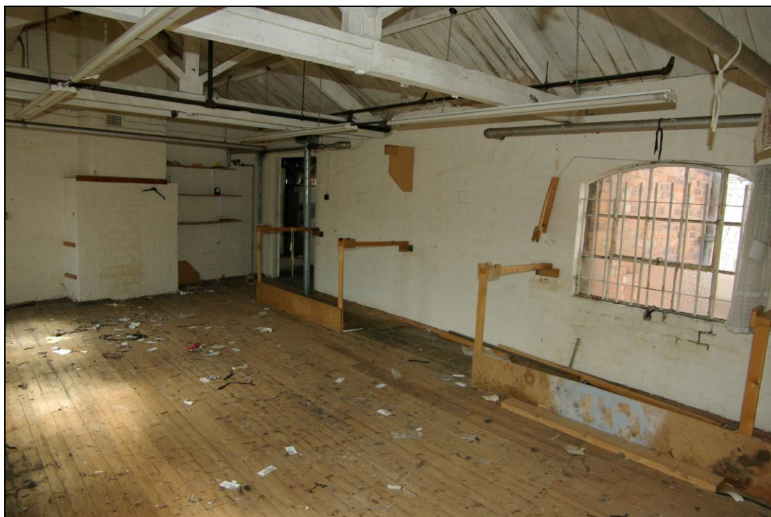
Figure 17. Main building, first floor. Blocked windows on rear wall and inserted doorway. Looking south-west.
