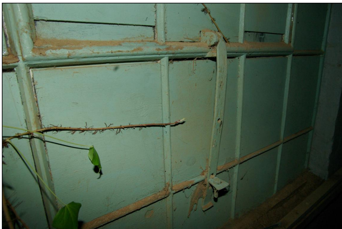
Figure 15. Main building. Window latch detail.
