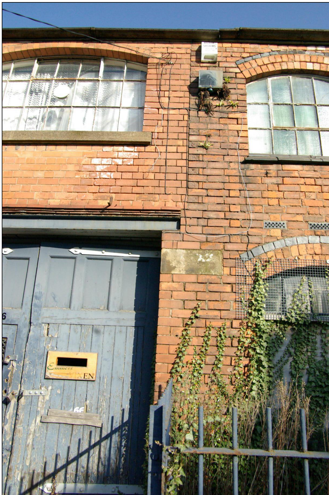
Figure 9. Laban Tansey Building. Joint between phases on frontage. Looking west.
