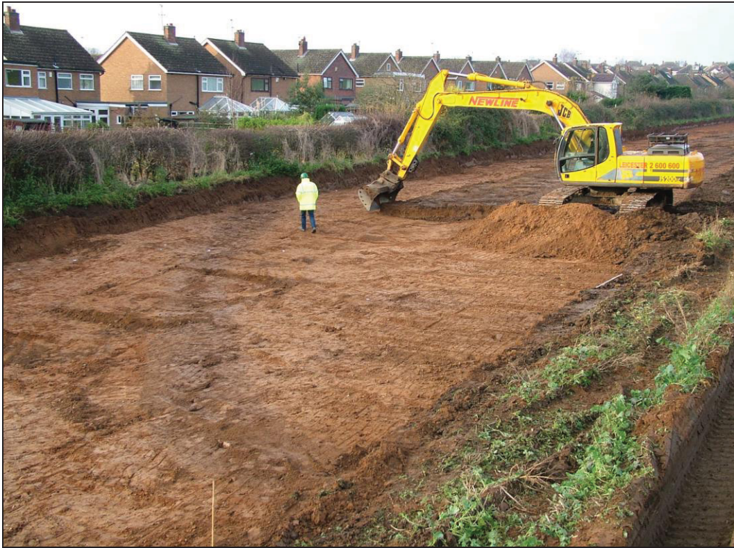
Figure 7: View showing the topsoil removal by machine looking south-west. The south-east corner of Enclosure I is visible in the centre-foreground,
