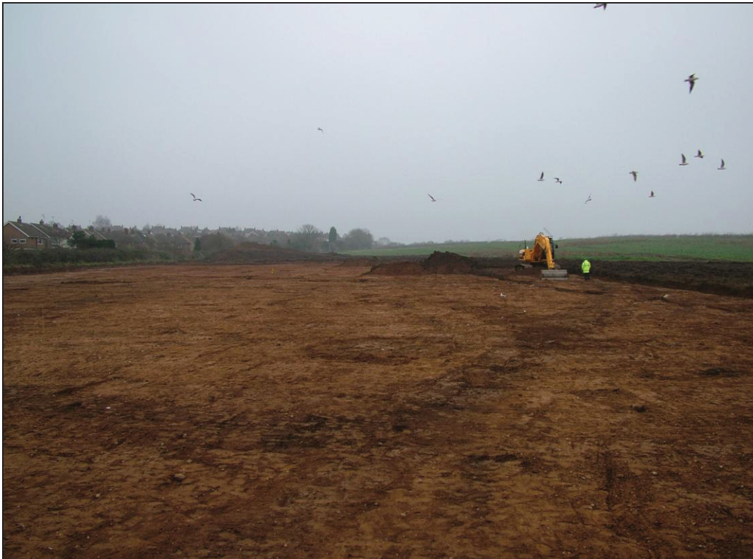
Figure 8: View showing topsoil removal by machine looking west. The north-east corner of Enclosure I ditch is visible in the foreground.
