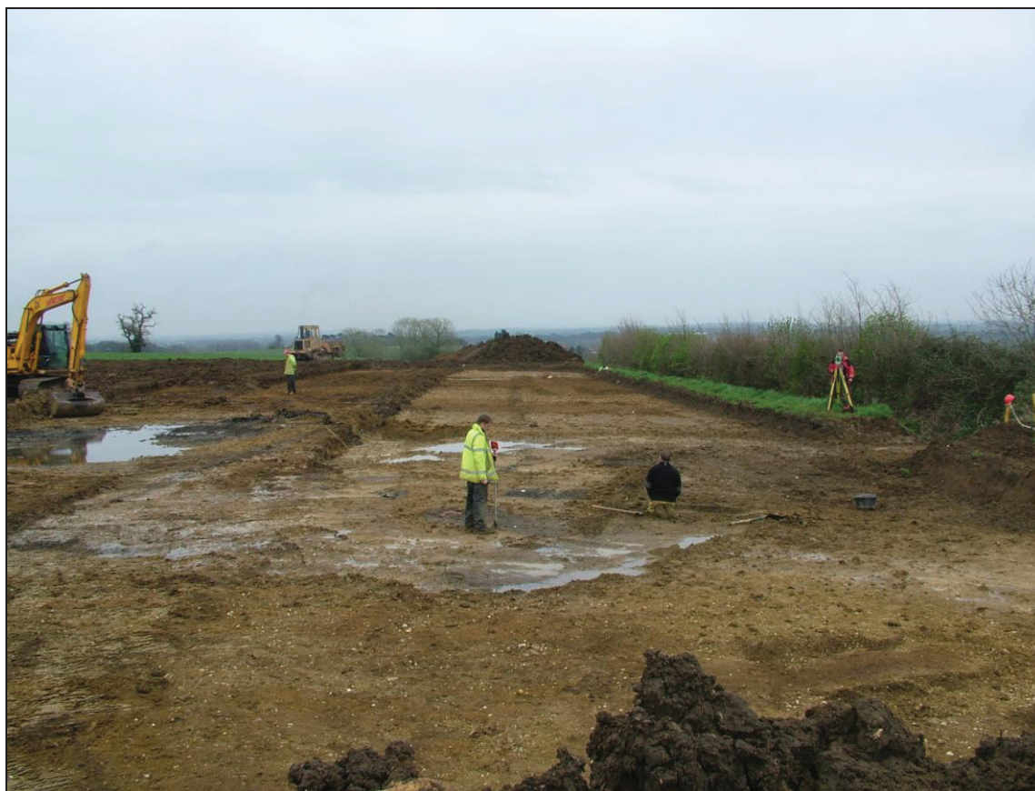
Figure 51: Area 3, general working view looking east with excavation, recording, and further machining in progress. The waterlogged conditions are evident from the standing water in the centre of the photo.
