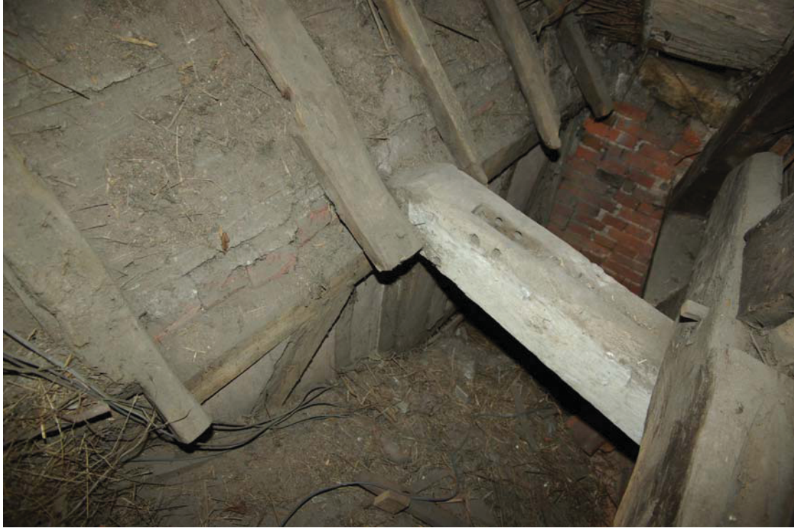
Plate 9. As above, viewed within roof space, with continuation of side wall-frame and rafters above service end bay of box-framed building, interrupted by inserted stair. Looking east.
