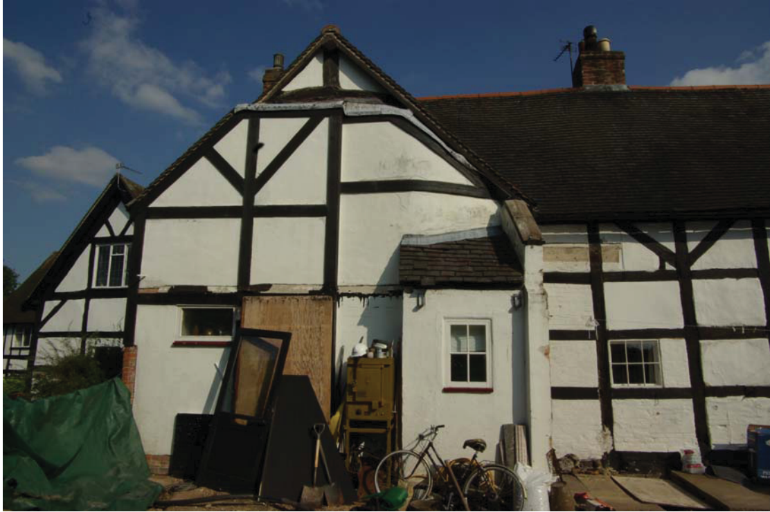
Plate 3. Modern gable end wall, with top of cruck frame visible above, and box-frame structure to right. Looking east.
