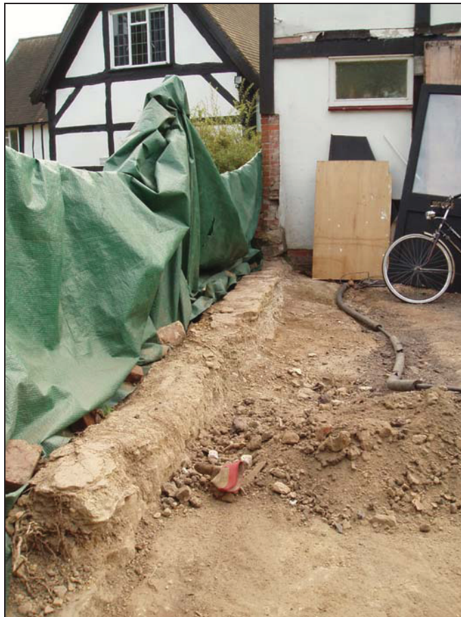
Plate 25. Northern limit of excavation, with 'shelf' of natural sandstone. Looking east towards modern gable end wall, to cruck-truss cross-wing stub.
