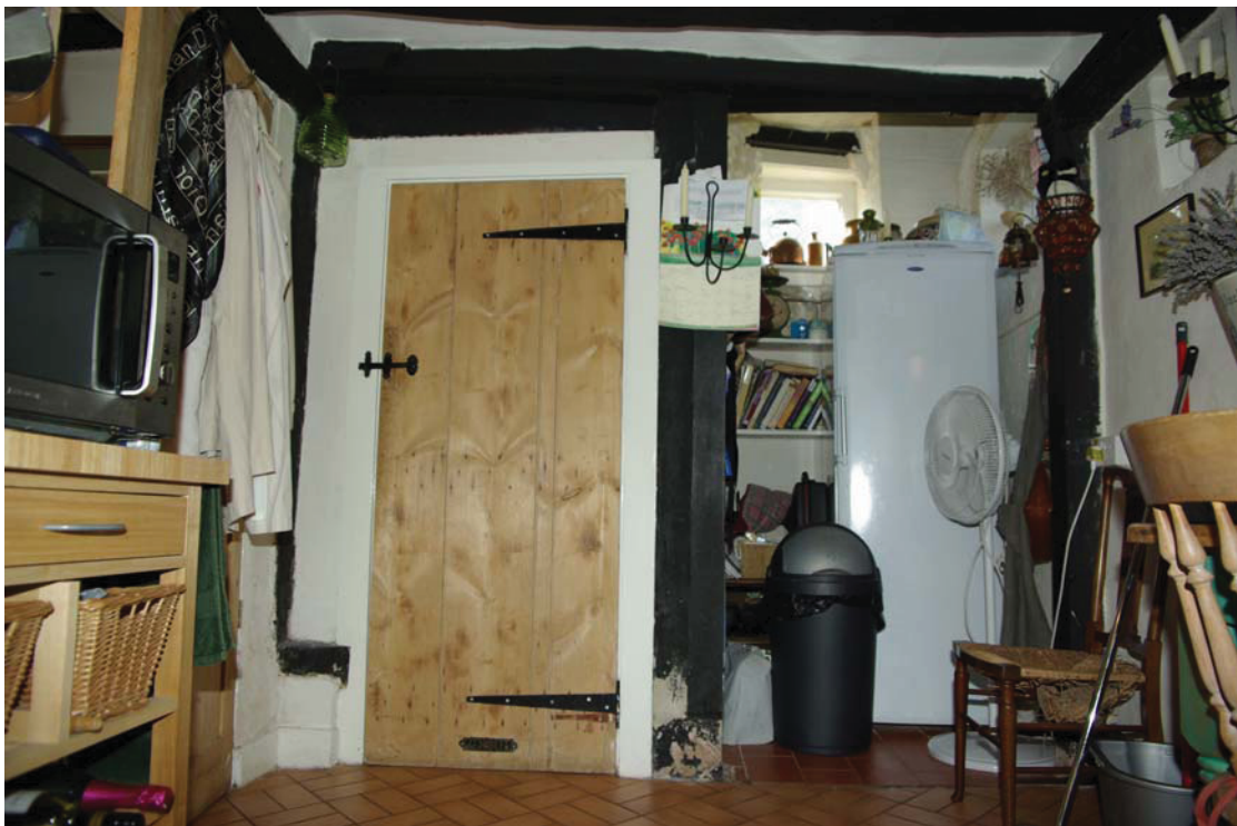
Plate 12. Wall-posts and girding beam within service end bay, showing continuation of box-framed structure. Looking west.
