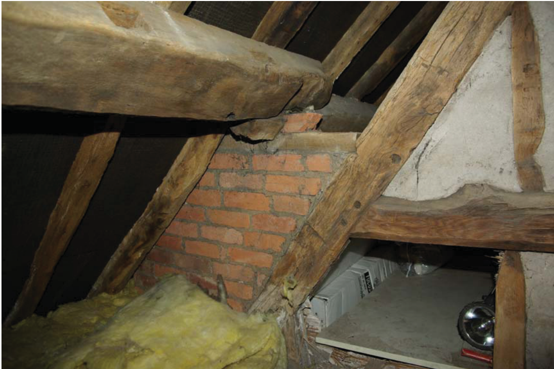
Plate 17. 18 th century modifications to raise height of eaves to frontage façade of box-framed structure. Looking southeast.
