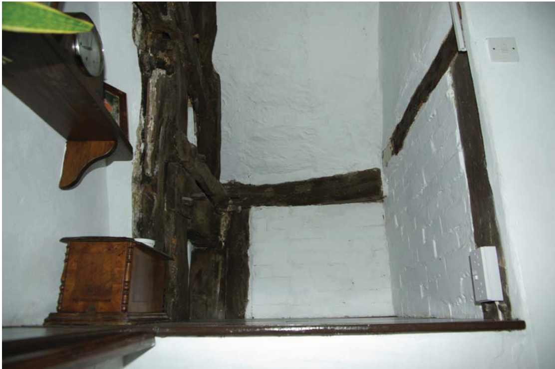
Plate 8. Linking section between box-framed structure, to right and cruck truss, to left. Looking north.
