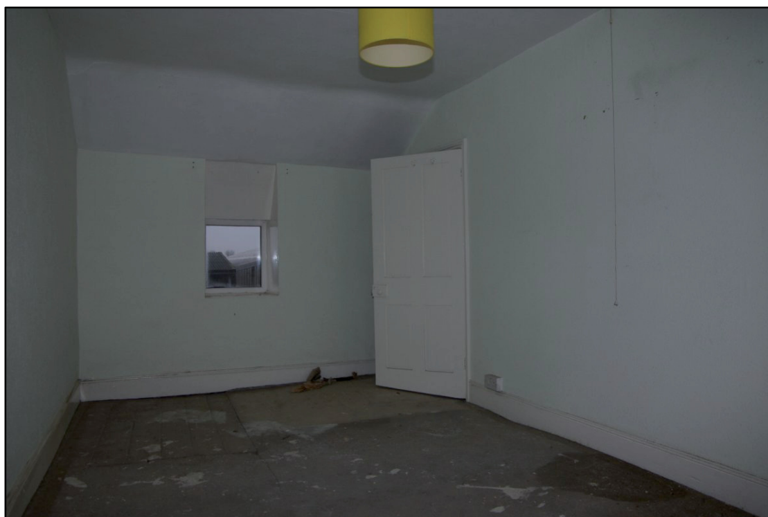
Figure 27 First floor, eastern room. Boarded hole in corner. Facing south west.
