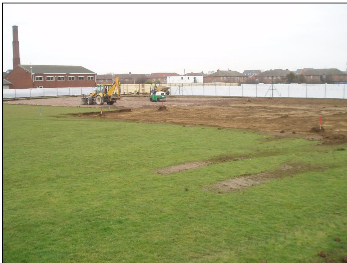
Figure 4. Area after stripping. Facing north east Existing school on left of picture. Stone pile mat being laid.
