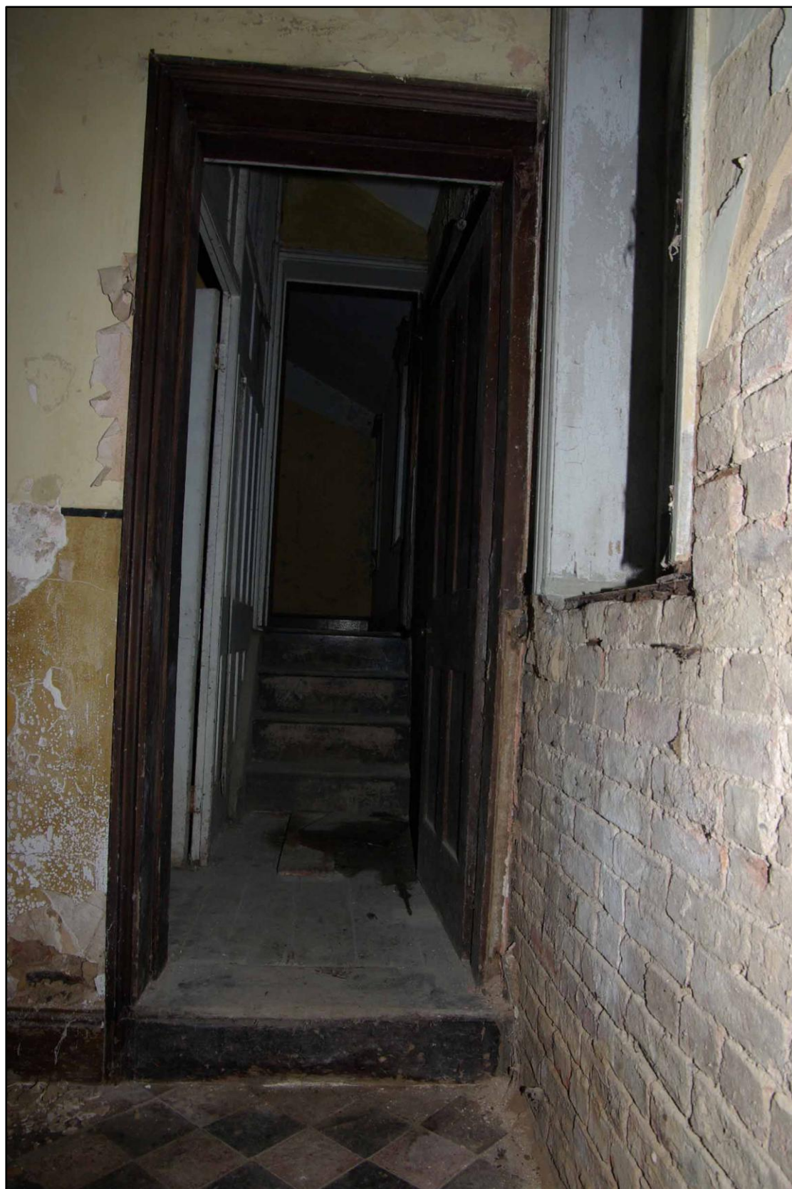
Figure 15. View from room four through room five and stairs to room six. Looking west.
