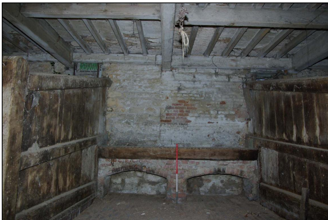
Figure 64 North west to south east stables, trough and blocked entrance Looking north east. 1m scale
