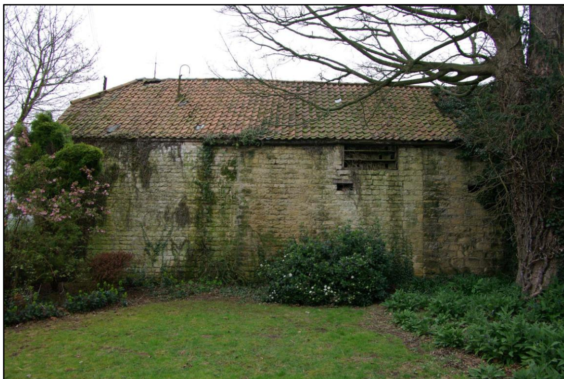
Figure 61 North west to south east stables, north east elevation Looking south west
