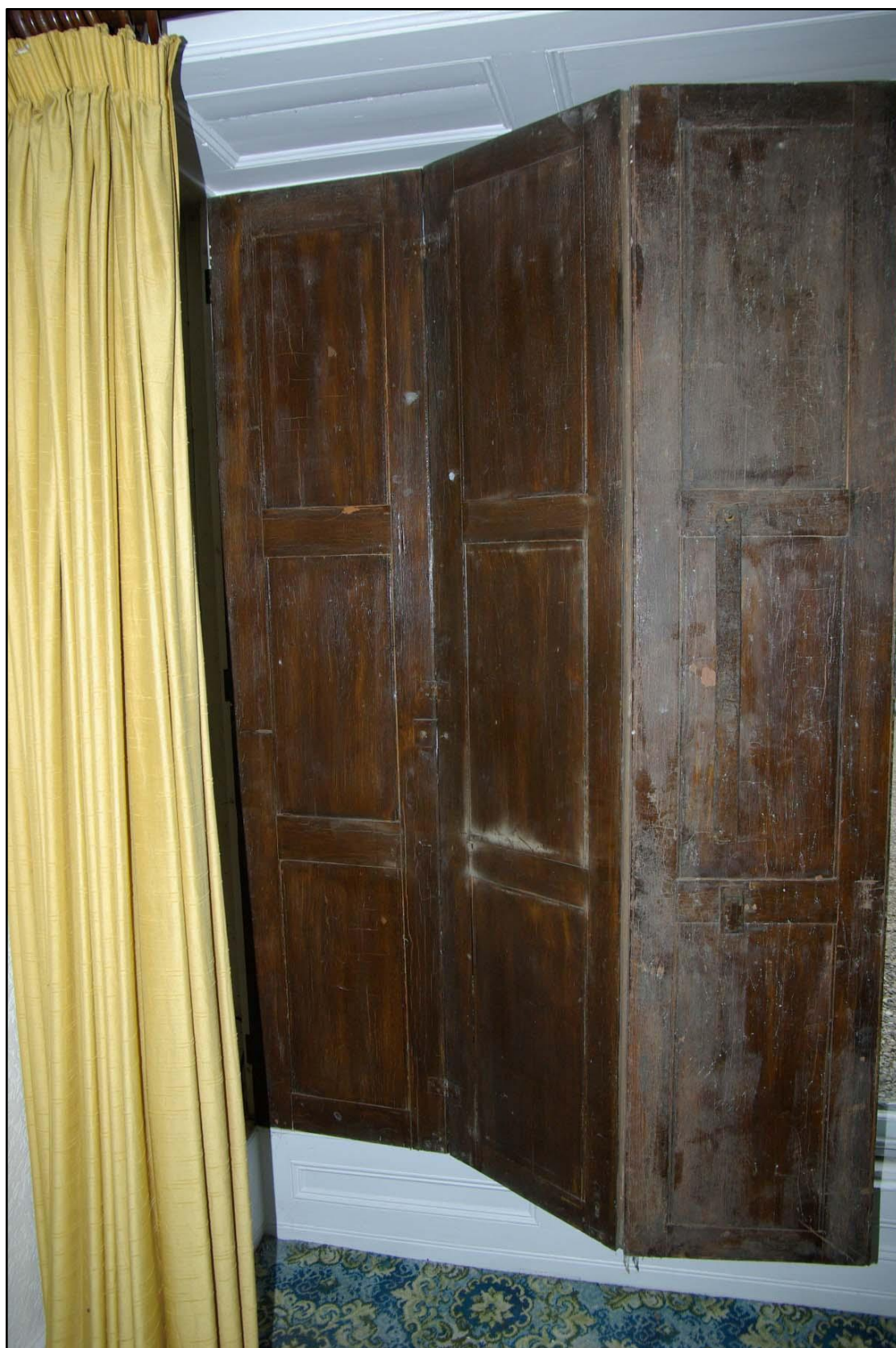
Figure 19 Front window shutters, eastern room Looking south east
