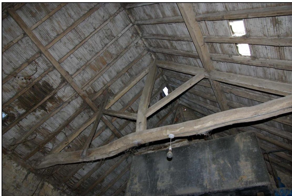
Figure 62 North west to south east stables, roof structure at southern end Looking south east
