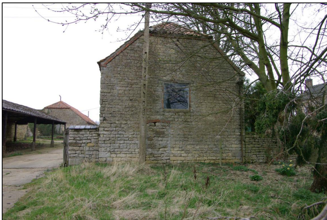
Figure 60 North west to south east stables, southern gable end Looking north west
