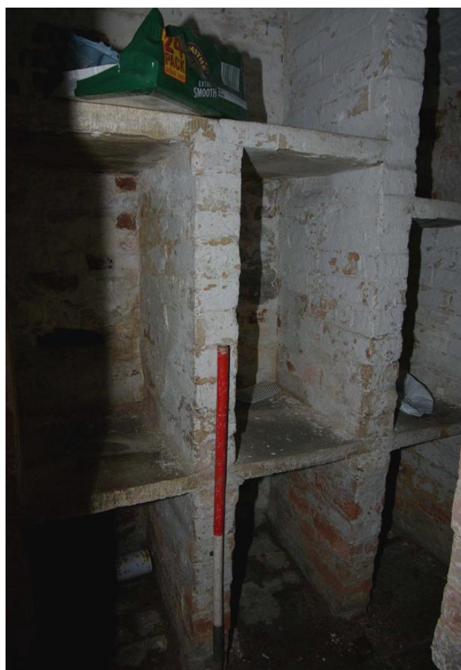
Figure 25 Racks in cellar Looking south. 1m scale
