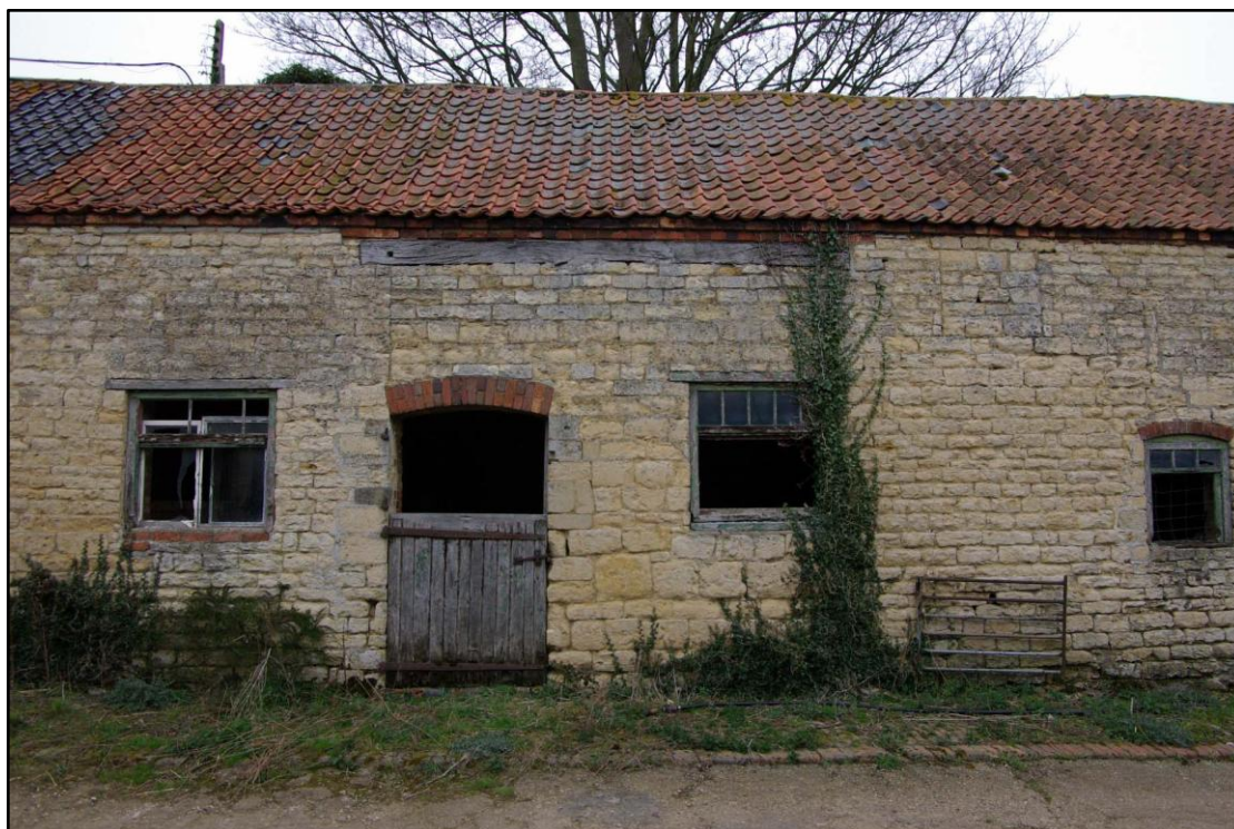
Figure 59 North west to south east stables, blocked barn door Looking north east. Ivy on right hides joint
