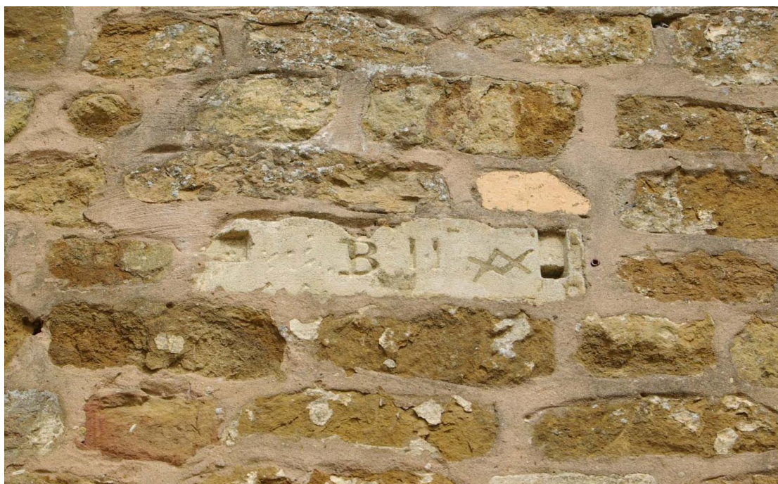
Figure 16 Graffiti on south-east elevation
