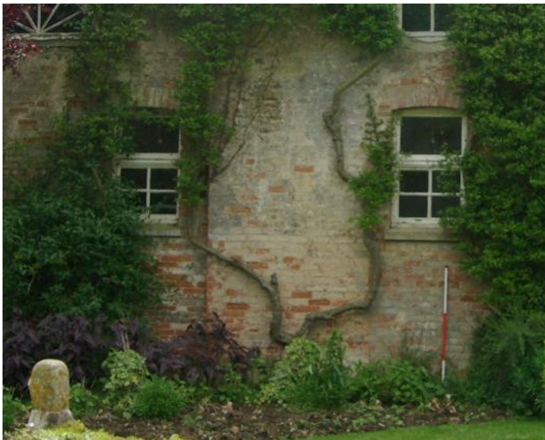
Figure 11 Blocked opening beneath ground floor gable window 1.5m scale
