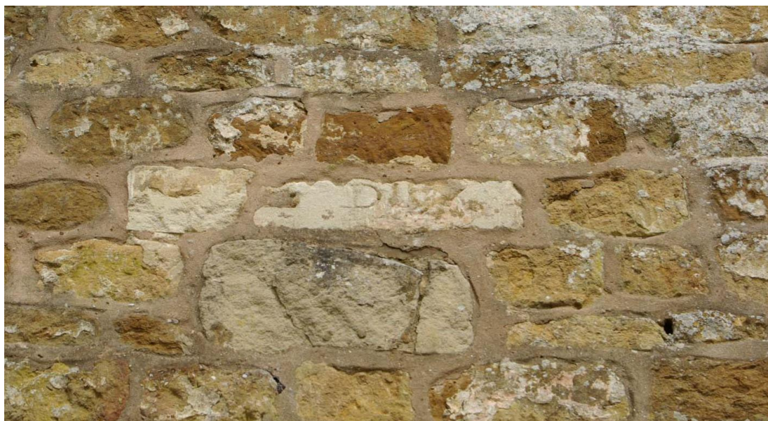
Figure 17 Graffiti on south-east elevation
