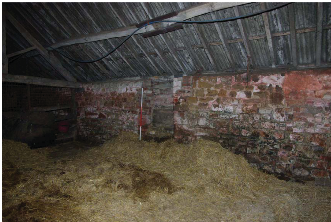
Figure 27 Barn A blocked doorway and missing roof truss Looking north. 1.5m scale.
