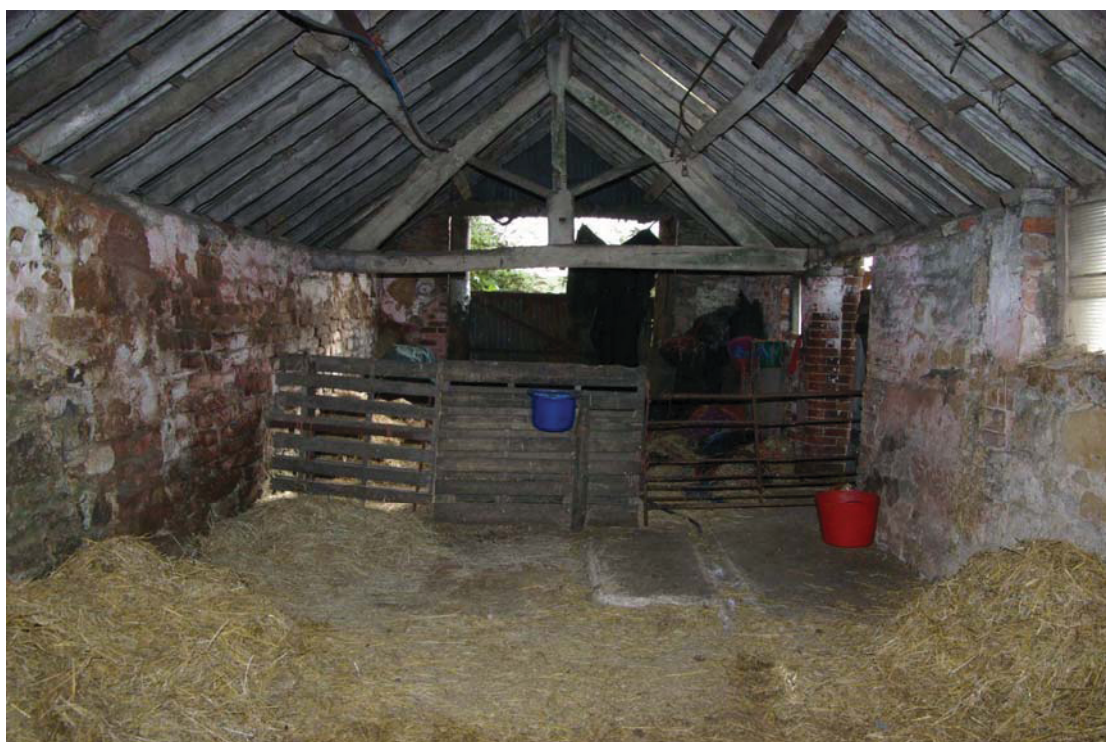
Figure 29 Barn A fourth and fifth bays and missing roof truss Looking south-east.
