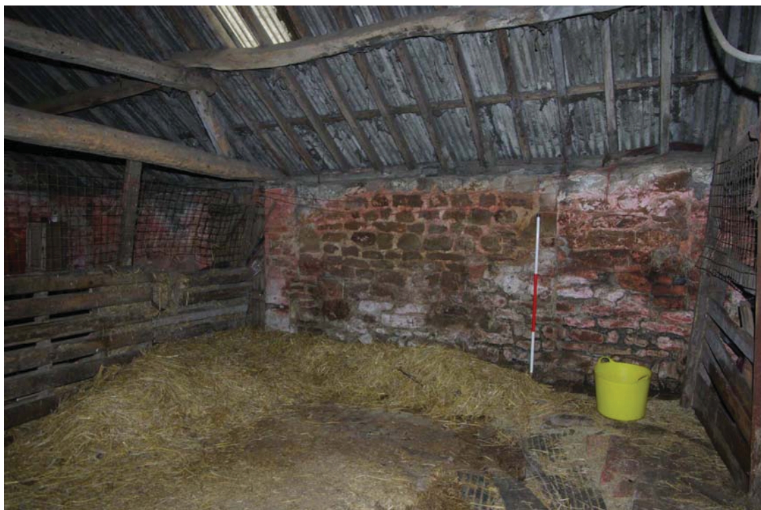
Figure 25 Barn A second bay and straight line joint Looking north-east. 1.5m scale.
