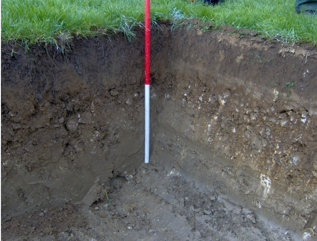
Figure 3: Turbine trench – a typical section showing the basic stratigraphic sequence of topsoil, natural gravel and natural clay. Looking west.
